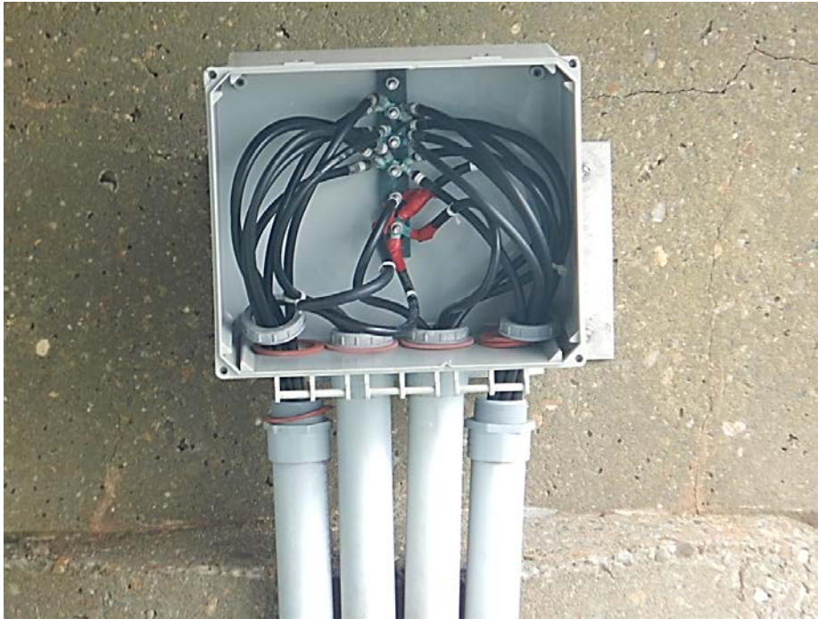
Photo 8.5-23: CNB191 Pile C – Life Jacket Rectifier with No Cover (Looking North)
