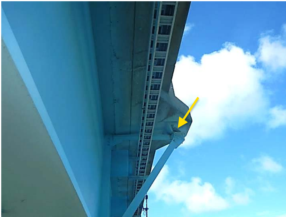
Photo 8.8-18: NCB-SB Span 5 Light Pole – Concrete Support Pedestal Spalled with Exposed Reinforcement (Looking Southwest)
