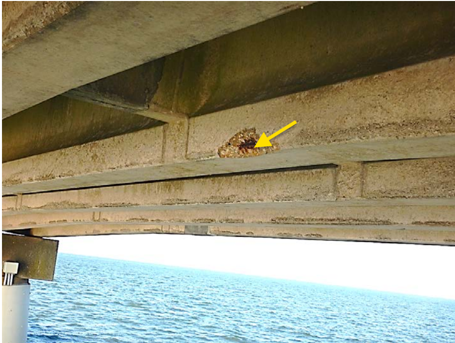
Photo 8.1-7: ANB133 Girder 4 - Spall with 1 Exposed Prestressing Strand (Looking Northeast)
