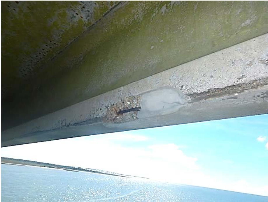
Photo 8.12-9: ESB10 Girder 1 - Failed Repair in Zone 2 with 1 Exposed Prestressing Strands (Looking Southwest)
