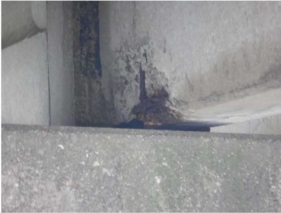
Photo 8.5-17: CNB187 Girder 8 - Failed Repair with Exposed Reinforcement Near Bearing (Looking Northeast)
