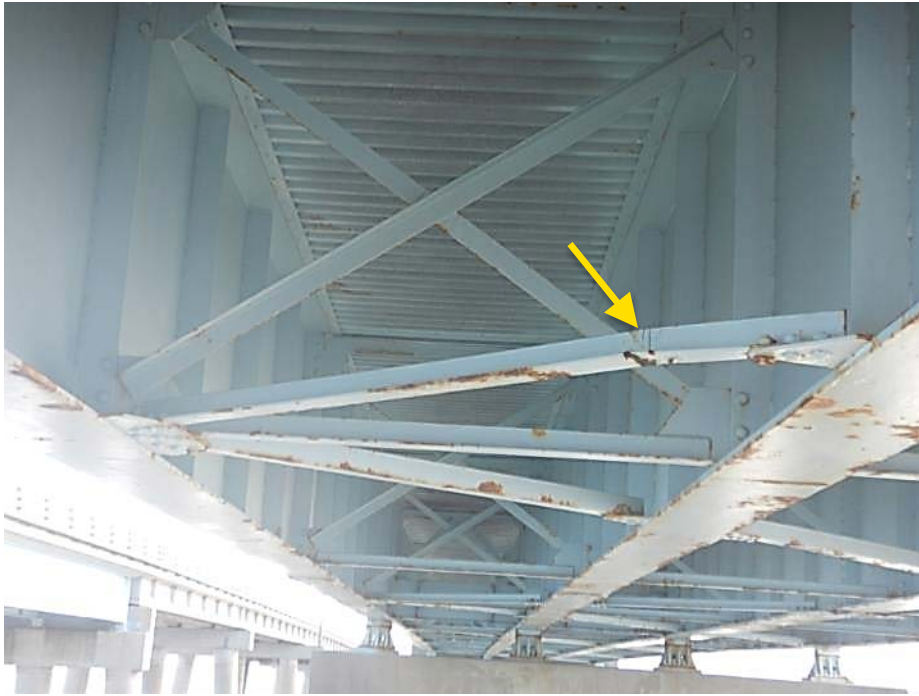
Photo 8.12-15: FIB-SB Span 2, Bay 3, Cross Frame 4 Lower Lateral Bracing - Buckled Lower Lateral Bracing Member with Typical Freckled Rust and Paint Failure (Looking South)
