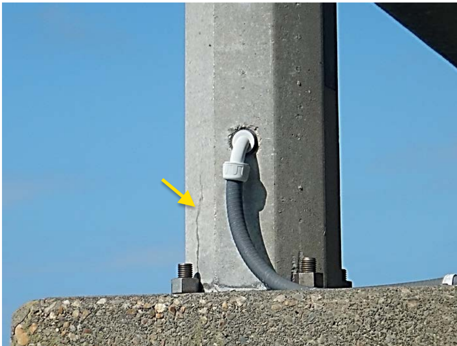
Photo 8.3-20: BNB111 Light Pole – Cracking at Baseplate (Looking Northwest)
