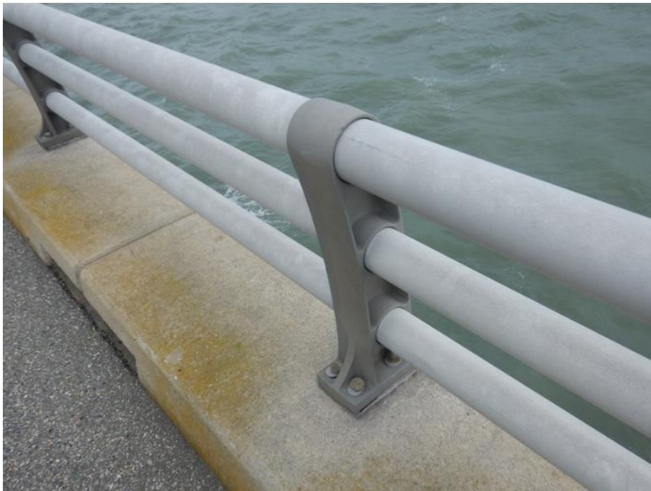
Photo 8.6-2: CSB136 Metal Bridge Railing – Top Connection is Loose, 4 th Post from North (Looking Southwest)
