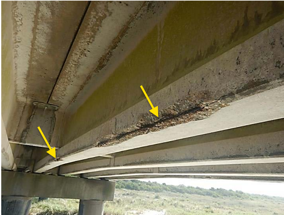
Photo 8.9-9: DNB7 Girder 4 – 2 Spall Locations with 1 Exposed Prestressing Strand (Looking Northeast)
