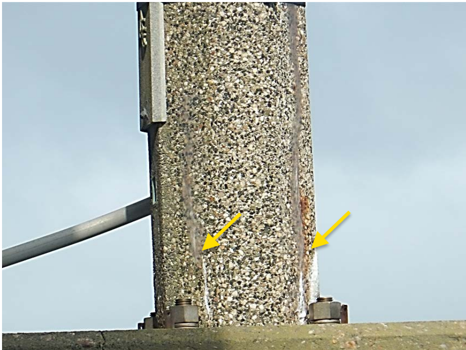
Photo 8.5-30: CNB195 Light Pole – Cracking at Baseplate with Efflorescence and Rust Staining (Looking North)
