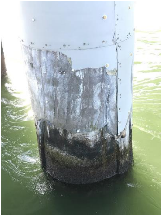
Photo 8.1-13: ANB89 Pile A - Damaged Life Jacket missing Grout and Zinc Mesh on Northwest Quadrant
