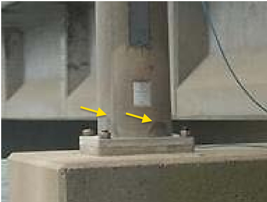
Photo 8.6-16: CSB139 Light Pole – Delamination Near Baseplate (Looking Southwest)
