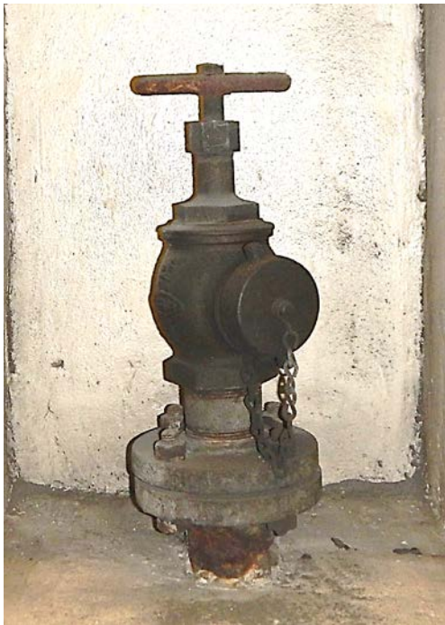
Photo 8.14-14: Hose Valve #35 at STA 519+53 - Corrosion at Concrete Interface
