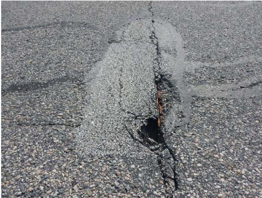
Photo 8.3-3: BNB130 Asphalt Wearing Surface – Deck Spall at Patch (Looking East)
