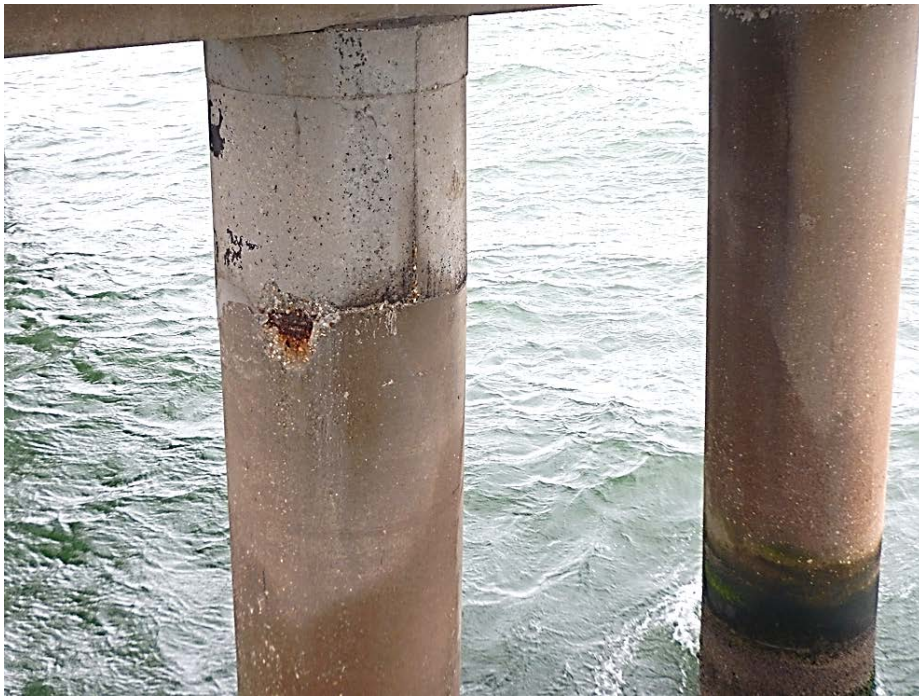
Photo 8.5-20: CNB182 Pile B - Spall with Exposed Reinforcement (Looking Northeast)
