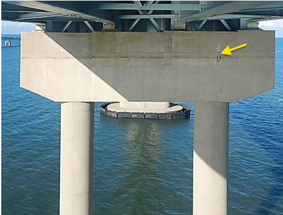
Photo 8.8-13: NCB-SB Pier 11 Reinforced Concrete Pier Cap and Columns - Minor Cracking with Efflorescence (Looking South)
