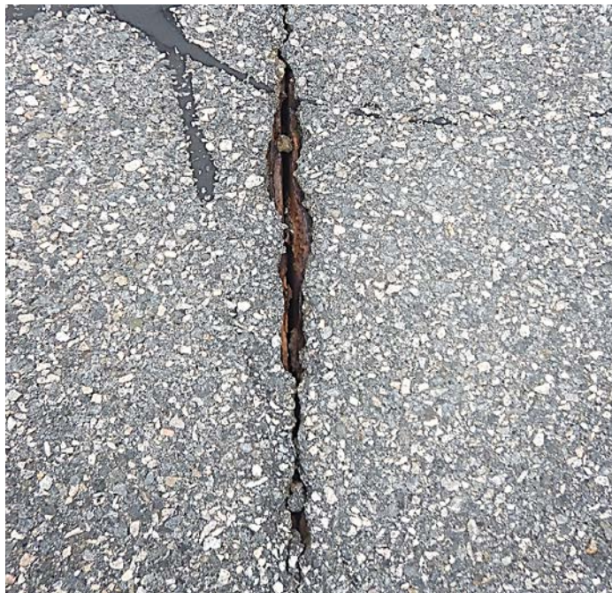
Photo 8.5-6: CNB150 Open Expansion Joint – Steel Joint Header, Worse Condition observed during FY2019 Inspection – Closeup
