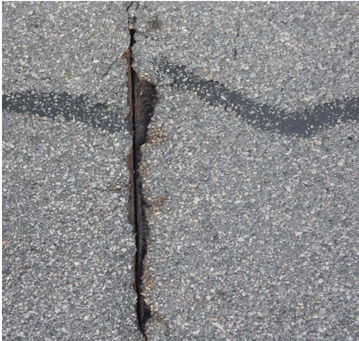
Photo 8.5-9: CNB159 Open Expansion Joint – Steel Joint Header - Closeup
