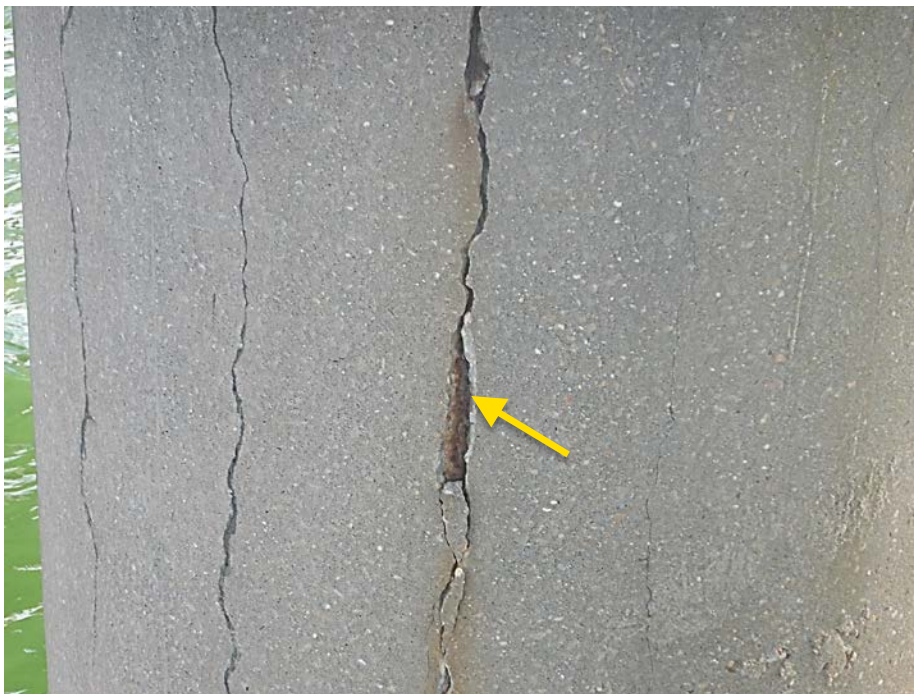
Photo 8.3-18: BNB129 Pile A – Wide Crack along Exposed Prestressing Strand with Efflorescence and Rust Staining (Looking Northeast) - Closeup
