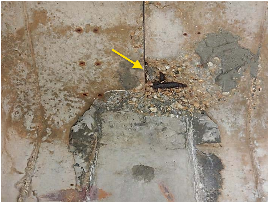
Photo 8.9-2: DNB1 Reinforced Concrete Top Flange (Underside) - Spall with Exposed Reinforcing in Zone 1 between Girder 4 and Girder 5 (Looking South)
