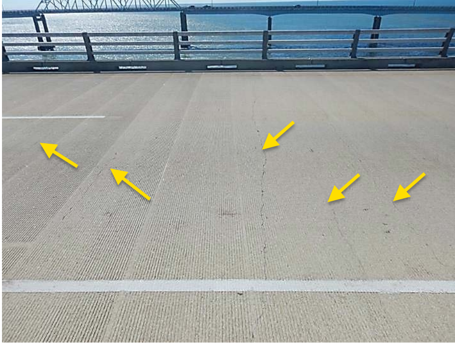
Photo 8.8-1: NCB-SB Span 8 Concrete Deck – Typical Frequent Transverse Cracking (Looking East)
