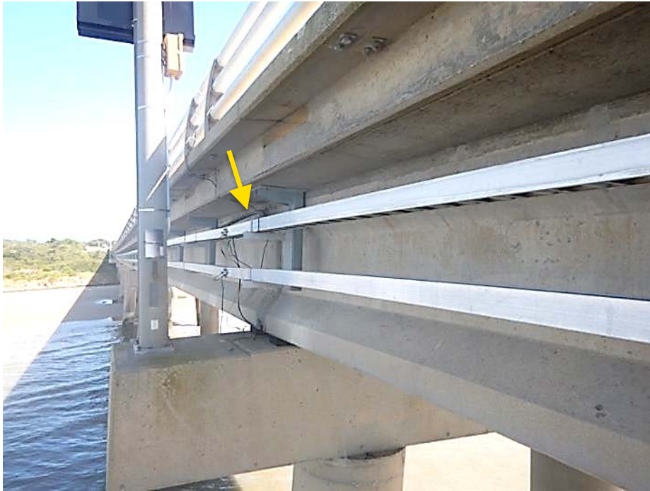
Photo 8.10-9: DSB9 Cable Tray – Cable Displaced from Tray (Looking Northeast)
