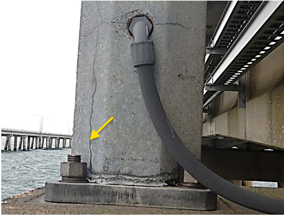
Photo 8.5-31: CNB198 Light Pole – Cracking at Baseplate (Looking North)
