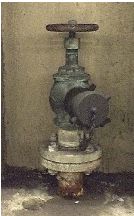
Photo 8.14-8: Hose Valve #4 at STA 474+50 - Corrosion at Concrete Interface
