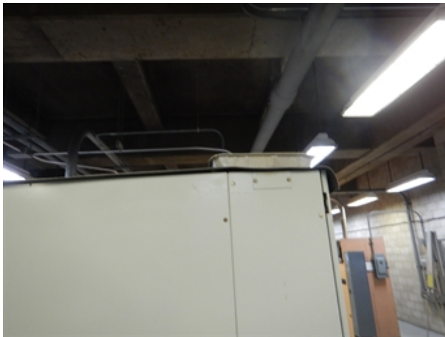
Photo 8.14-28: Emergency Generator System - Portal Island #3 Switchgear Does Not Have a Watertight Seal, and does not have NEC Acceptable Drip Pan at Locations Where Water is Ponding
