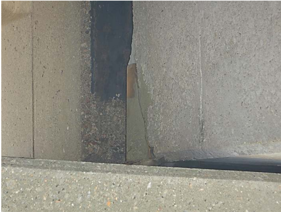
Photo 8.1-5: ANB132 Girder 6 – Failed Repair at Bearing (Looking Southwest)
