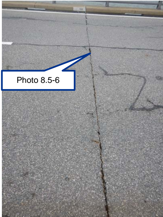
Photo 8.5-5: CNB150 Open Expansion Joint that has been Paved over Exhibiting Reflective Cracking (Looking East)
