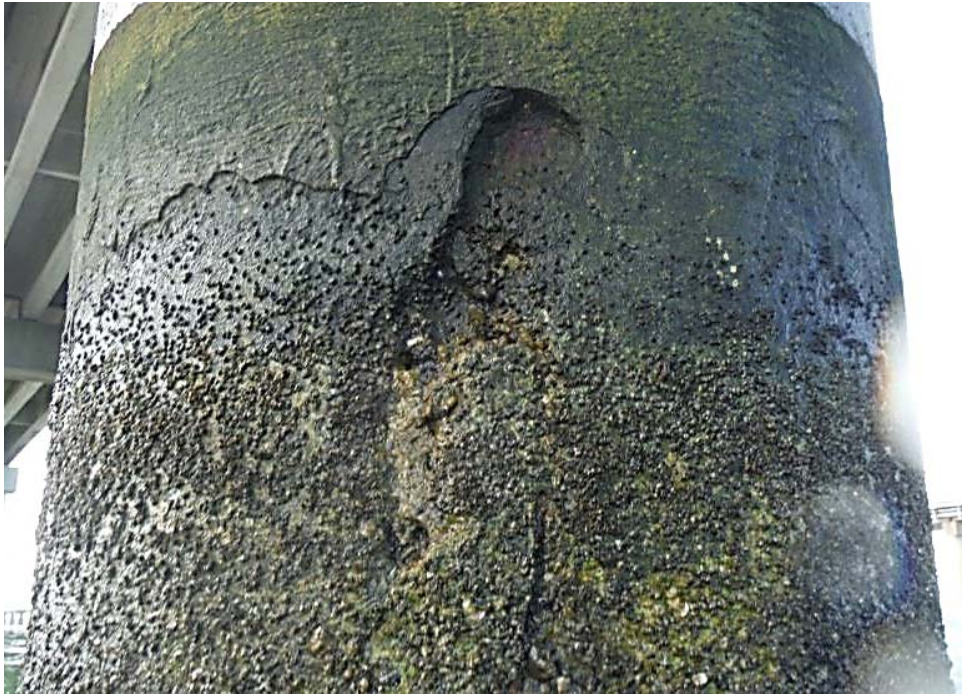
Photo 8.1-15: ANB112 Pile B - Protective Coating Failures with Cracking, Spalling, and Rust Staining (Looking South)
