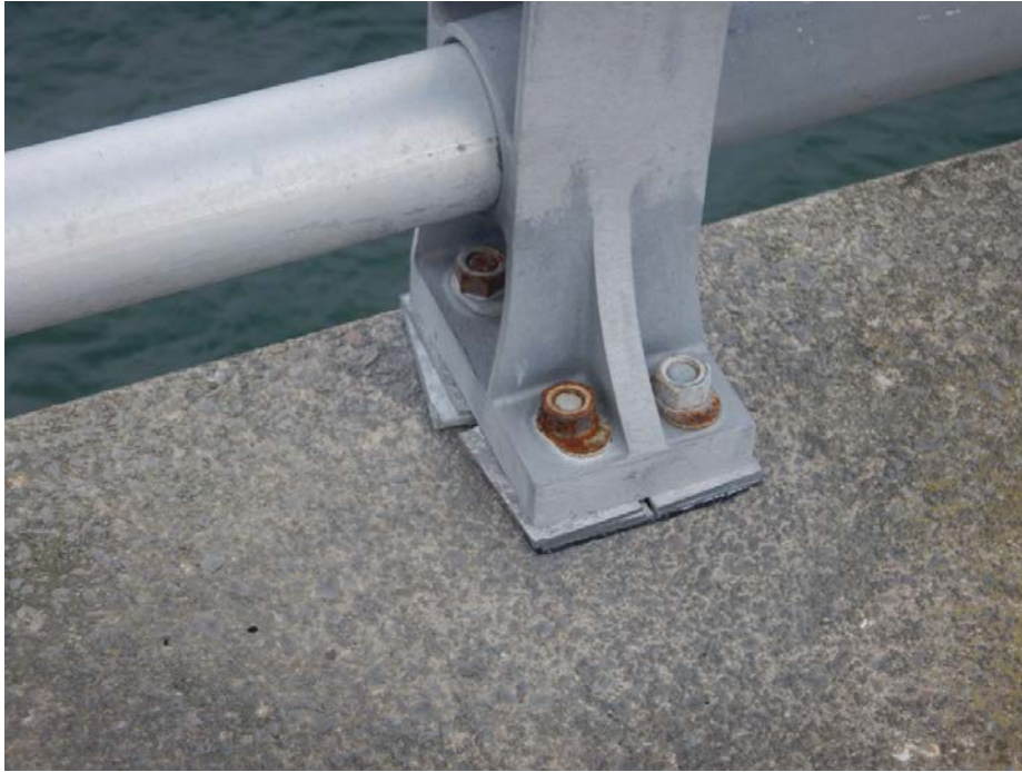
Photo 8.5-1: CNB171 Metal Bridge Railing 1 st Post from the South – Rust and Tightly Fastened Connection Results in Bolts that do not Extend Above Nuts (Looking Northwest)
