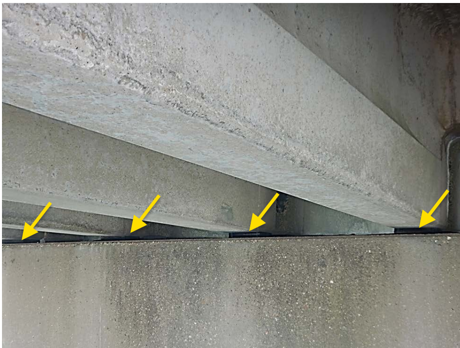
Photo 8.5-18: CNB138 Elastomeric Bearings at Girders 4, 5, 6, & 7 - Split with Exposed and Corroded Steel Plates (Looking Northwest)
