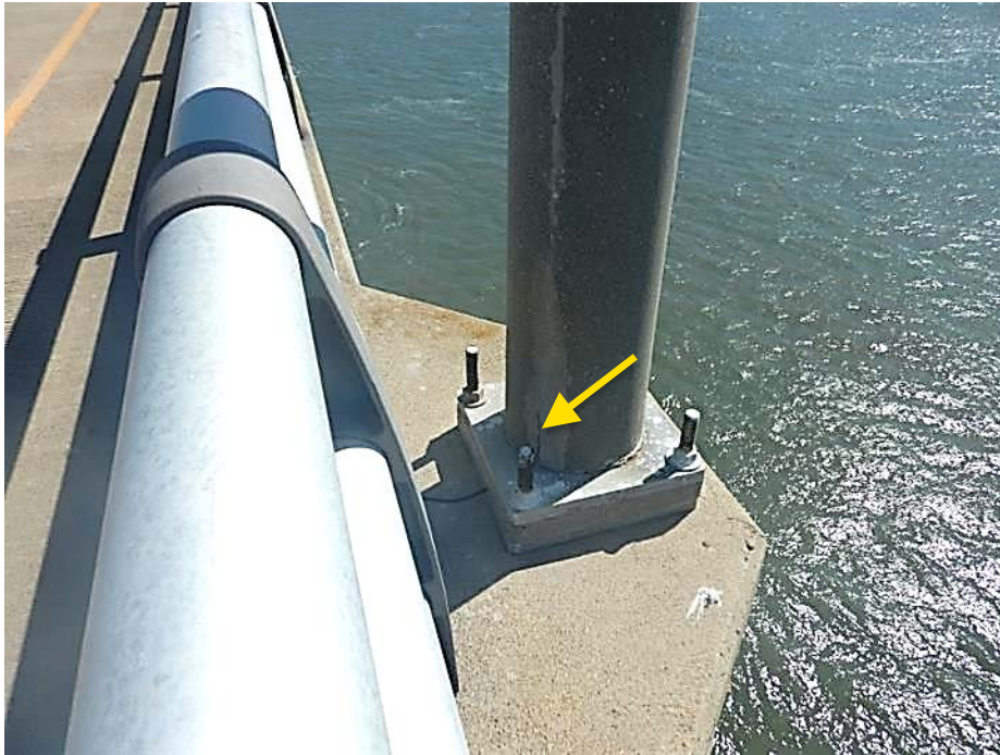
Photo 8.8-19: NCB-SB Span 6 Southeast Light Pole – Cracking at Baseplate (Looking Northeast)
