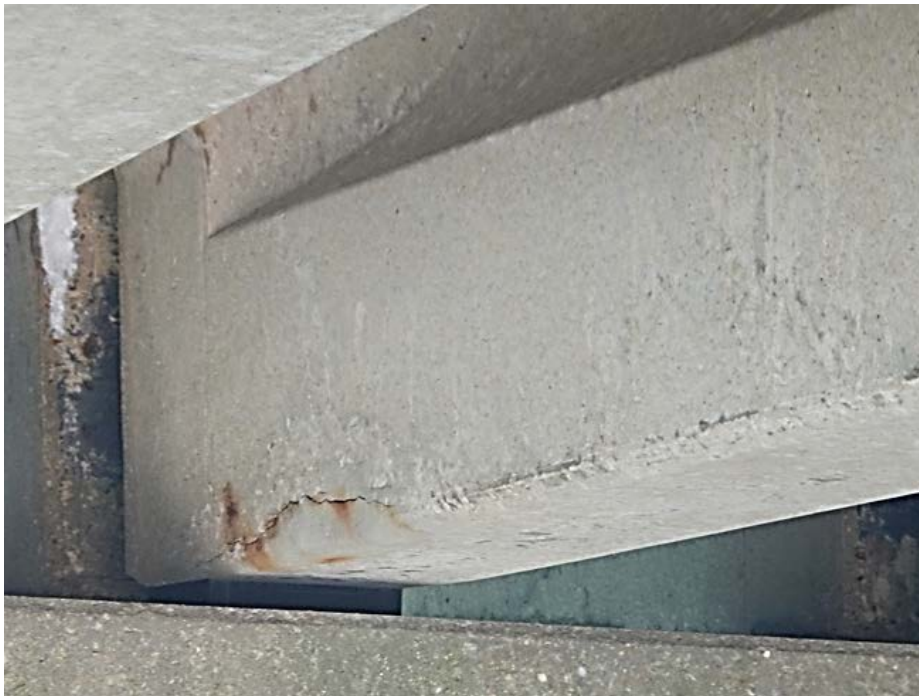
Photo 8.5-12: CNB138 Girder 8 - Failed Repair with Rust Staining Near Bearing (Looking Northeast)
