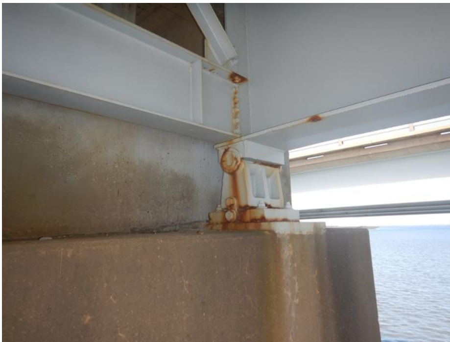
Photo 8.12-16: FIB-SB Pier 4 G4 Movable Bearing - Typical Condition of Isolated areas of Surface Rust (Looking Southwest)
