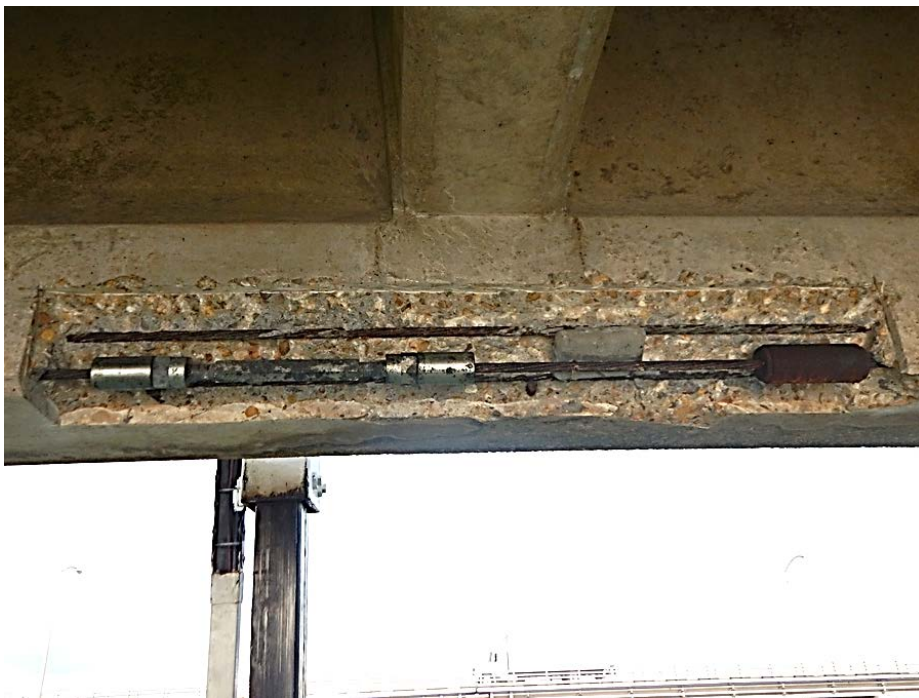
Photo 8.1-8: ANB149 Girder 8 - Girder Spall and Prestressing Strand Repair Preparation exhibiting Corrosion along Replacement Strand and Coupler (Looking West) ~ The District Corrected and Completed the Repair per Email dated 11/20/2018
