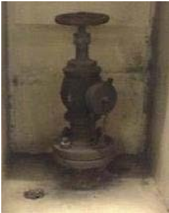
Photo 8.14-10: Hose Valve #27 at STA 508+10 - Corrosion at Concrete Interface
