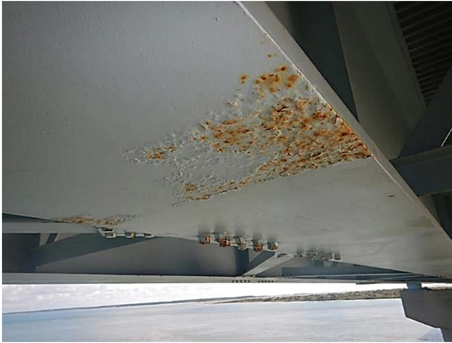
Photo 8.8-7: NCB-SB Span 9 Girder 2 – Top Protective Coating Bubbling with Freckled Rust (Looking Northwest)
