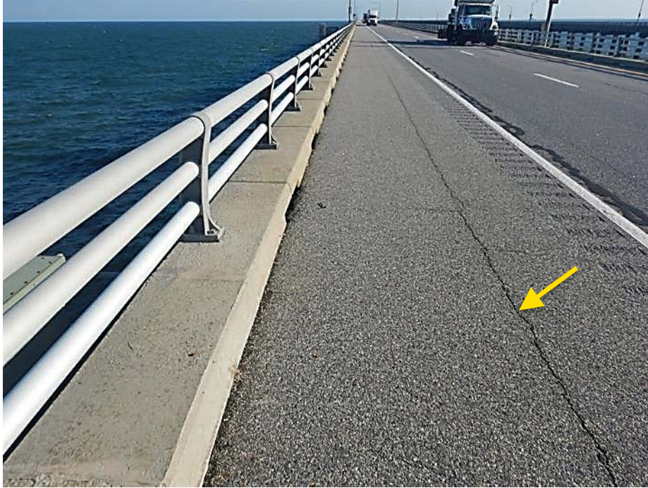
Photo 8.4-1: BSB104 Asphalt Wearing Surface – Crack along Pavement extends to BSB105 (Looking North)
