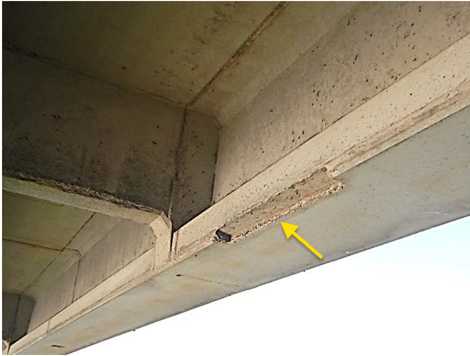
Photo 8.2-3: ASB117 Girder 1 – Portion of Bottom Corner Missing (appears to have been constructed this way) (Looking Southeast)
