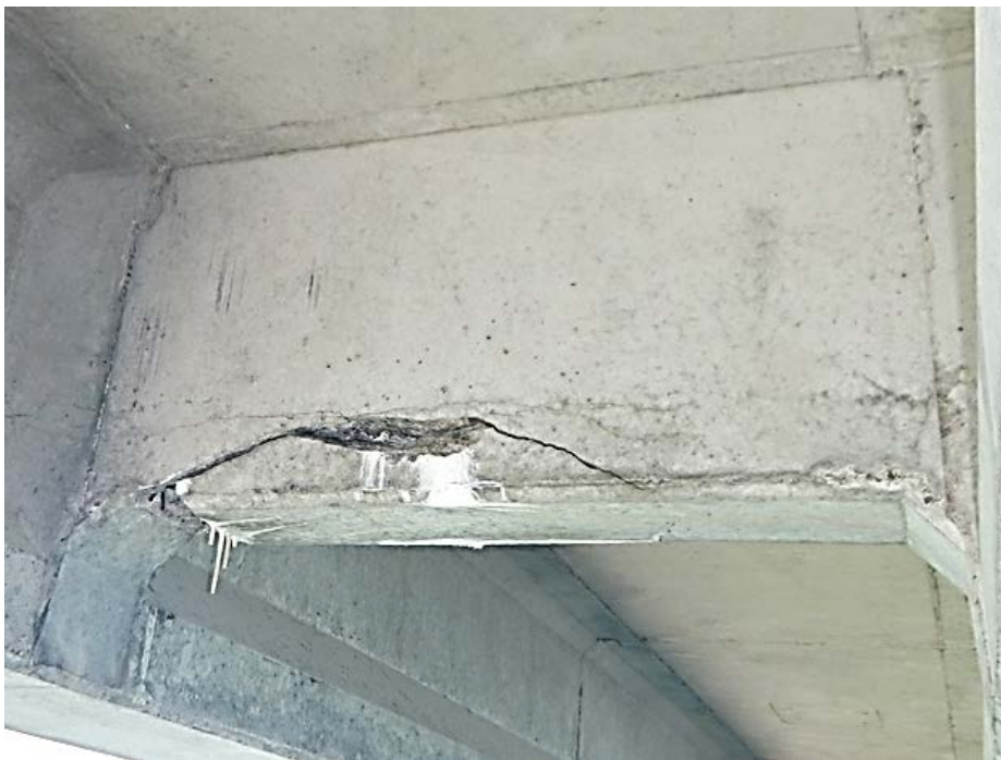
Photo 8.2-4: ASB93 Bay 5 Zone 1/2 Intermediate Diaphragm – Spalling, Cracking, and Efflorescence Surrounding the Lower Post Tension Duct (Looking Southeast)
