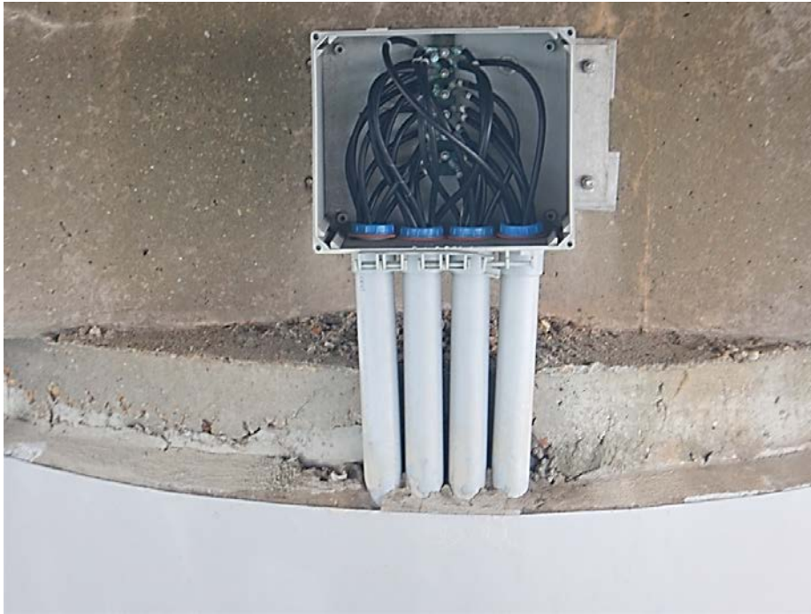
Photo 8.5-21: CNB183 Pile B – Life Jacket Rectifier with No Cover (Looking North)
