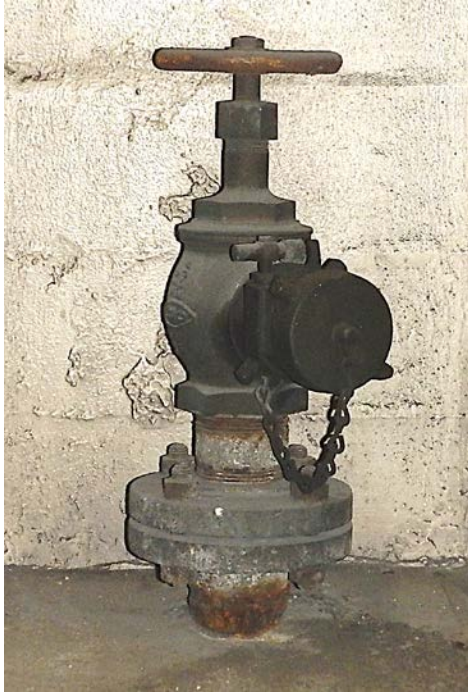
Photo 8.14-15: Hose Valve #36 at STA 521+10 - Corrosion at Concrete Interface
