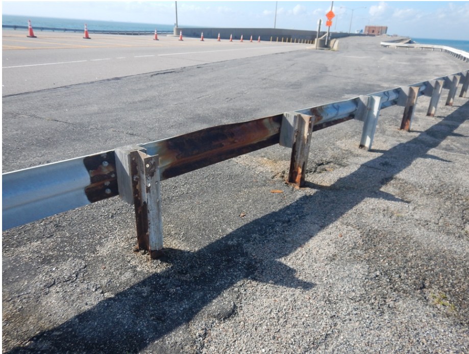
Photo 8.15-31: Portal Island 4 – Northwest Guardrail with Impact Damage and Corrosion with Isolated Areas of Significant Section Loss (Looking Southeast)
