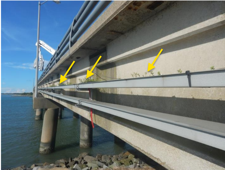
Photo 8.12-19: ESB1 Cable Tray - Vegetation Along the Entire Top Tray (Looking Northeast)
