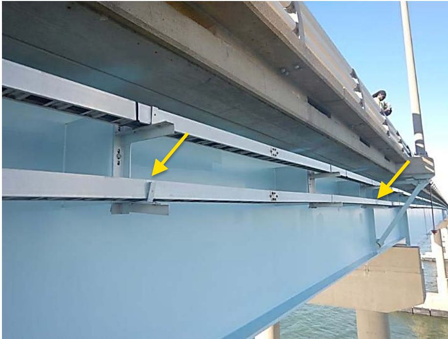
Photo 8.8-15: NCB-SB Span 11 Cable Tray – Lower Cable Tray Detached at 2 Clips Adjacent to Light Pole (Looking Southeast)
