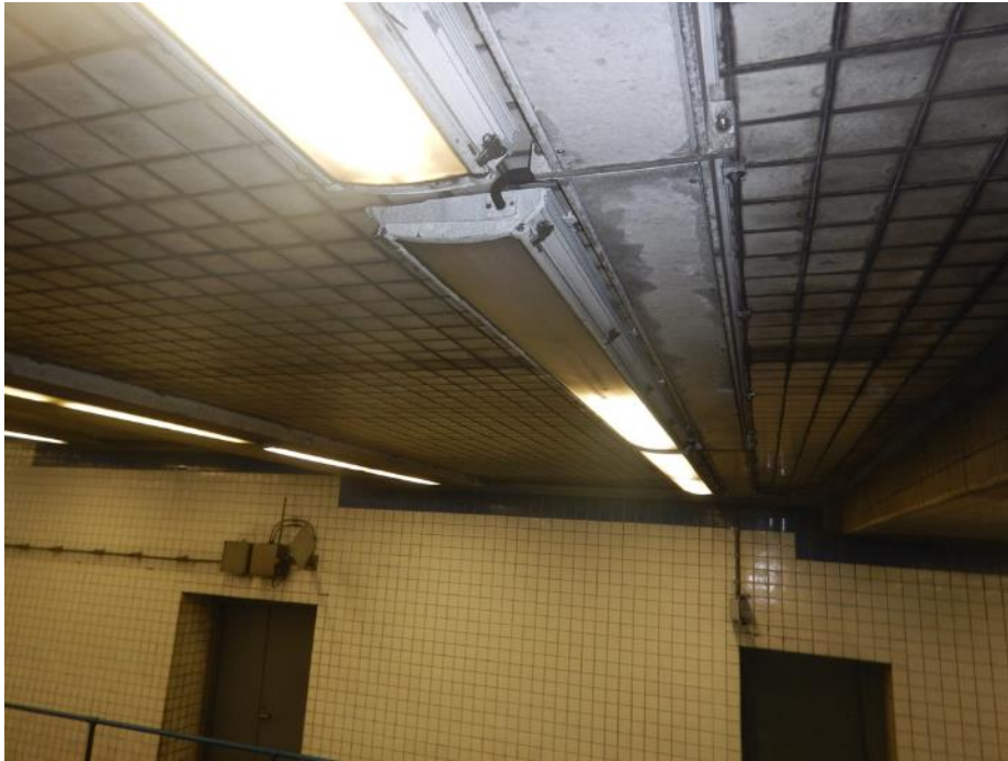
Photo 8.14-19: Light on Sidewalk Side at STA 469+85 - Light Bulb is not Lighting
