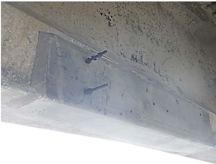
Photo 8.5-16: CNB187 Girder 1 - Galvanized Hardware used for Core Extraction should be removed (Looking Southeast)
