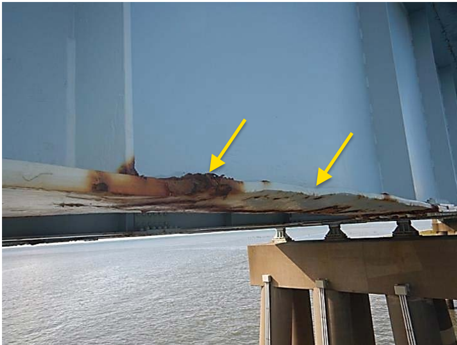
Photo 8.12-14: FIB-SB Span 2 Girder 4 – Bottom Flange Distorted for 3' on East Edge (No Mitigation Required) with Typical Freckled Rust and Paint Failure (Looking Northwest)
