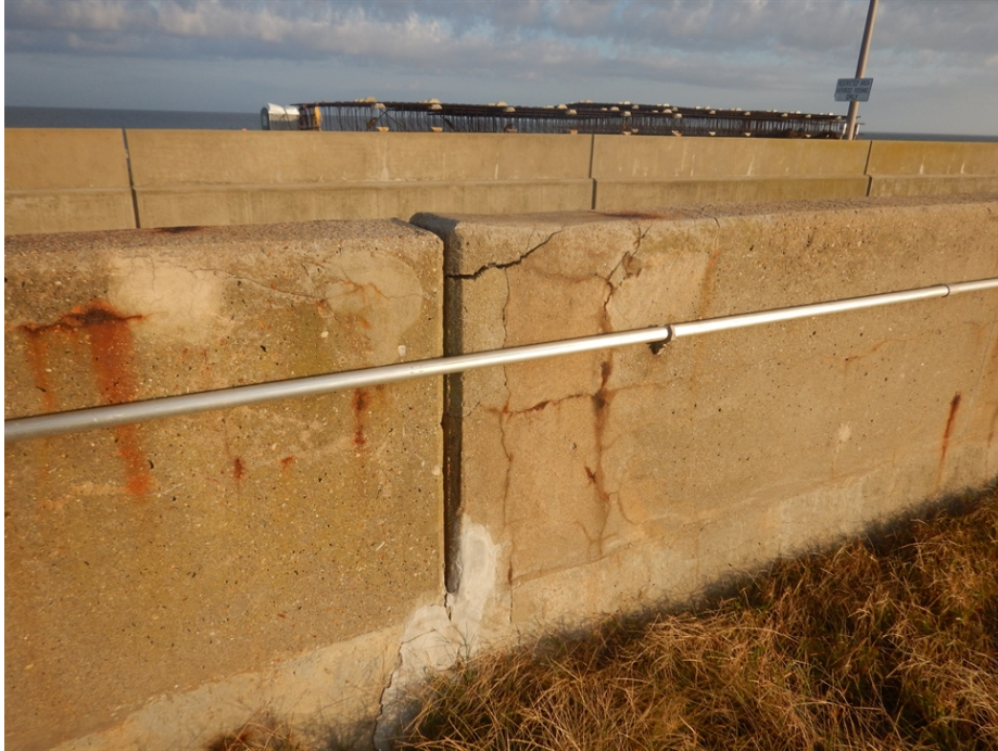
Photo 8.15-1: Portal Island 3 – Spalling on top of East Approach Wall Approximately 200' from South (Looking Northwest)
