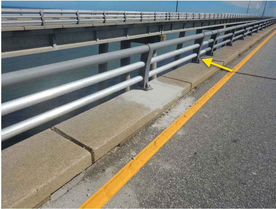
Photo 8.12-3: FSB6 Metal Bridge Railing - Disconnected Grounding Cable at Location of Recent Repair (Looking Southeast)
