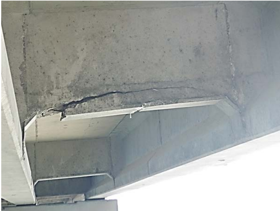
Photo 8.2-5: ASB82 Bay 1 Zone 2/3 Intermediate Diaphragm – Spalling, Cracking, and Efflorescence Surrounding the Lower Post Tension Duct (Looking Southeast)
