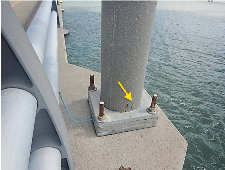
Photo 8.8-17: NCB-SB Span 2 Southeast Light Pole – Cracking at Baseplate (Looking Northeast)
