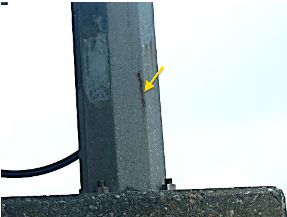
Photo 8.5-26: CNB162 Light Pole – Cracking near Baseplate with Rust Staining (Looking Southwest)
