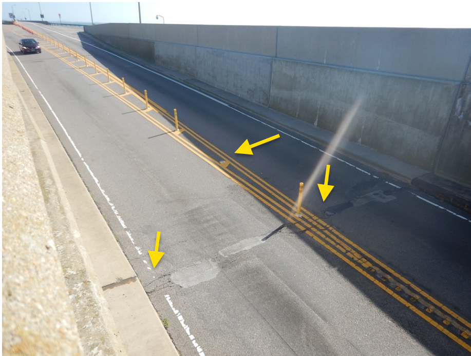
Photo 8.15-26: Portal Island 4 – Missing Delineator Post and Asphalt Cracking and Surface Spalling
