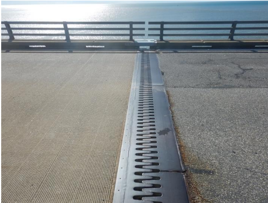
Photo 8.12-7: FIB-SB Pier 4 Assembly Joint without Seal - Tooth Expansion Joint Typical Condition with Minor and Isolated Locations of Freckled Rust (Looking West)
