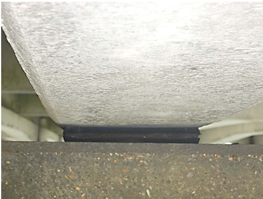
Photo 8.1-10: ANB146 Elastomeric Bearing at Girder 4 - Split with Exposed and Corroded Steel Plates (Looking South)
