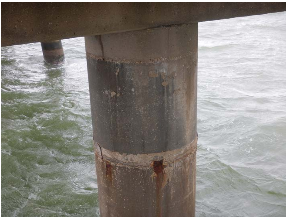
Photo 8.5-24: CNB193 Pile B - Spall with Exposed Reinforcement (Looking Northeast)
