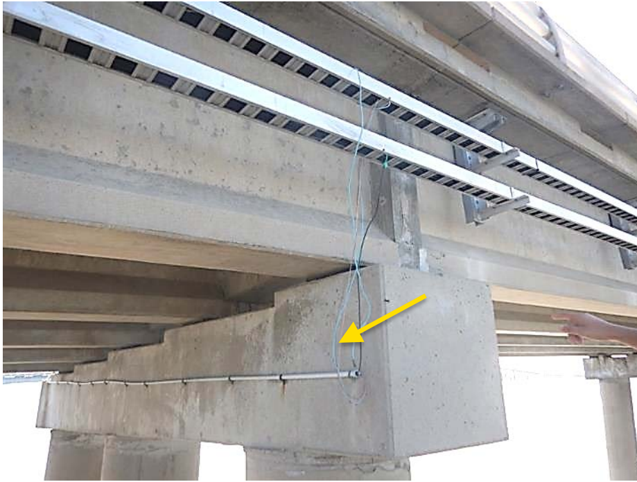
Photo 8.10-7: DSB7 Cable Tray – Blue Cable Disconnected (Looking Southeast)
