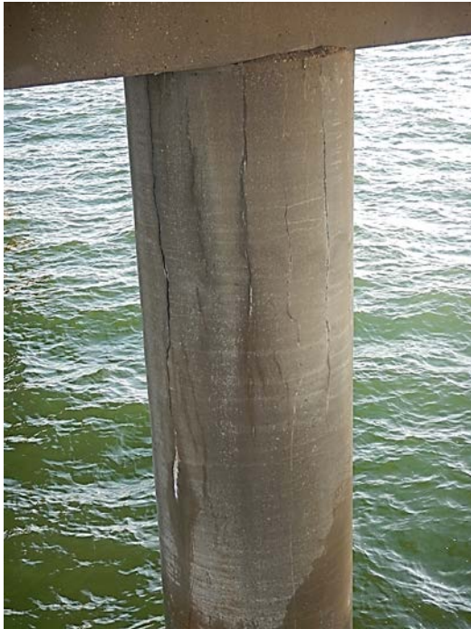
Photo 8.3-15: BNB121 Pile B – Wide Cracks with Efflorescence (Looking Northeast)
