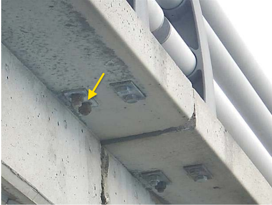
Photo 8.6-1: CSB115 Metal Bridge Railing – Loose Anchor Bolt Connection near Bent CSB115 (Looking Northwest)
