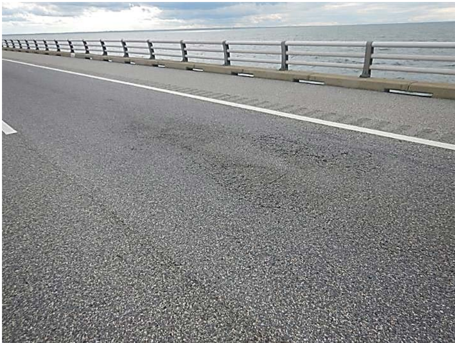
Photo 8.6-4: CSB110 Asphalt Wearing Surface – Typical Abrasion and Scaling (Looking Southwest)
