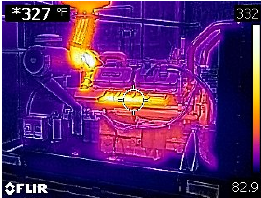
Photo 8.14-33: Emergency Generator System - Thermal Image of Portal Island #4 Generator
