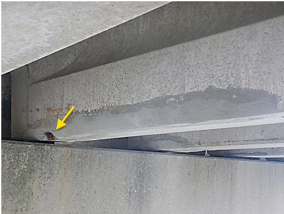
Photo 8.5-14: CNB138 Girder 8 - Failed Repair with Rust Staining Near Bearing (Looking Northeast)
