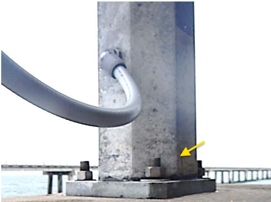
Photo 8.5-28: CNB186 Light Pole – Cracking at Baseplate (Looking Northwest)
