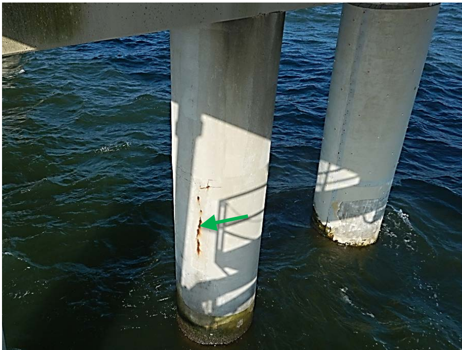
Photo 8.1-20: BNB135 Pile B - Cracks through Protective Coating with Rust Staining (Looking Northeast)
