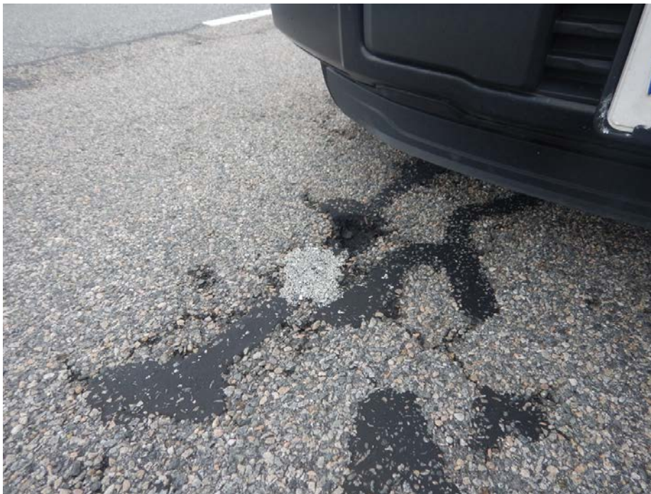
Photo 8.5-10: CNB184 Asphalt Wearing Surface – Surface Spalling and Cracking (Looking Southeast)
