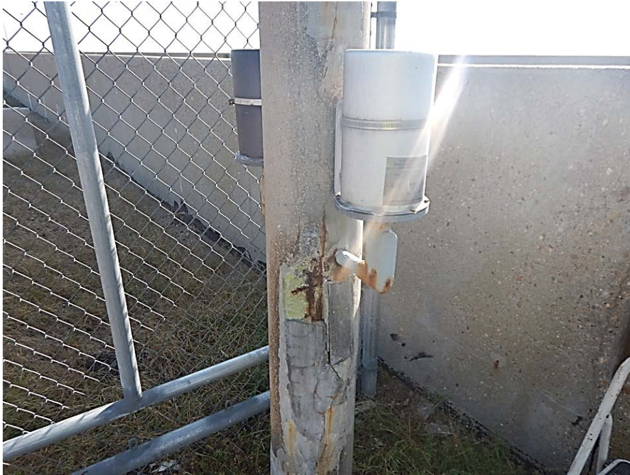
Photo 8.15-27: Portal Island 4 – Southwest Light Pole with Spalling with Exposed Reinforcement and Cracking extending towards the Base (Looking Northeast)
