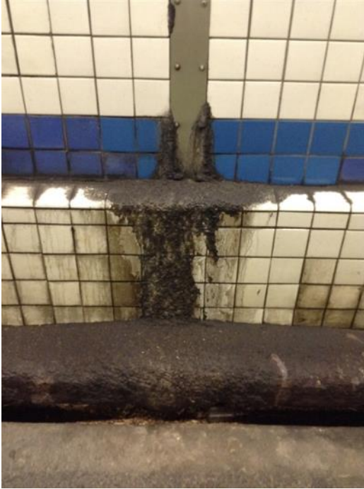
Photo 8.14-1: Drainage Channel Clean Out Plate at STA 489+50 - Clogged, Typical for Clean Out Plates
