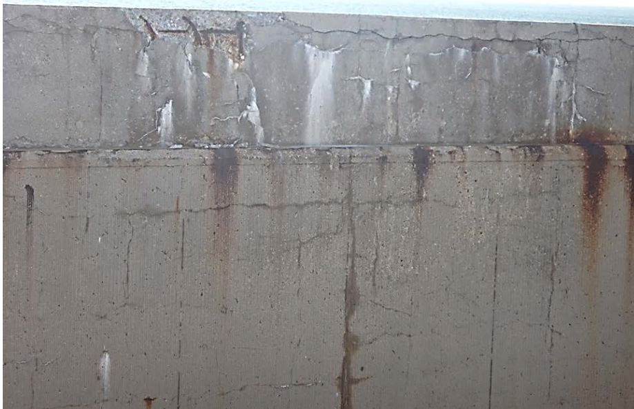
Photo 8.15-12: Portal Island 3 – Spalling with Exposed Reinforcement on top of East Approach Wall Approximately 500' from South (Looking Southeast)
