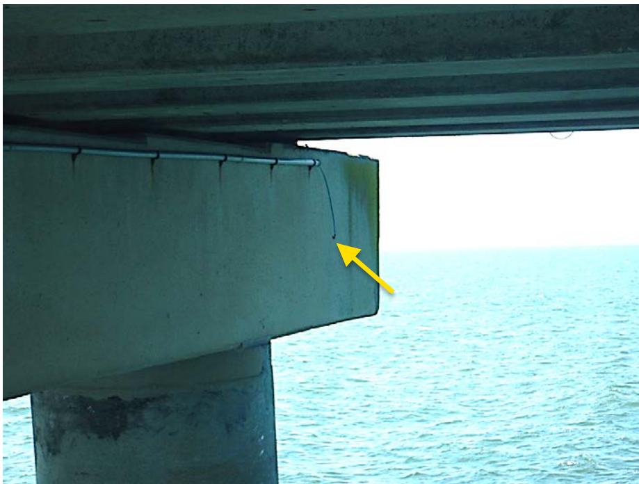
Photo 8.2-6: ASB Bent 96 - Disconnected Cable (Looking Southwest)
