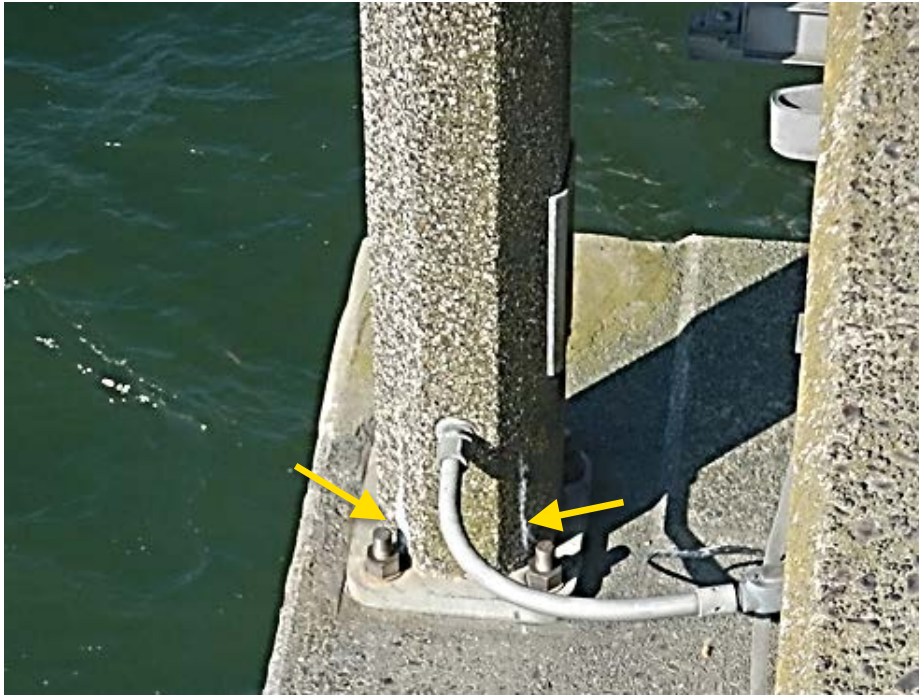
Photo 8.1-21: ANB129 Light Pole – Cracking at Baseplate (Looking Northwest)
