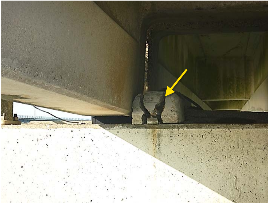
Photo 8.1-11: ASB Bent 135 – Spalled Shear Tab (Looking Northwest)
