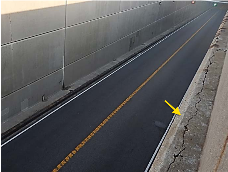
Photo 8.15-3: Portal Island 3 – Cracking/Delamination on East Approach Wall Approximately 700’ from South (Looking Northwest)
