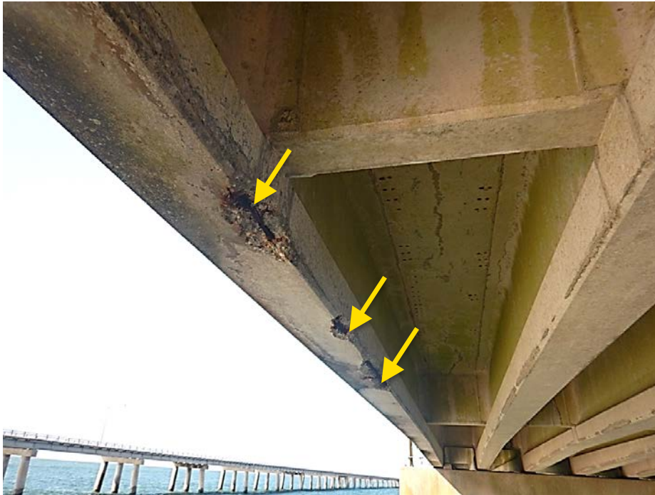
Photo 8.3-7: BNB116 Girder 8 - Spall with 1 Exposed Prestressing Strand, 3 Locations (Looking Northwest)
