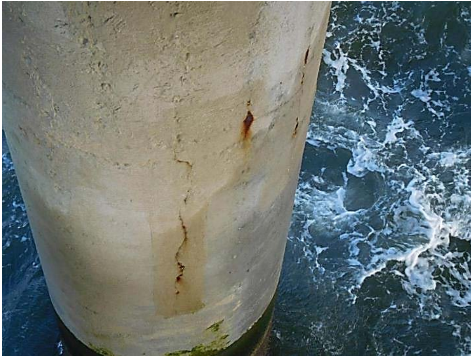
Photo 8.1-17: ANB117 Pile A - Cracks through Protective Coating with Rust Staining (Looking Northwest)
