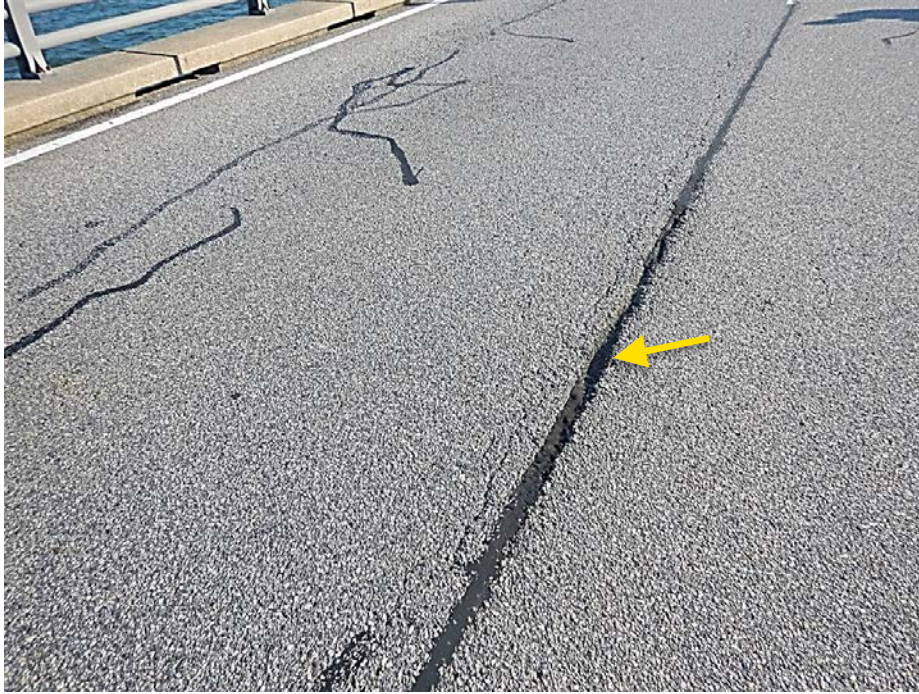
Photo 8.1-1: ANB129 Asphalt Wearing Surface – Surface Spall along Center Line (Looking Southeast)
