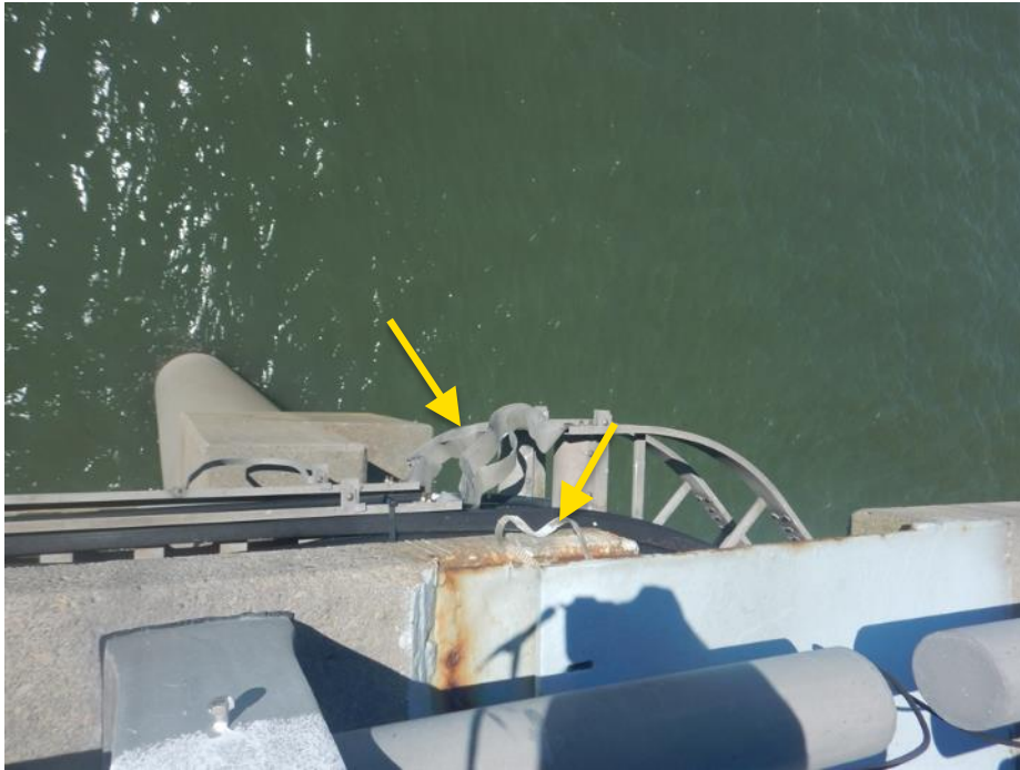
Photo 8.12-21: FIB-SB Pier 1 Cable Tray - 2 Broken Cable Tray Expansion Straps (Looking West)
