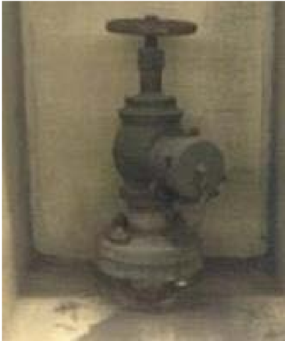
Photo 8.14-9: Hose Valve #22 at STA 500+79 - Corrosion at Concrete Interface
