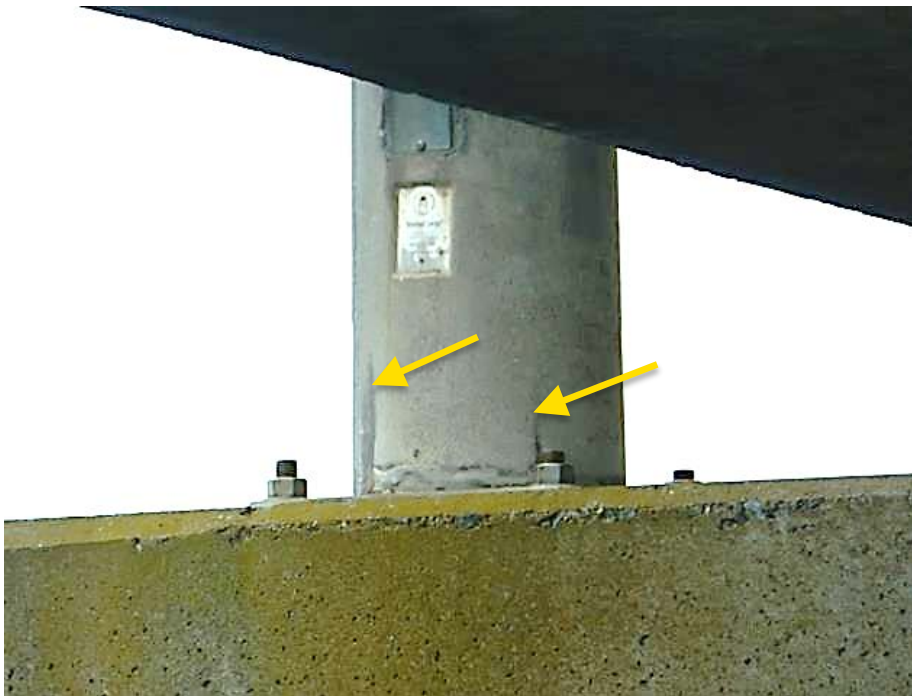
Photo 8.6-18: CSB147 Light Pole – Vertical Cracking Near Baseplate (Looking Northwest)
