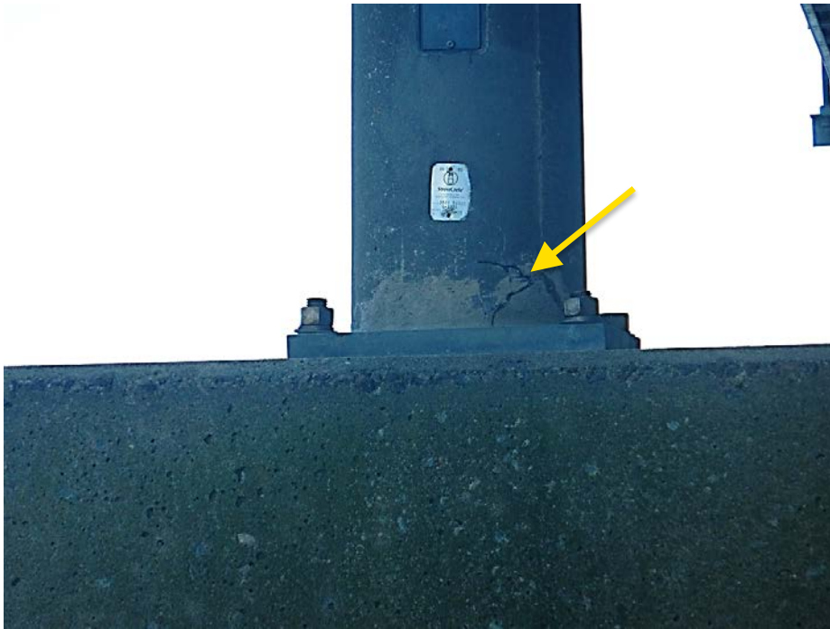
Photo 8.2-7: ASB87 Light Pole – Vertical Cracking Near Baseplate (Looking Southwest)
