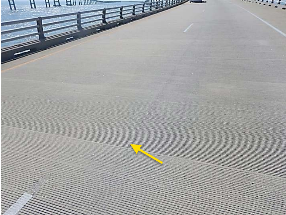
Photo 8.10-1: DSB9 Concrete Deck – Narrow Width Longitudinal Crack, Full Span Length (Looking Southeast)
