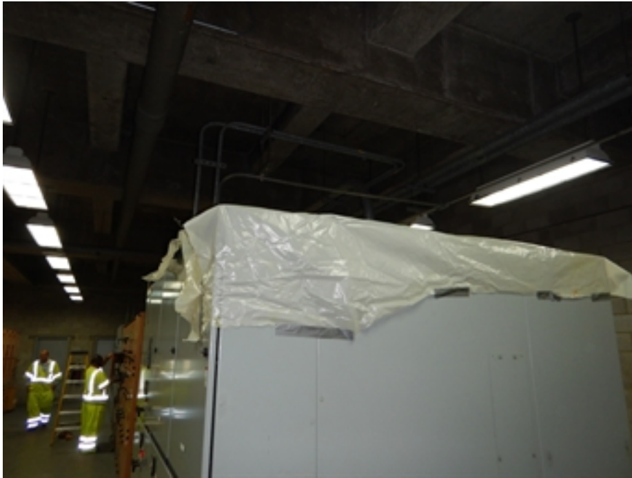
Photo 8.14-29: Emergency Generator System - Portal Island #4 Switchgear Does Not Have a Watertight Seal, and does not have NEC Acceptable Drip Pan at Locations Where Water is Ponding
