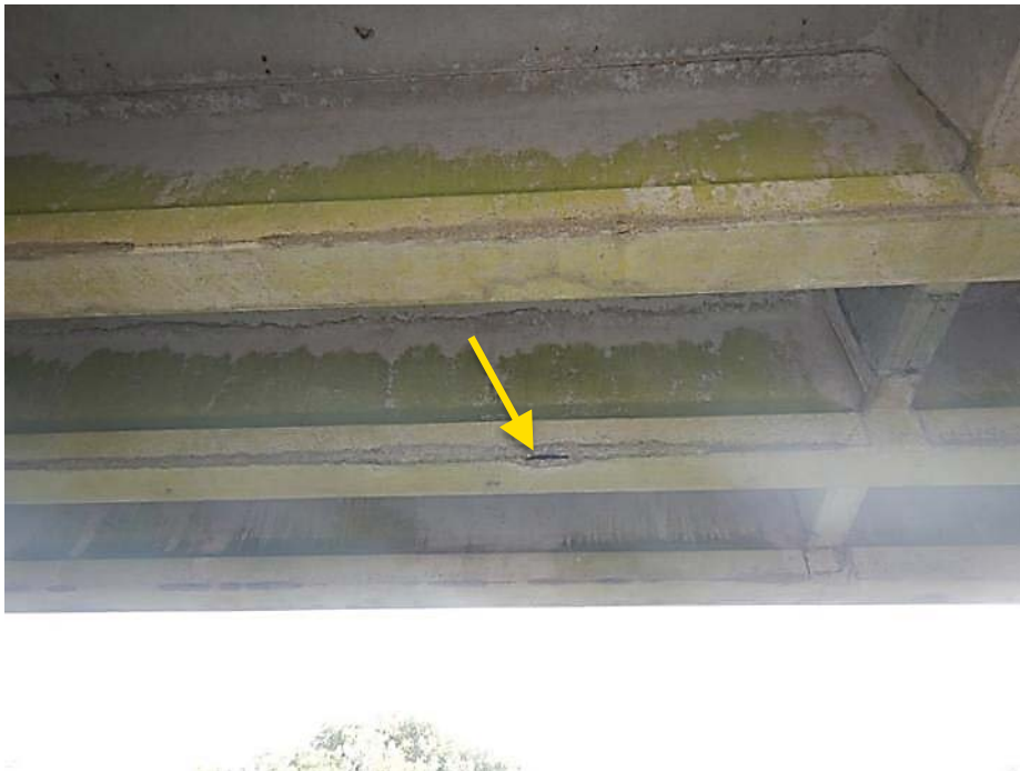
Photo 8.9-10: DNB11 – Girder 2 – Spall with 1 Exposed Prestressing Strand (Looking East)
