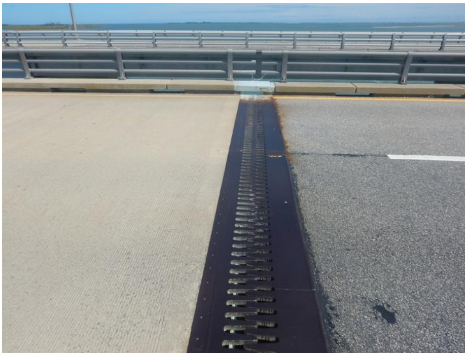
Photo 8.12-6: FIB-SB Pier 1 Assembly Joint without Seal - Tooth Expansion Joint Typical Condition with Minor and Isolated Locations of Freckled Rust (Looking East)
