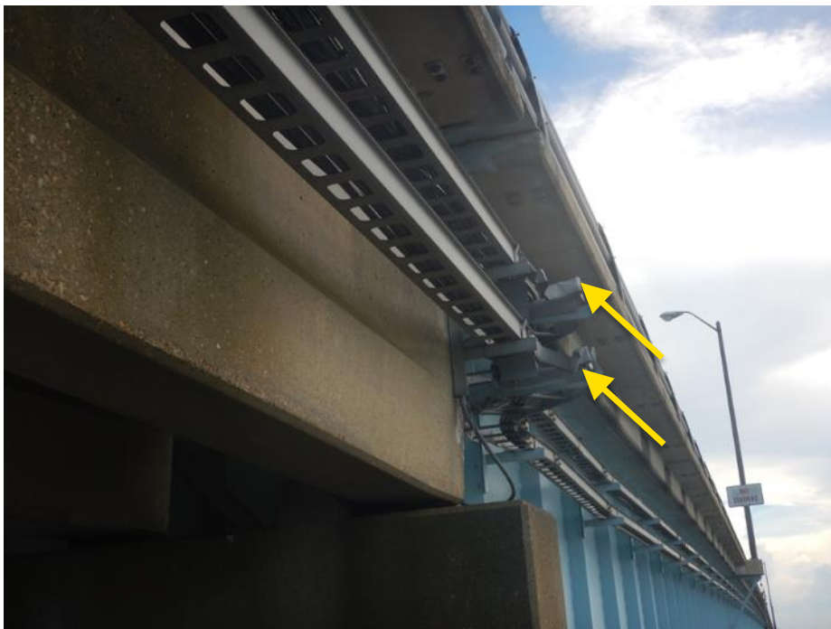
Photo 8.12-22: FIB-SB Pier 4 Cable Tray - 2 Broken Cable Tray Expansion Straps (Looking Southeast)
