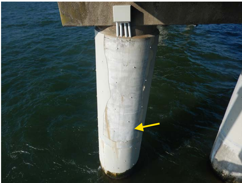
Photo 8.1-18: BNB133 Pile A - Life Jacket with Damaged Fiberglass Jacket and Slightly Exposed Zinc Mesh (Looking North)
