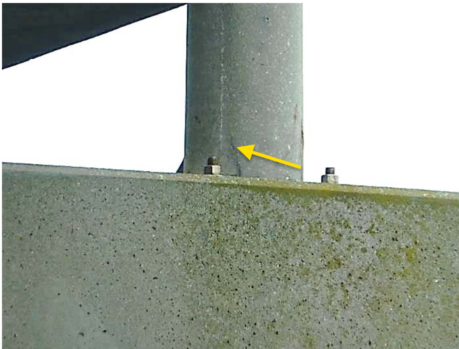
Photo 8.6-20: CSB151 Light Pole – Vertical Cracking Near Baseplate (Looking Southwest)
