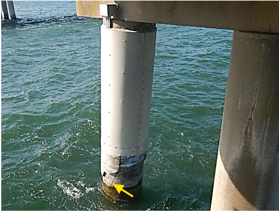
Photo 8.3-13: BNB116 Pile A - Damaged Life Jacket missing Grout and Zinc Mesh on Southeast Quadrant with Exposed Cable (Looking Northwest)
