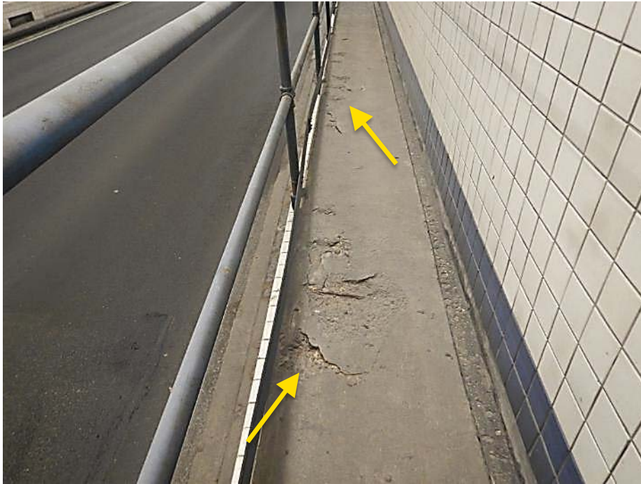
Photo 8.14-3: Sidewalk at STA 511+30 - Spalling with Exposed Reinforcement
