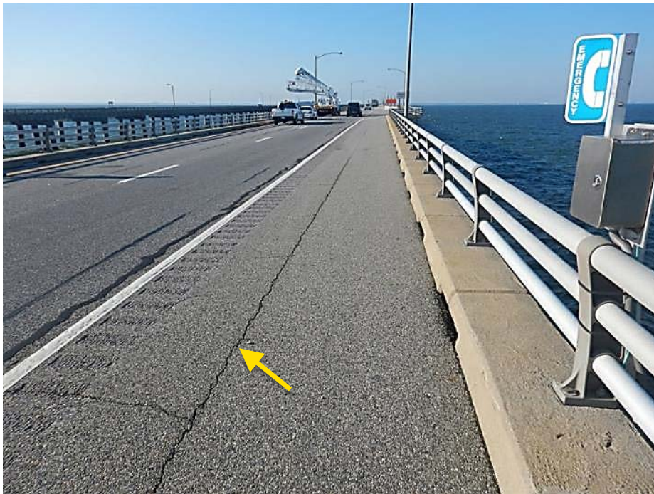
Photo 8.4-2: BSB103 Asphalt Wearing Surface – Crack along Pavement extends to BSB102 (Looking South)
