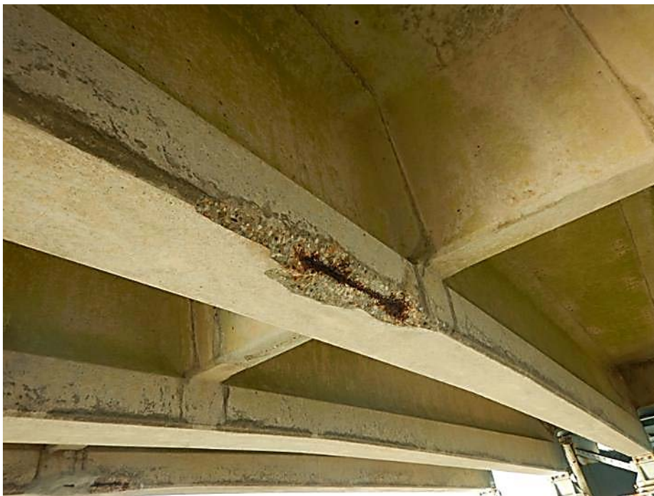
Photo 8.9-4: DNB1 Girder 3 - Spall with 1 Exposed Prestressing Strand (Looking Southeast)
