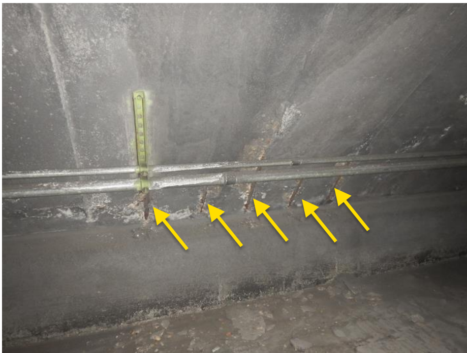
Photo 8.14-22: Exhaust Duct Liner at STA 482+70 - Spalling with Exposed Transverse Reinforcement (Little to No Section Loss of Steel Reinforcement, Looking East)
