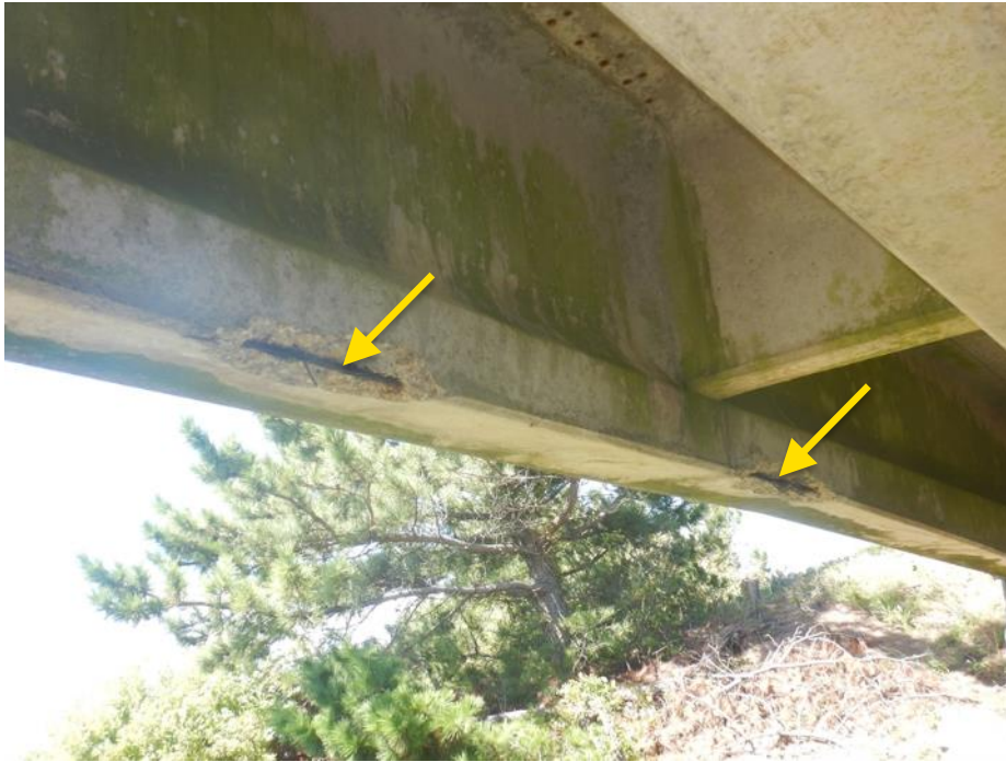
Photo 8.12-13: FSB8 Girder 1 - Two Spalls with 1 Exposed Prestressing Strand (Looking Northwest)
