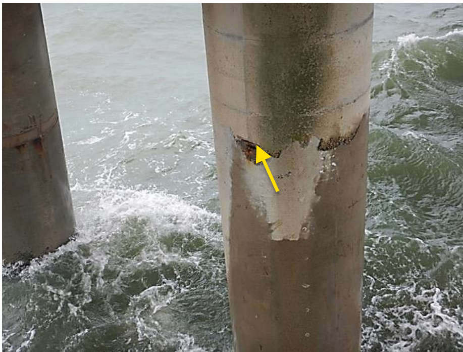
Photo 8.6-8: CSB128 Pile B - Spall with Exposed Reinforcement Spirals (Looking North)
