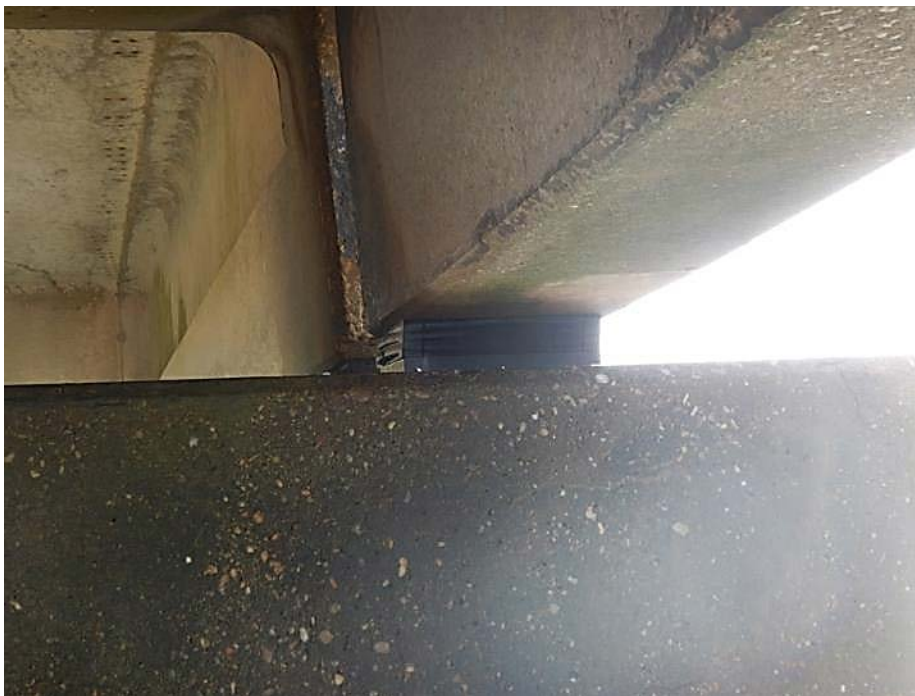
Photo 8.9-12: DNB1 Girder 1 – Elastomeric Bearing Bulging Greater than 15% of Thickness (Looking North)
