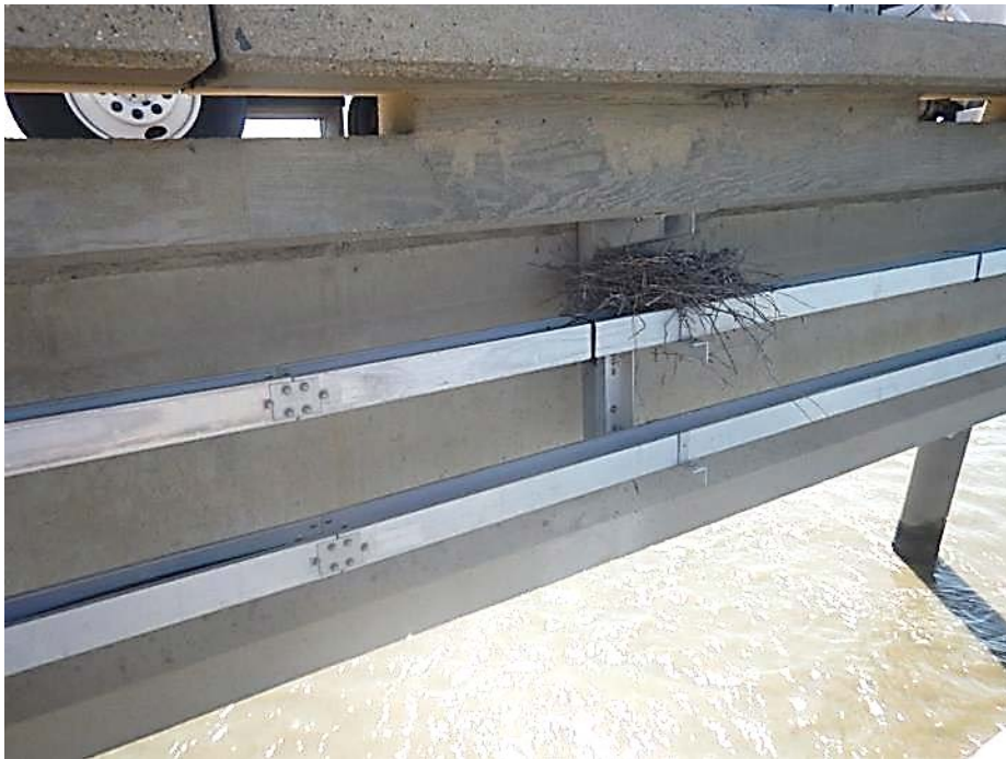
Photo 8.10-8: DSB9 Cable Tray – Debris in Cable Tray (Looking Southeast)
