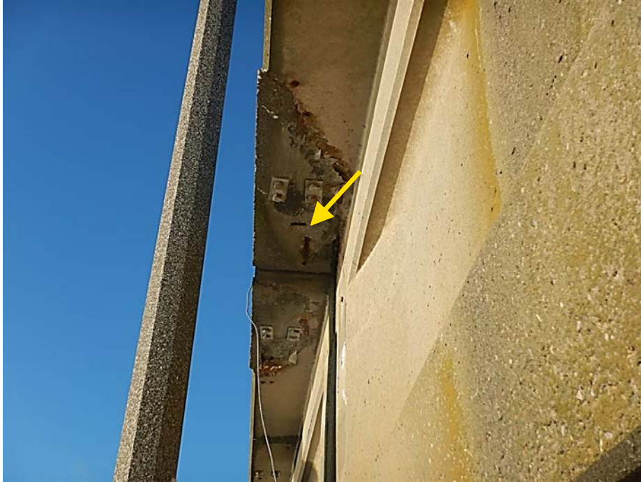
Photo 8.3-1: BNB119 Metal Bridge Railing – Failed Curb Repair with Exposed Reinforcement (Looking South)
