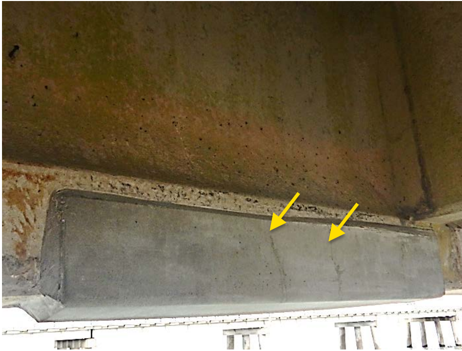
Photo 8.5-13: CNB147 Girder 8 - Repair with Minor Transverse Cracking (Looking Northwest)
