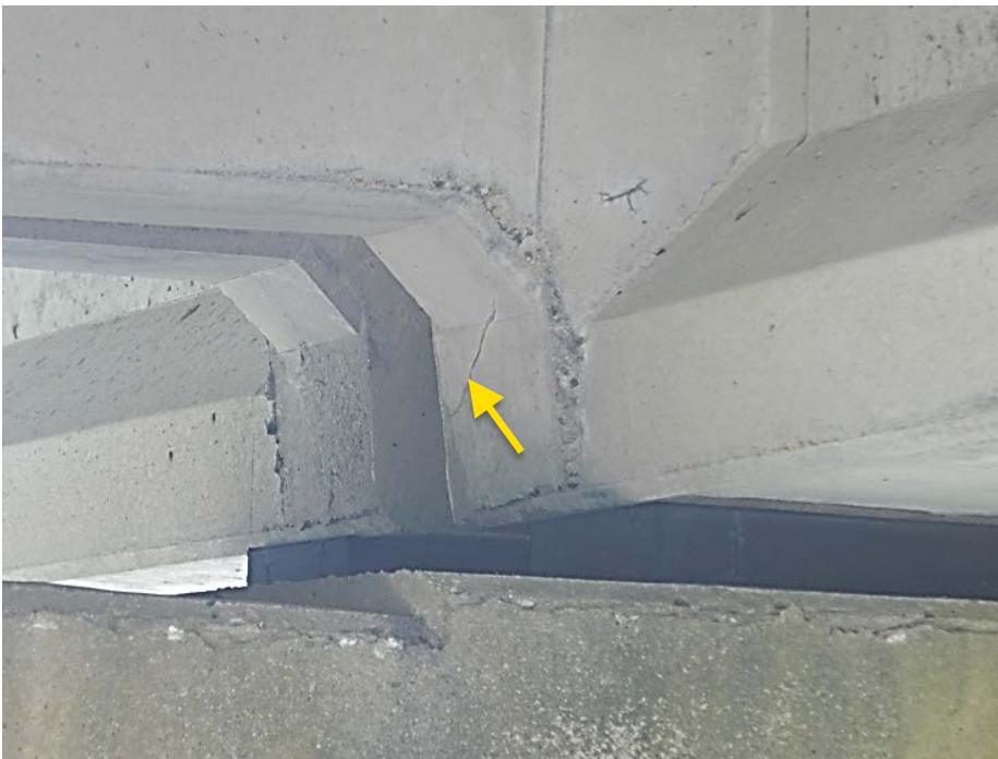
Photo 8.2-2: ASB95 Girder 5 – End Cracking at Bearing (Looking Southwest)
