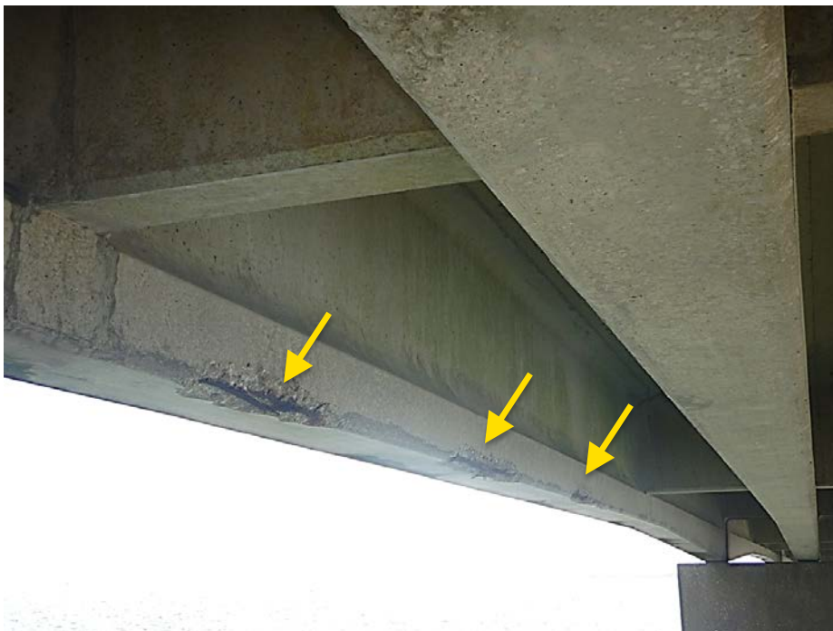
Photo 8.3-6: BNB107 Girder 8 - Spall with 1 Exposed Prestressing Strand, 3 Locations (Looking Southeast)
