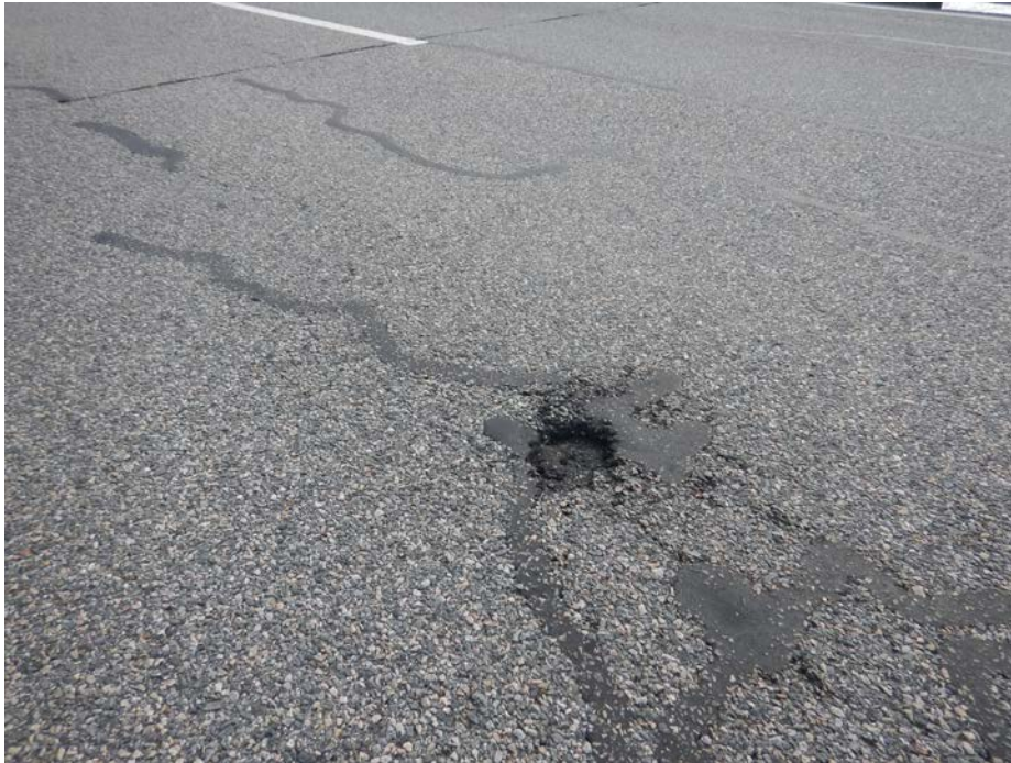
Photo 8.5-7: CNB156 Asphalt Wearing Surface – Surface Spalling (Looking Northeast)
