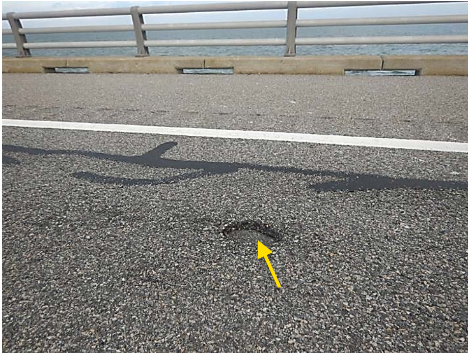
Photo 8.6-5: CSB120 Asphalt Wearing Surface – Surface Spall in Right Lane (Looking West)
