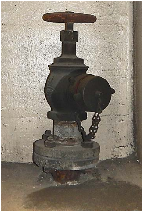
Photo 8.14-12: Hose Valve #31 at STA 513+69 - Corrosion at Concrete Interface
