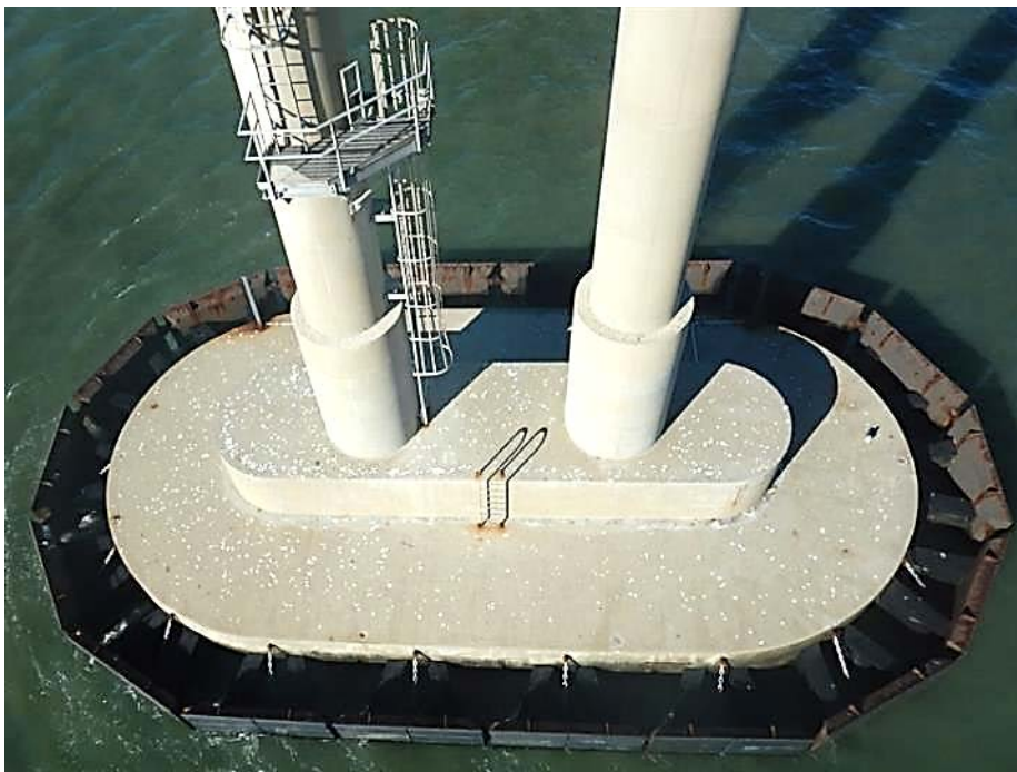
Photo 8.8-14: NCB-SB Pier 10 Reinforced Concrete Pile Cap/Footing and Columns - Minor Cracking with Efflorescence/Rust Staining (Looking South)
