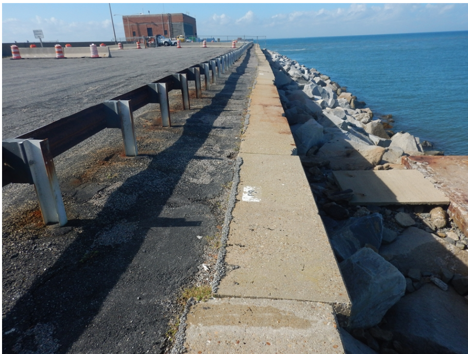
Photo 8.15-32: Portal Island 4 – Splash Walls Rotated Outward with Spalling (Looking South from Splash Wall 60)
