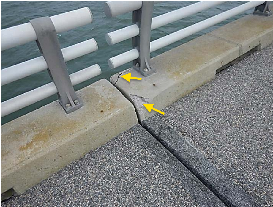
Photo 8.6-3: CSB152 Metal Bridge Railing – Failed Curb Repair (Looking Northwest)
