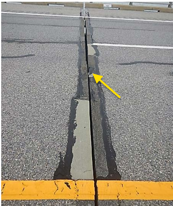
Photo 8.6-6: CSB125 Open Joint – Area of Degradation in Header (Looking West)
