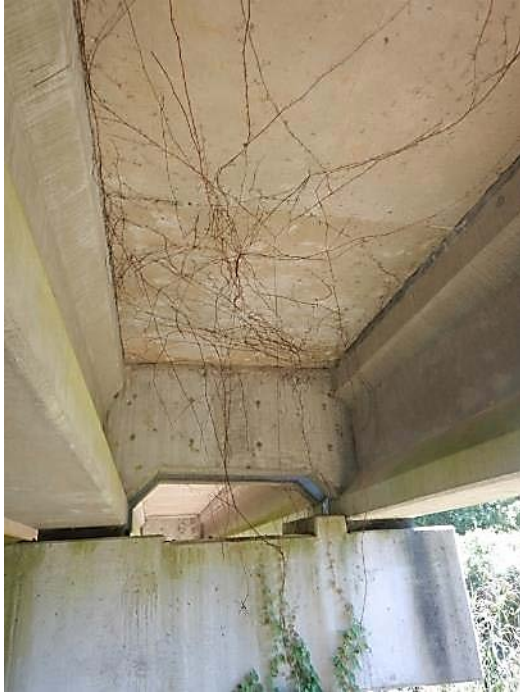
Photo 8.10-3: DSB18 Bay 4 – Vegetation on Pile Cap, Diaphragm, Girders, and Deck Underside (Looking North)
