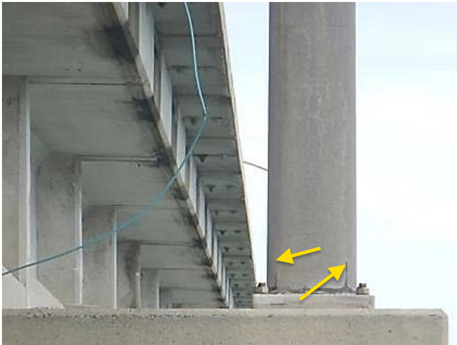
Photo 8.6-14: CSB129 Light Pole – Vertical Cracking Near Baseplate (Looking North)
