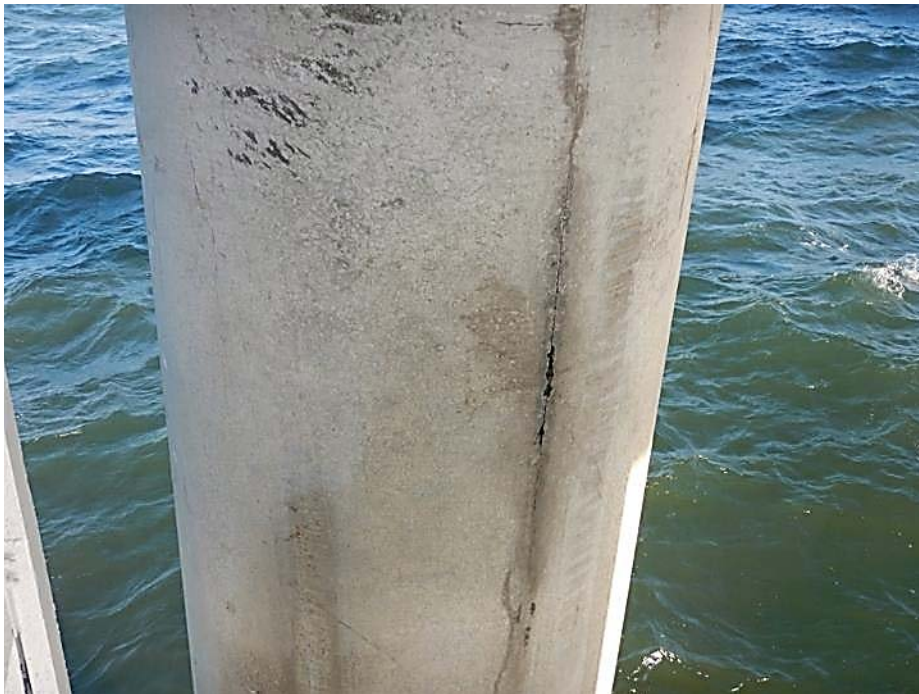
Photo 8.4-4: BSB 104 Pile A - Wide Crack/Minor Spalling along Seam (Looking Northwest)
