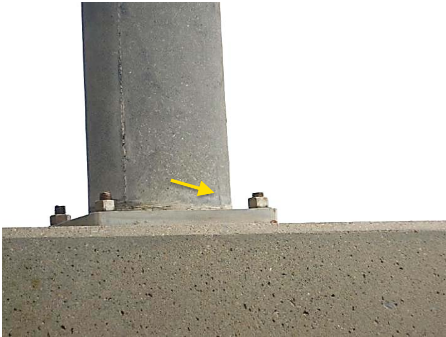
Photo 8.6-17: CSB141 Light Pole – Vertical Cracking Near Baseplate (Looking Northeast)
