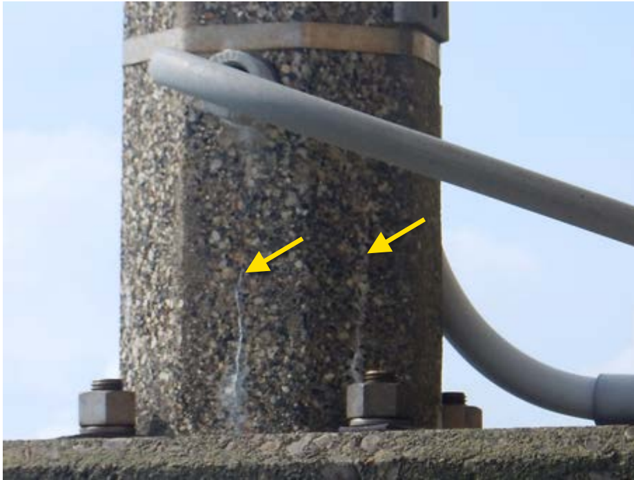
Photo 8.5-27: CNB165 Light Pole – Cracking at Baseplate with Efflorescence (Looking Southeast)
