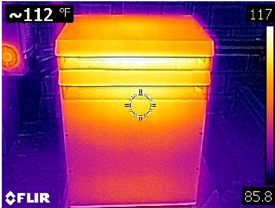
Photo 8.14-35: Electrical Distribution System - Thermal Image of Portal Island #3 CBE-3
