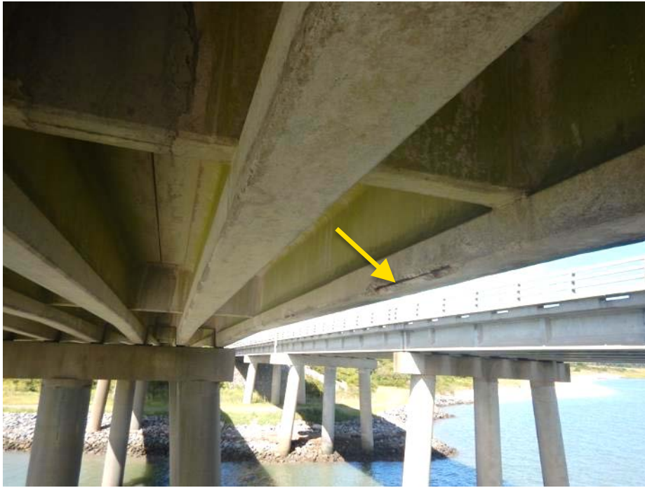
Photo 8.12-11: FSB4 Girder 8 - Failed Repair in Zone 2 with 1 Exposed Prestressing Strands (Looking Northeast)
