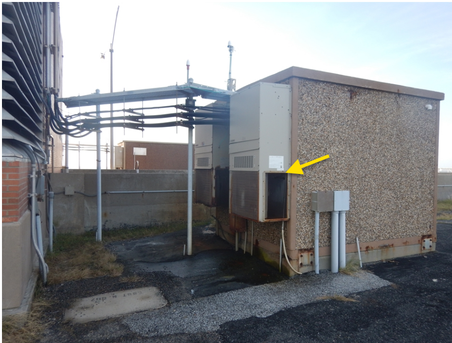
Photo 8.15-8: Portal Island 3 Utility Structure – Corroded Enclosures on Air Handling Unit (Looking East)
