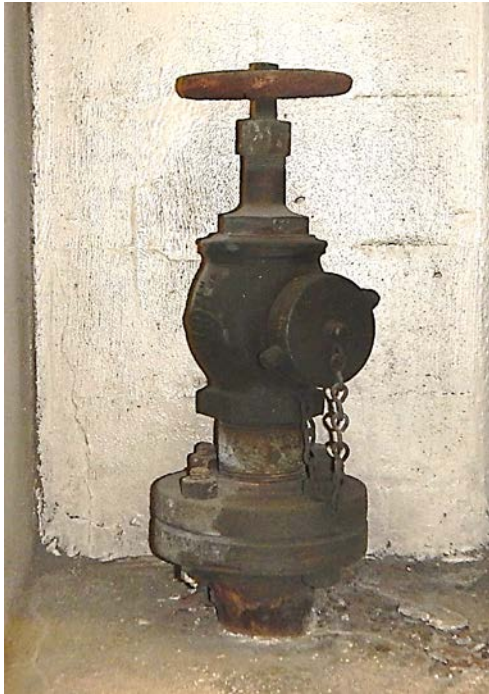
Photo 8.14-13: Hose Valve #32 at STA 515+15 - Corrosion at Concrete Interface
