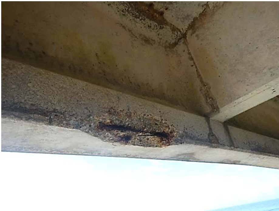
Photo 8.9-8: DNB7 Girder 1 – Spall with 1 Exposed Prestressing Strand (Looking Southeast)
