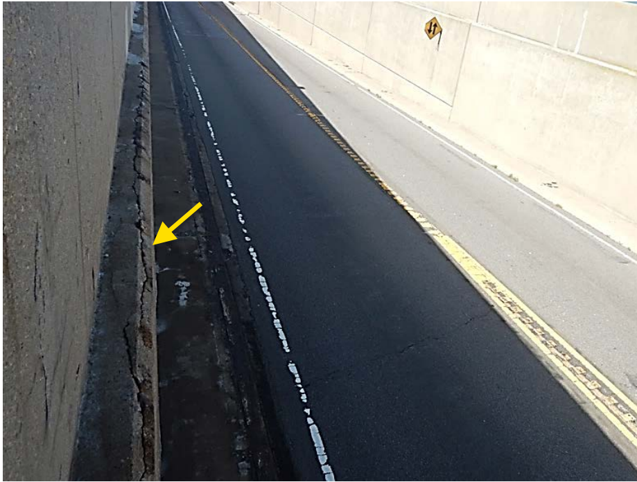
Photo 8.15-21: Portal Island 4 – Cracking/Delamination on East Approach Wall Approximately 150' from North (Looking South)
