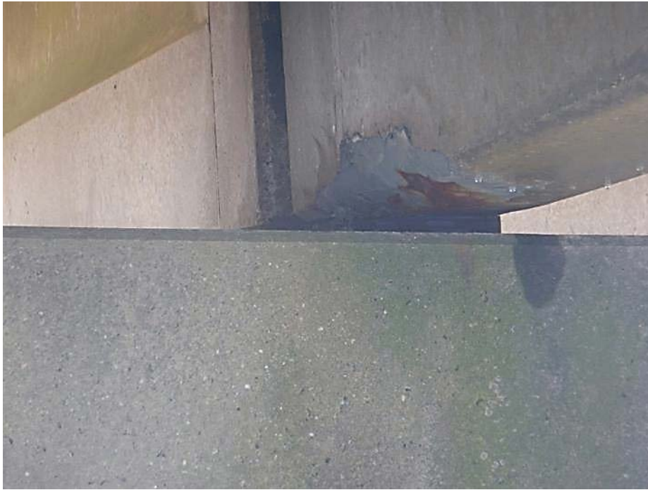
Photo 8.9-7: DNB5 Girder 5 – Failed Repair at Bearing (Looking Northeast)
