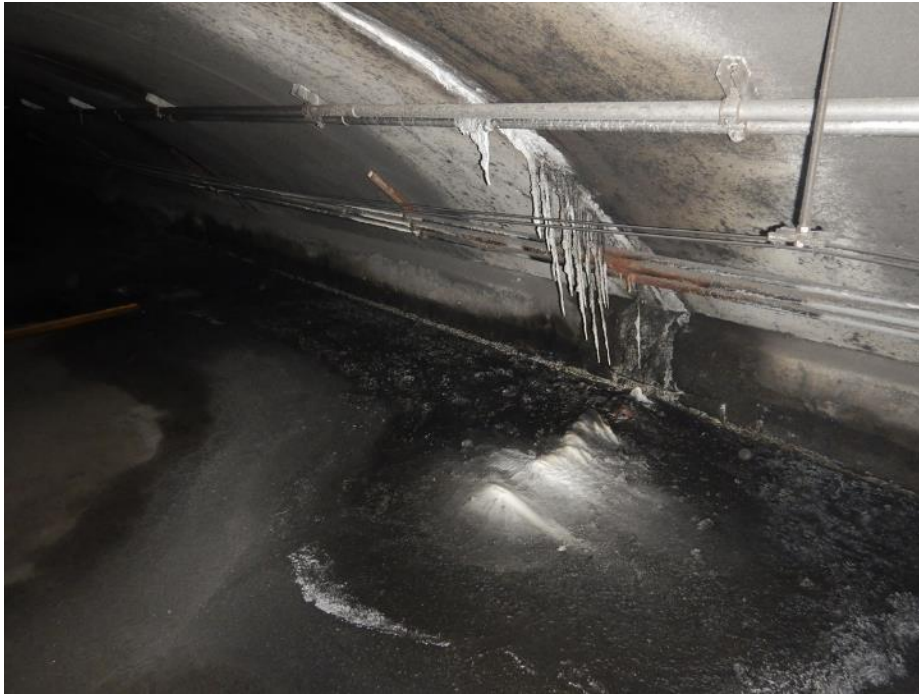
Photo 8.14-23: Exhaust Duct at STA 502+50 - Crack in Tunnel Liner with Active Heavy Efflorescence (Looking Southwest)
