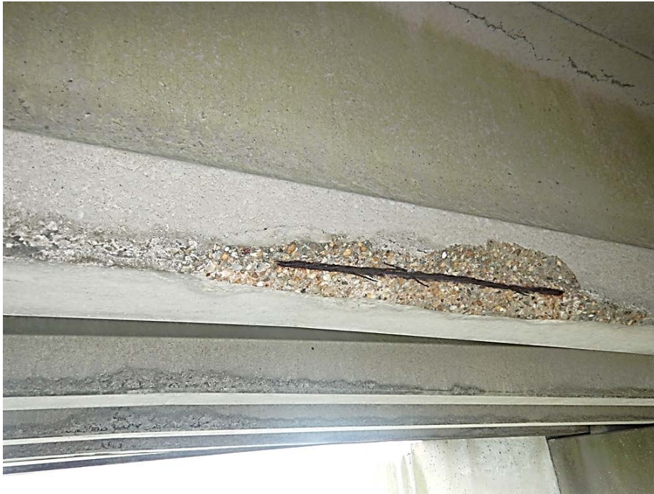
Photo 8.1-9: ANB159 Girder 6 - Spall with 1 Exposed Prestressing Strand (Looking Southeast)
