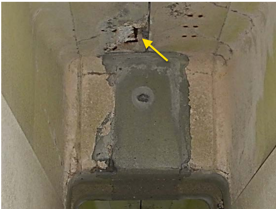
Photo 8.1-4: ANB142 Reinforced Concrete Top Flange (Underside) - Spall with Exposed Reinforcing in Bay 3 Zone 3 (Looking North)
