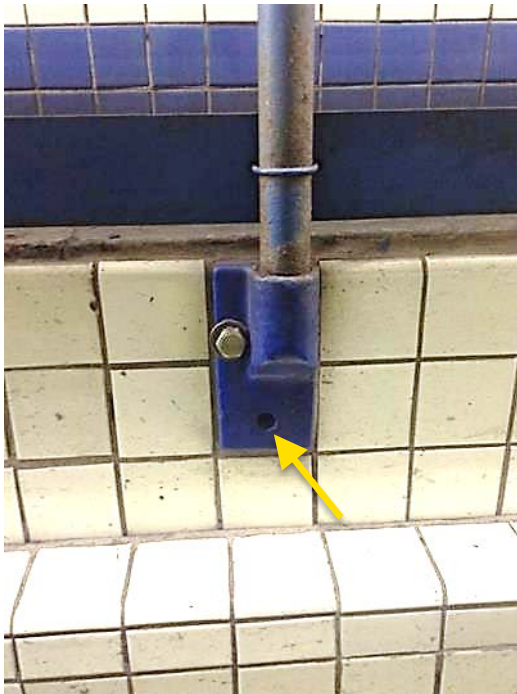
Photo 8.14-6: Steel Pedestrian Railing at STA 486+18 - Anchor Bolt Missing
