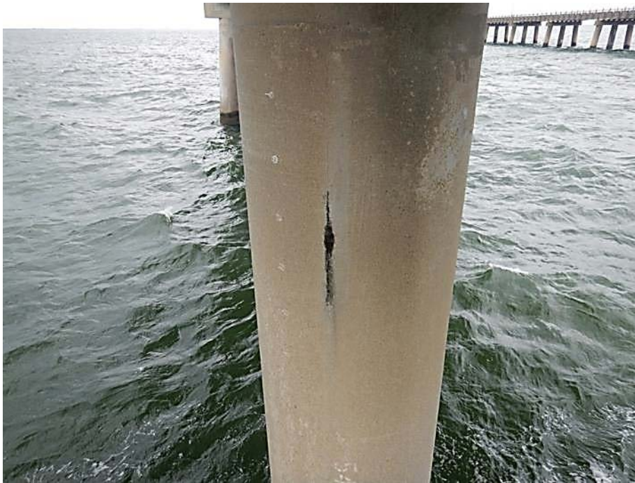
Photo 8.4-5: BSB 111 Pile B - Wide Crack/Minor Spalling along Seam (Looking North)
