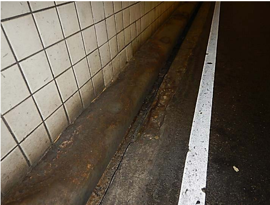
Photo 8.14-2: Invert Slab at STA 473+20 - Spall at Roadway Edge with Exposed Reinforcement
