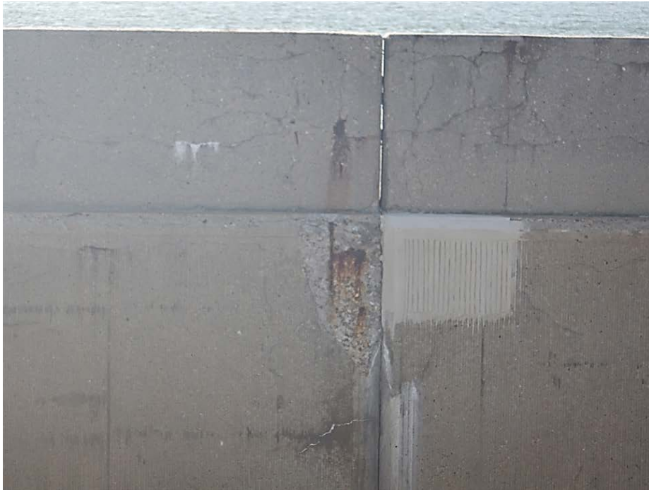
Photo 8.15-13: Portal Island 3 – Spalling with Exposed Reinforcement on East Approach Wall Approximately 100' from South (Looking East)
