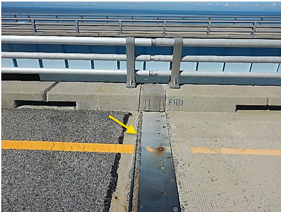
Photo 8.11-2: FIB1 Assembly Joint without Seal - Sliding Plate Expansion Joint Loose Debris Present in Joint (Looking West)
