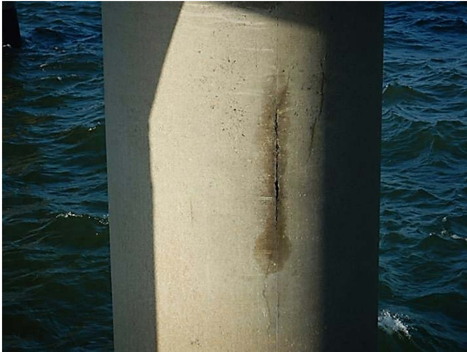
Photo 8.4-3: BSB 103 Pile B - Wide Crack/Minor Spalling along Seam (Looking Southwest)
