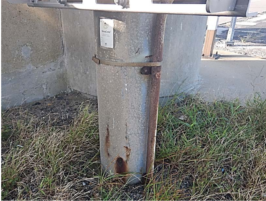
Photo 8.15-17: Portal Island 3 – Southwest Light Pole Cracking at Base (Looking Northeast)
