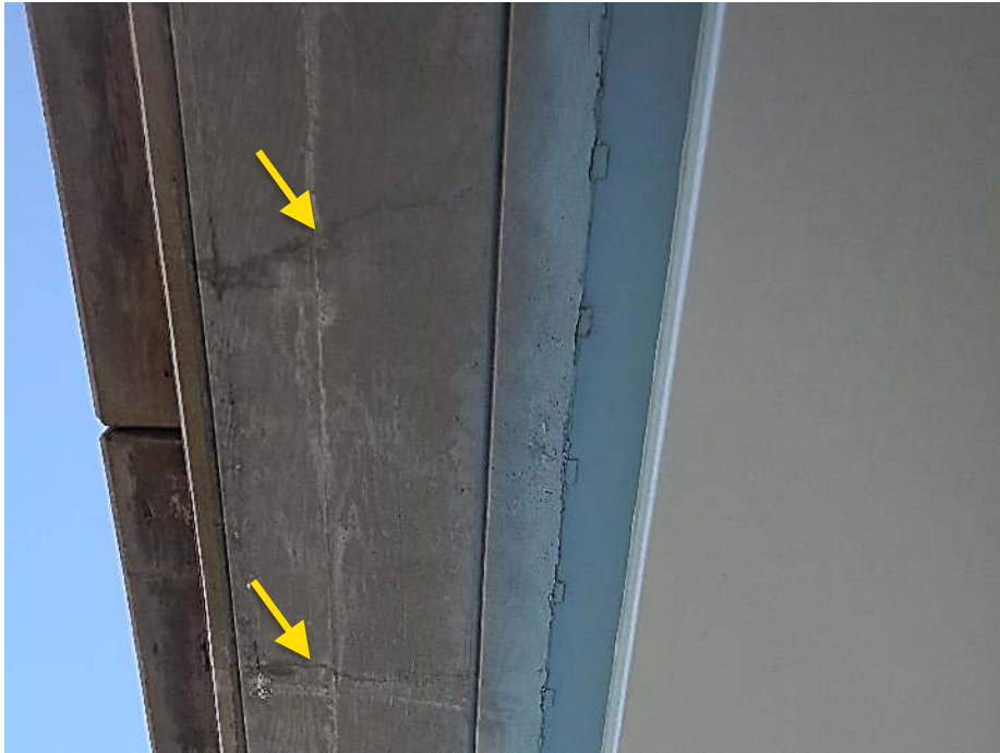
Photo 8.11-5: FIB-NB1 Reinforced Concrete Deck – Typical Minor Cracking along Edge Spaced at About 3-feet (Looking North)
