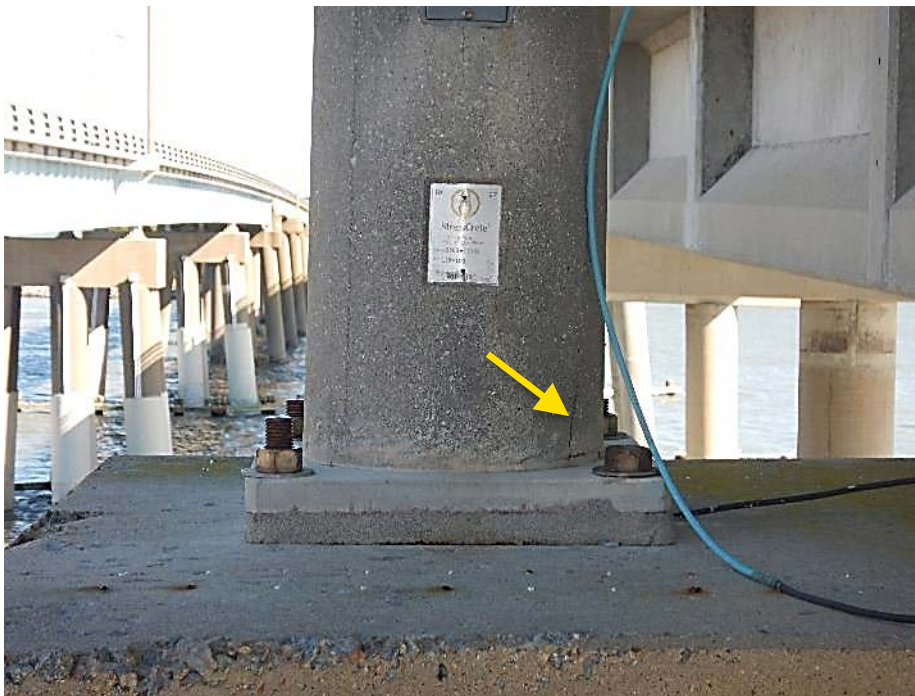
Photo 8.11-10: ENB10 Light Pole – Cracking at Baseplate (Looking North)
