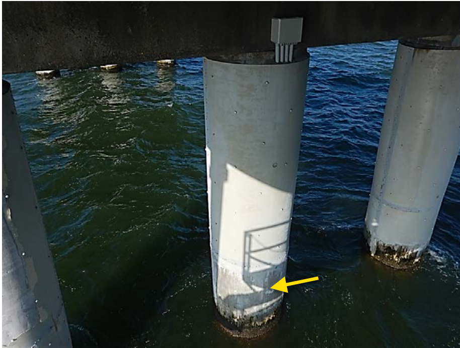
Photo 8.1-19: BNB133 Pile A - Life Jacket with Damaged Fiberglass Jacket and Slightly Exposed Zinc Mesh (Looking Northeast)
