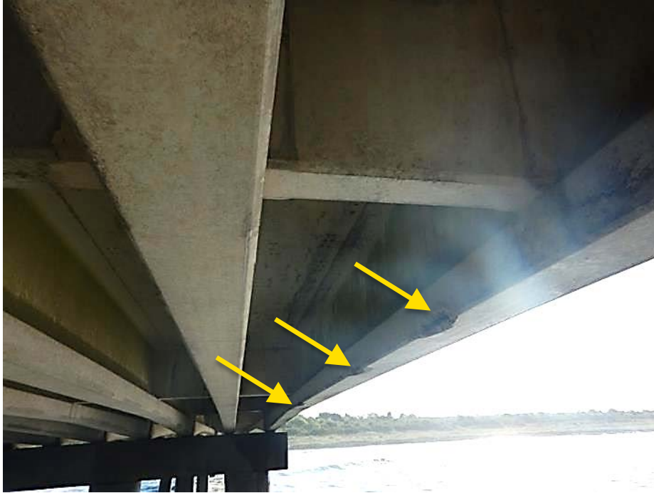
Photo 8.9-5: DNB2 Girder 1 – 3 Spall Locations with 1 Exposed Prestressing Strand (Looking Northeast)
