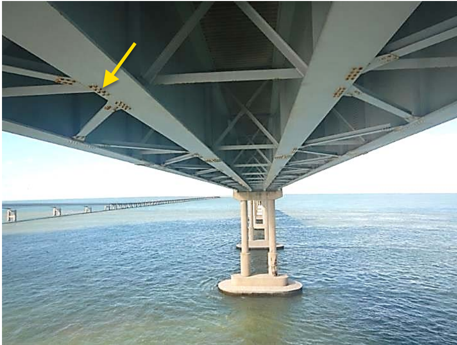
Photo 8.8-9: NCB-SB Span 8 Bracing – Typical Freckled Rust at Connections (Looking South)
