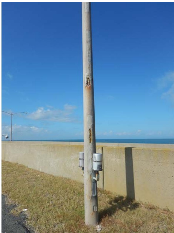
Photo 8.15-28: Portal Island 4 – 2 nd Light Pole from Northeast with Failed Repairs and Cracking extending towards the Base (Looking Southwest)
