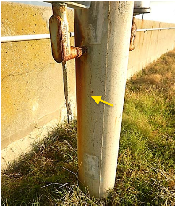
Photo 8.15-15: Portal Island 3 – 3 rd Light Pole from Southeast Cracking at Base (Looking Northeast)
