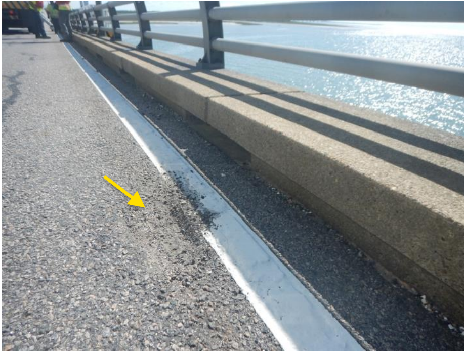
Photo 8.12-5: ESB8 Asphalt Wearing Surface - Deck Spall (Looking Southwest)
