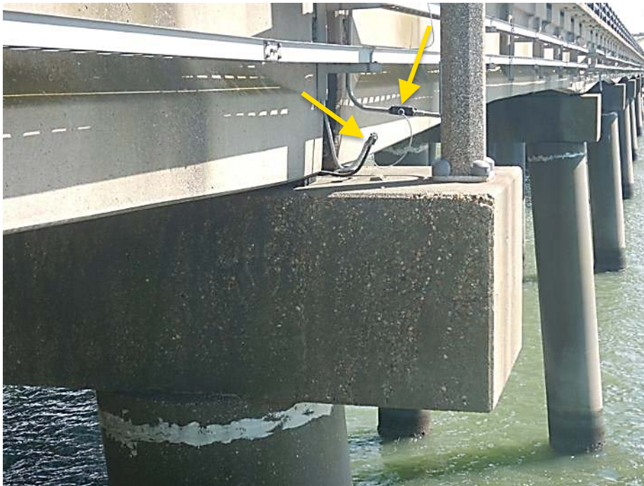
Photo 8.12-18: ESB8 Light Pole - Disconnected Cable (Looking Southeast)
