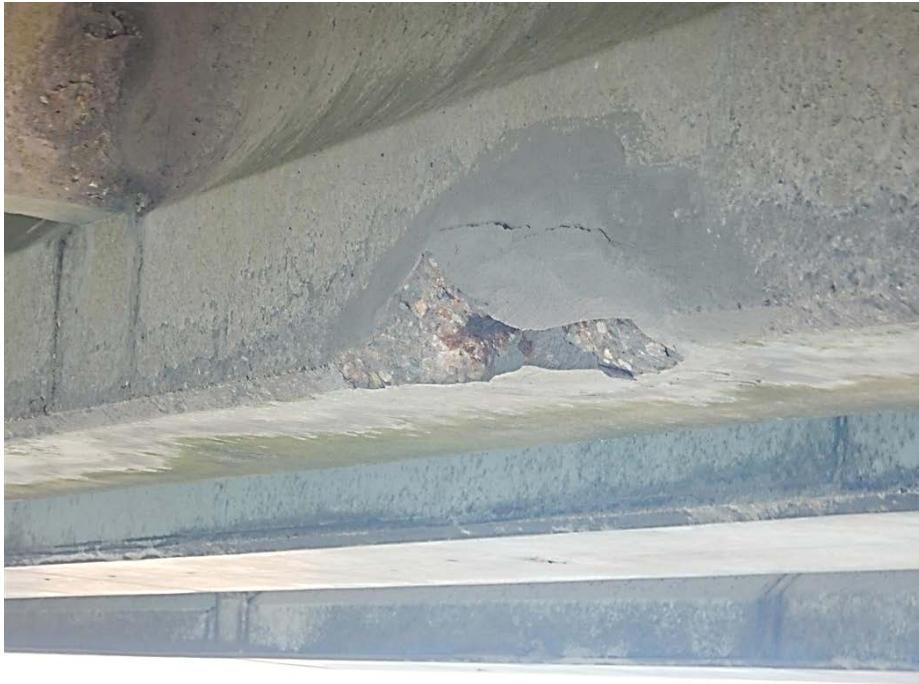
Photo 8.5-11: CNB136 Girder 3 - Repair with Exposed Prestressing Strand (Looking Northeast)
