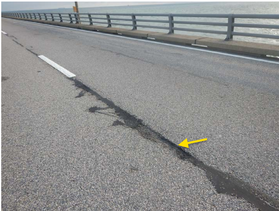
Photo 8.1-2: ANB143 Asphalt Wearing Surface – Surface Spall along Center Line (Looking Northeast)
