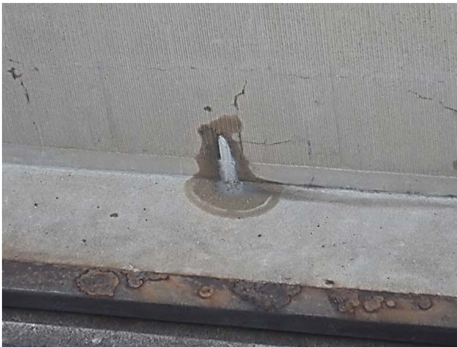
Photo 8.15-4: Portal Island 3 – Cracking with Efflorescence on West Approach Wall Approximately 700’ from South (Looking West)
