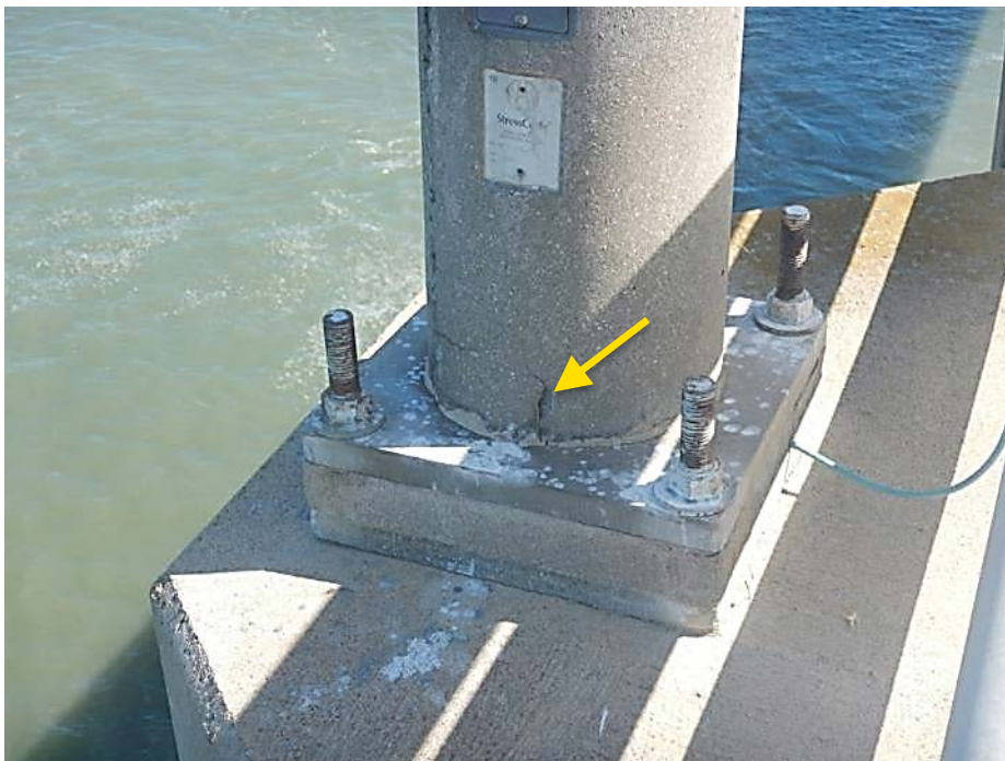
Photo 8.8-20: NCB-SB Span 6 Northwest Light Pole – Cracking and Delamination at Baseplate (Looking Northwest)
