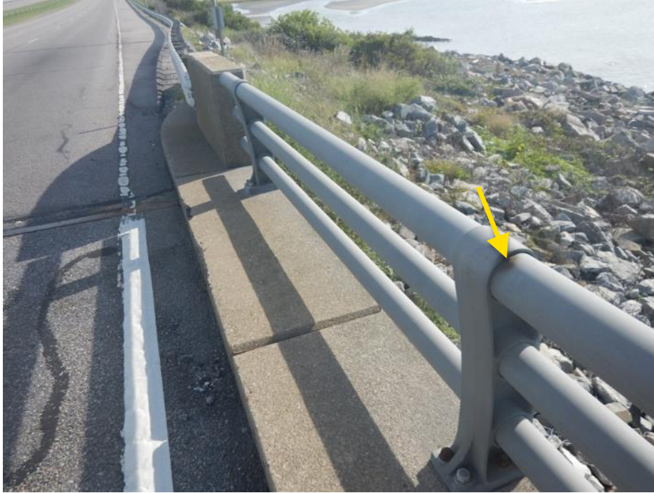
Photo 8.12-1: ESB1 Metal Bridge Railing - Corrosion on Top Rail at Post (Looking Southwest)
