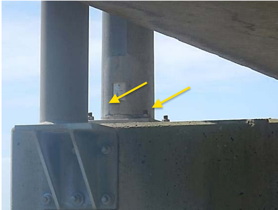
Photo 8.10-5: DSB11 Light Pole – Vertical Cracking Near Baseplate (Looking Southeast)
