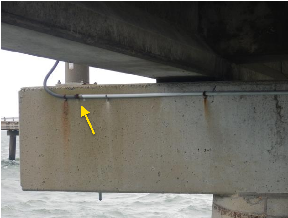
Photo 8.6-9: CSB Bent 121 - Conduit Separated (Looking South)
