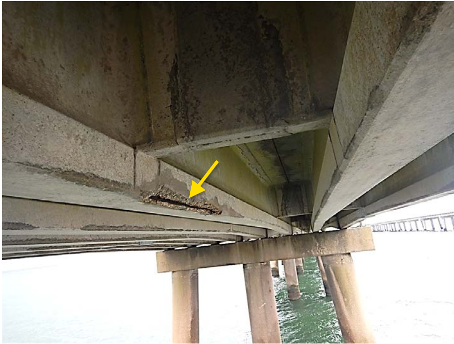
Photo 8.5-15: CNB174 Girder 6 - Failed Repair with Exposed Reinforcement Near Bearing (Looking Southeast)
