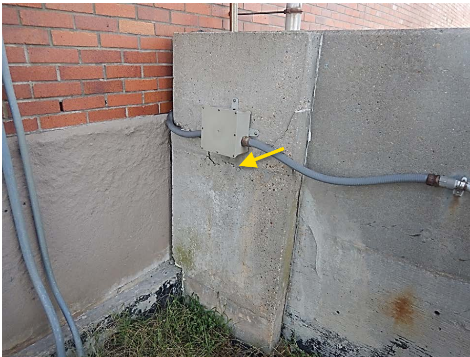
Photo 8.15-10: Portal Island 3 – Delaminated Concrete on West Approach Wall at Ventilation Building (Looking Northeast)
