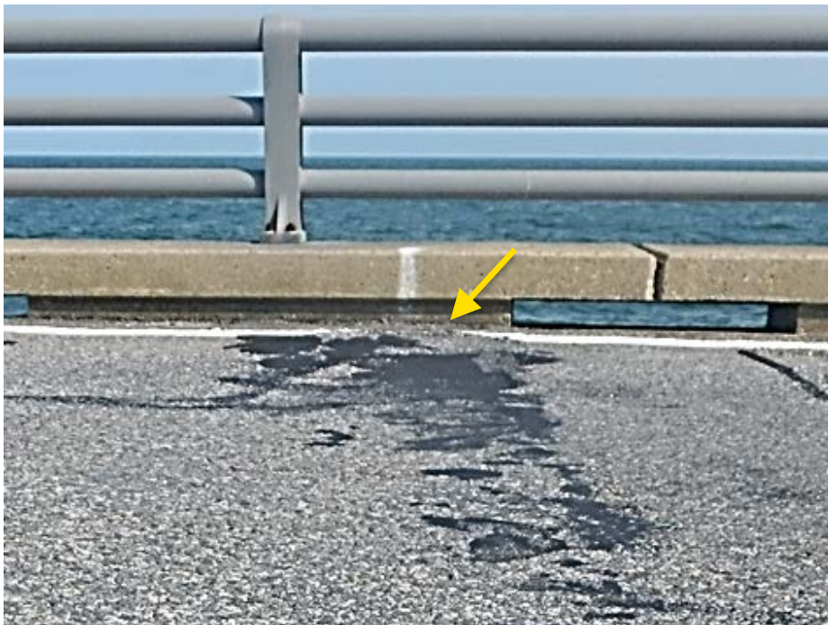
Photo 8.3-2: BNB109 Asphalt Wearing Surface – Elevated Pavement at Previous Repair in Right Lane (Looking East)
