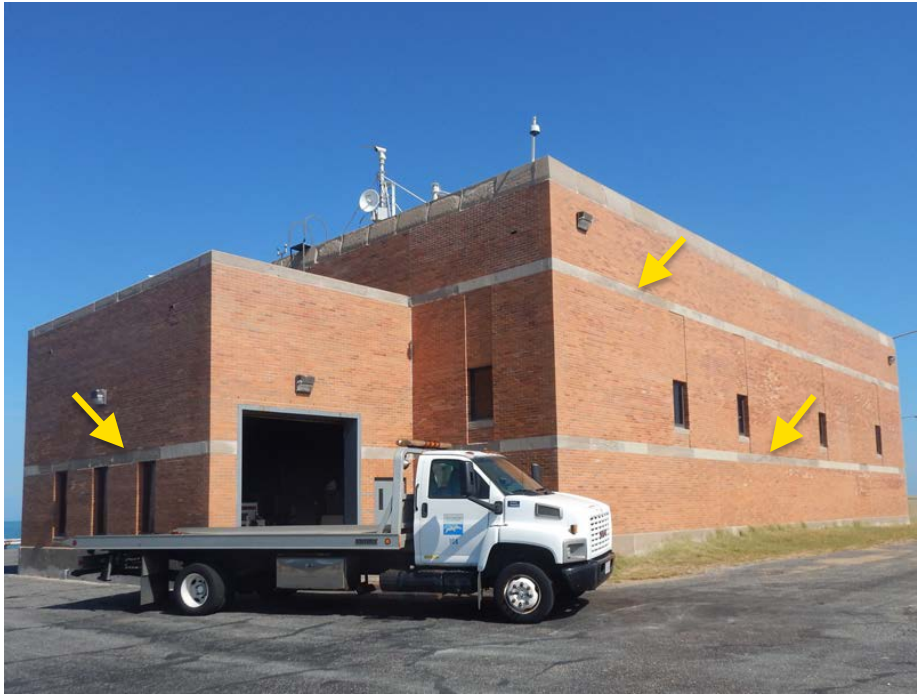
Photo 8.15-25: Portal Island 4 – Ventilation Building, Typical Erosion of Sandstone (Looking Northwest)
