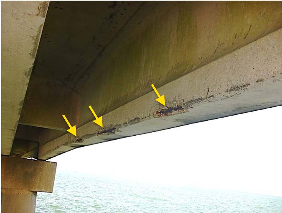
Photo 8.3-5: BNB106 Girder 1 - Spall with 1 Exposed Prestressing Strand, 3 Locations (Looking Northeast)
