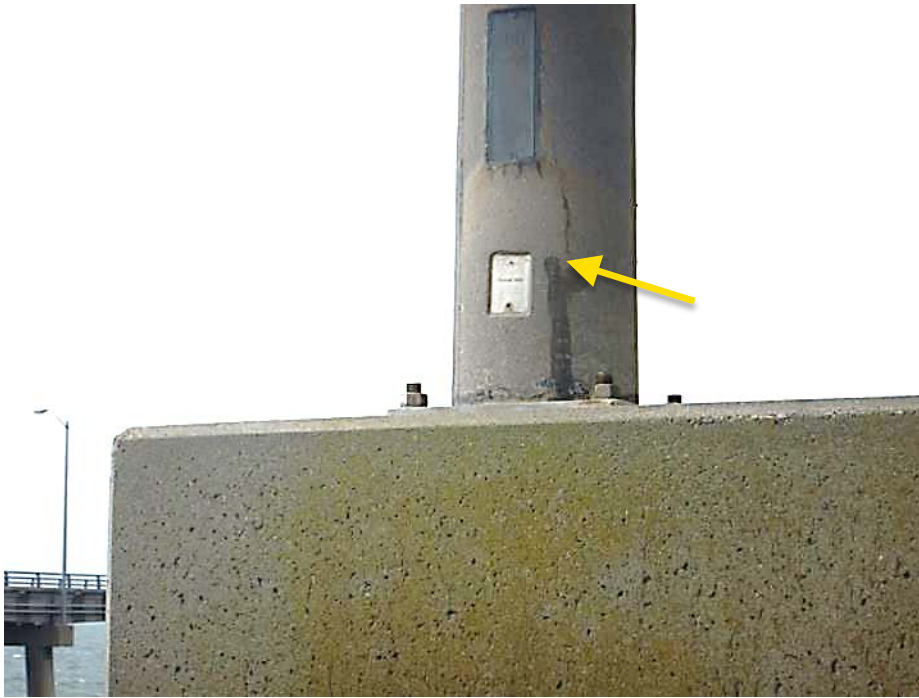
Photo 8.6-21: CSB153 Light Pole – Vertical Cracking Near Baseplate (Looking Southeast)
