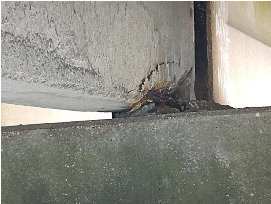
Photo 8.1-6: ANB133 Girder 3 - Spall at Bearing with 1 Exposed Reinforcement Bar (Looking Southeast)
