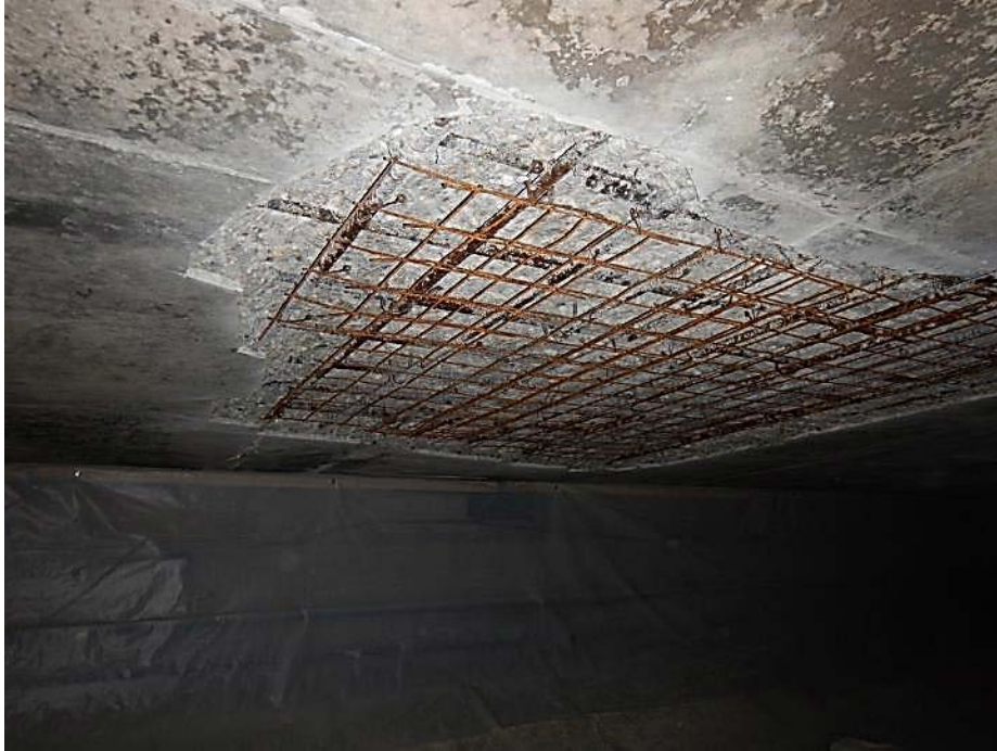
Photo 8.14-25: Invert Slab at STA 508+75 - Typical Condition of Invert Slab Prior to Shotcrete Repair (Little to No Section Loss of Existing Reinforcement)
