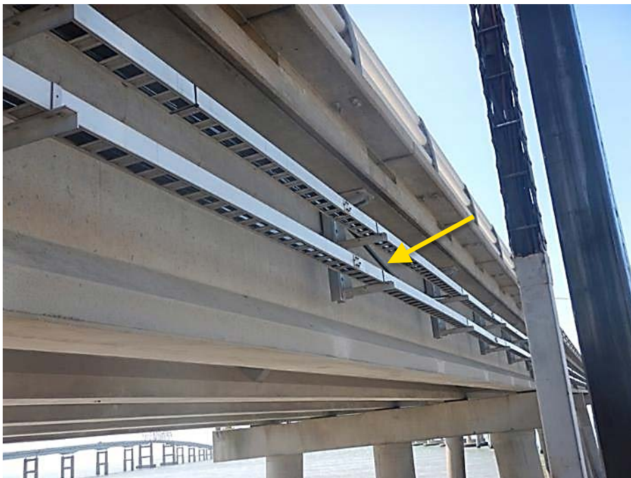
Photo 8.10-10: DSB12 Cable Tray – Cable Displaced from Tray (Looking Southeast)
