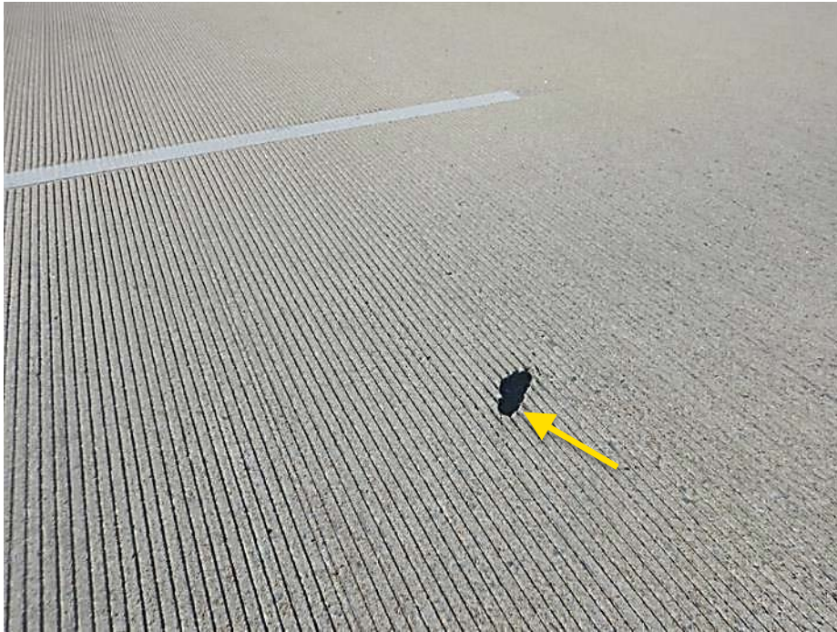
Photo 8.8-3: NCB-SB Span 10 Concrete Deck – Surface Spall, No Exposed Reinforcement (Looking Southeast)
