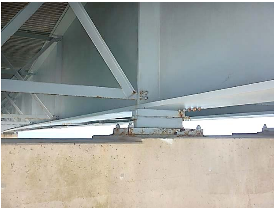
Photo 8.8-12: NCB-NB Pier 9 G2 Fixed Bearing - Typical Condition of Isolated areas of Surface Rust (Looking Southwest)
