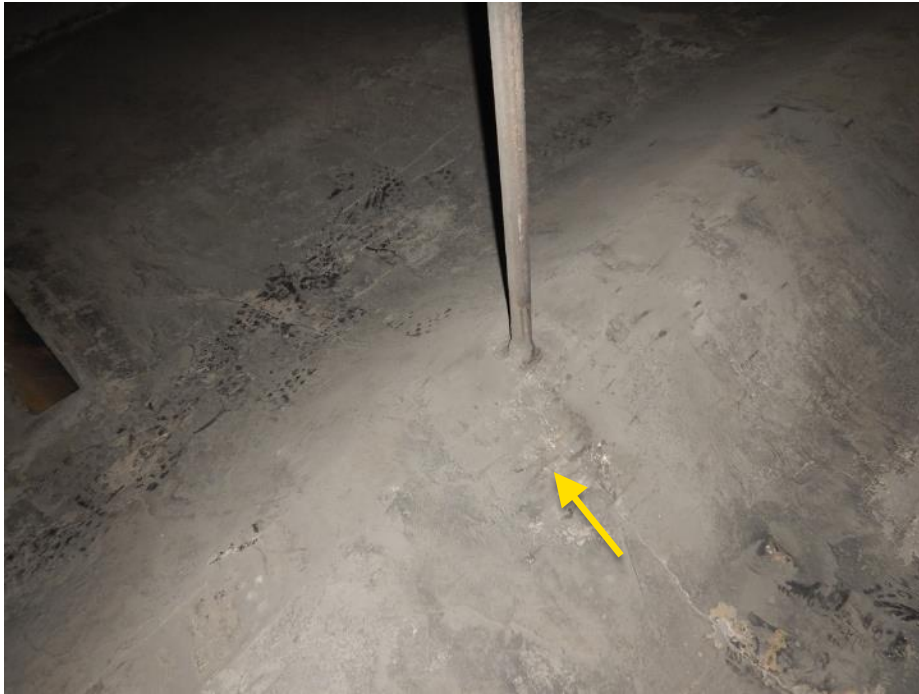
Photo 8.14-21: Ceiling Slab at STA 474+98 - Delamination in Haunch Beam Adjacent to Hanger Anchorage (Looking Northwest)
