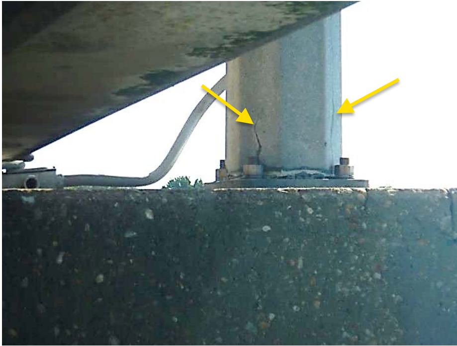
Photo 8.9-13: DNB5 Light Pole – Cracking at Baseplate (Looking Northeast)
