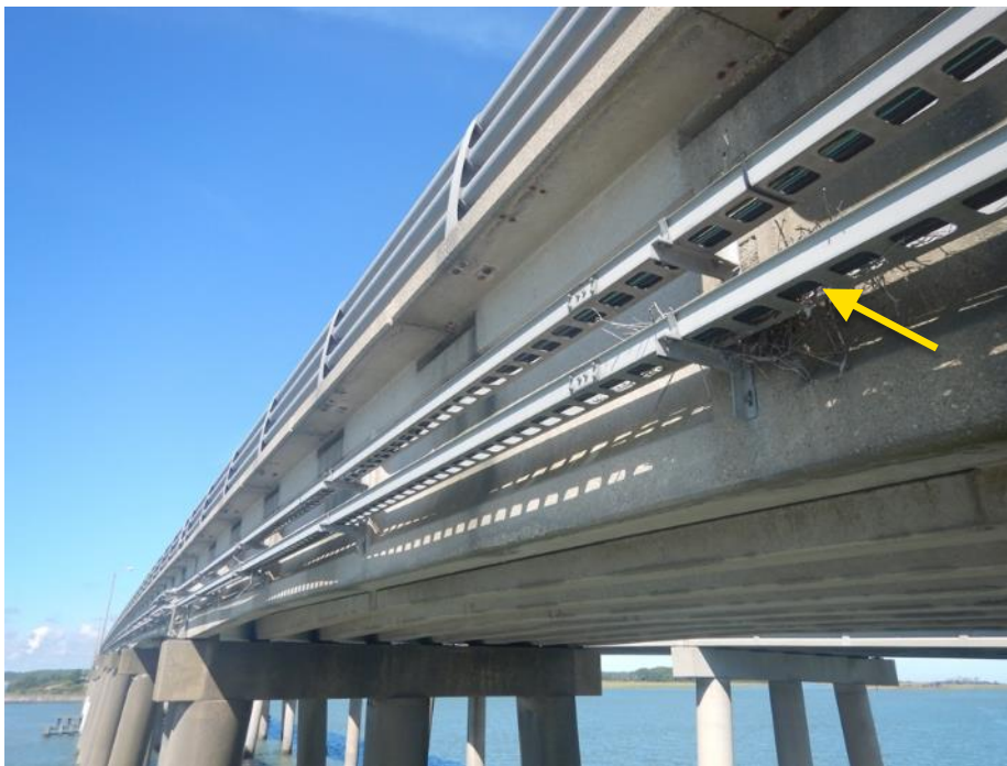
Photo 8.12-20: ESB9 Cable Tray - Debris (Looking Northeast)
