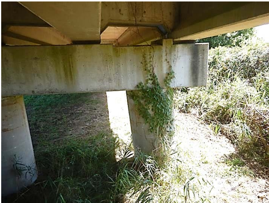
Photo 8.10-4: DSB Bent 18 Pile C – Vegetation on Pile and Pile Cap (Looking North)
