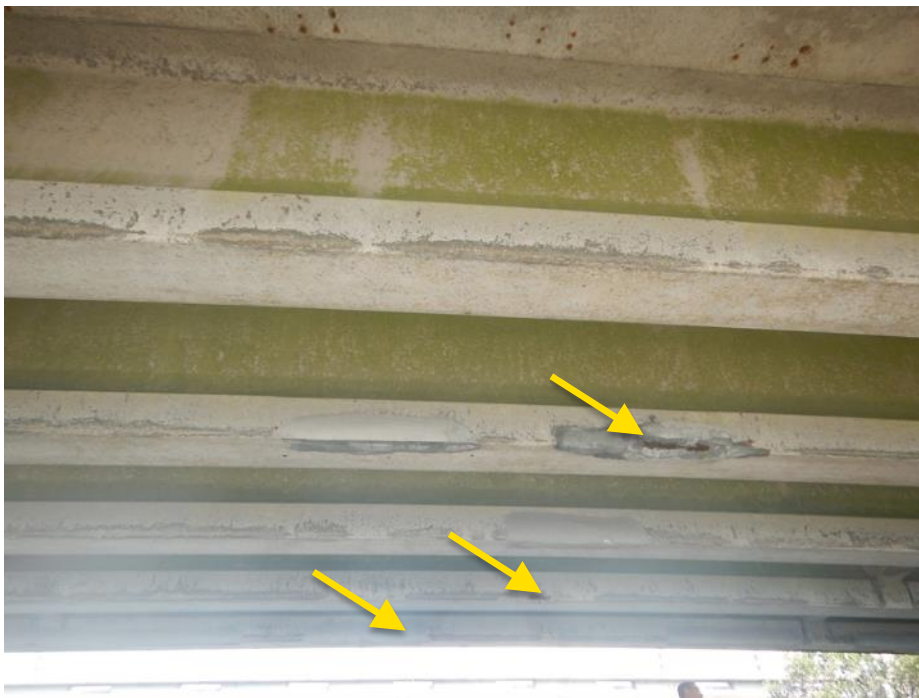
Photo 8.12-8: ESB1 Girders 5 thru 8 – Exposed Strand in Girder 5, and Cracking and Rust Staining in Repairs of Girders 7 and 8 (Looking East)
