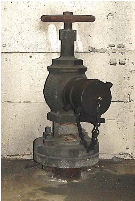
Photo 8.14-16: Hose Valve #37 at STA 522+40 - Corrosion at Concrete Interface
