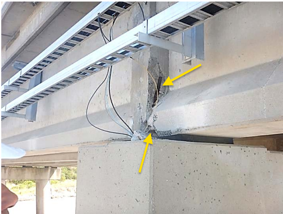
Photo 8.10-2: DSB11 Girder 1 – Spalling at Closure Diaphragm with Exposed Reinforcement and Prestressing Strand (Looking Northeast)
