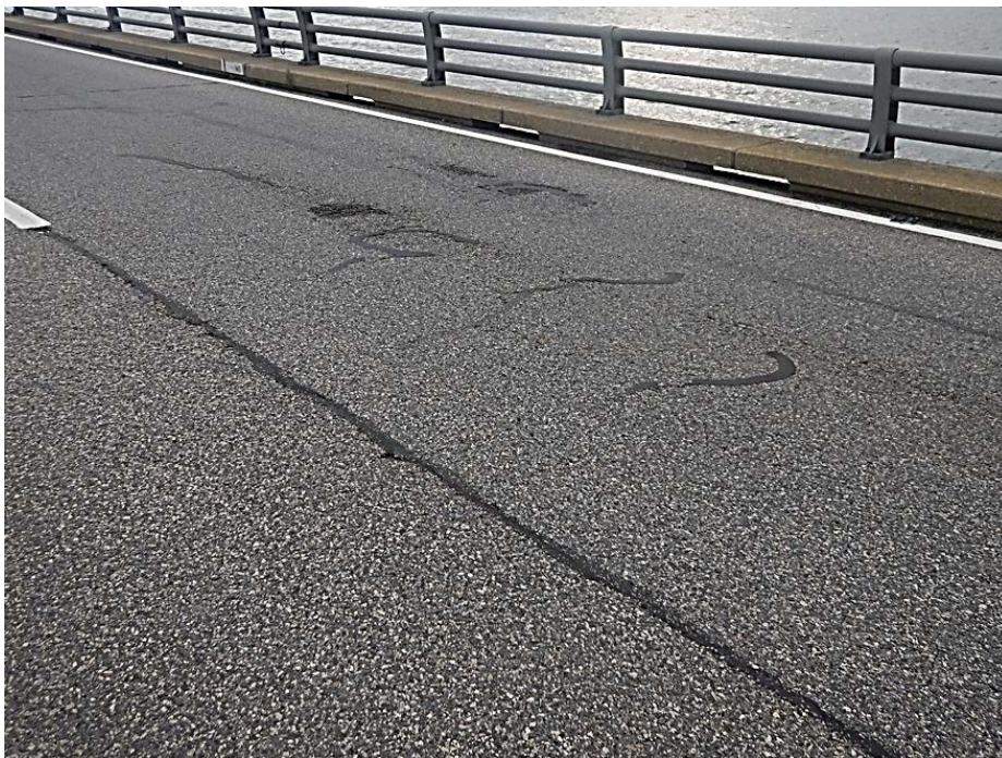
Photo 8.5-4: CNB144 Asphalt Wearing Surface – Scaling and Surface Spalling (Looking Northeast)
