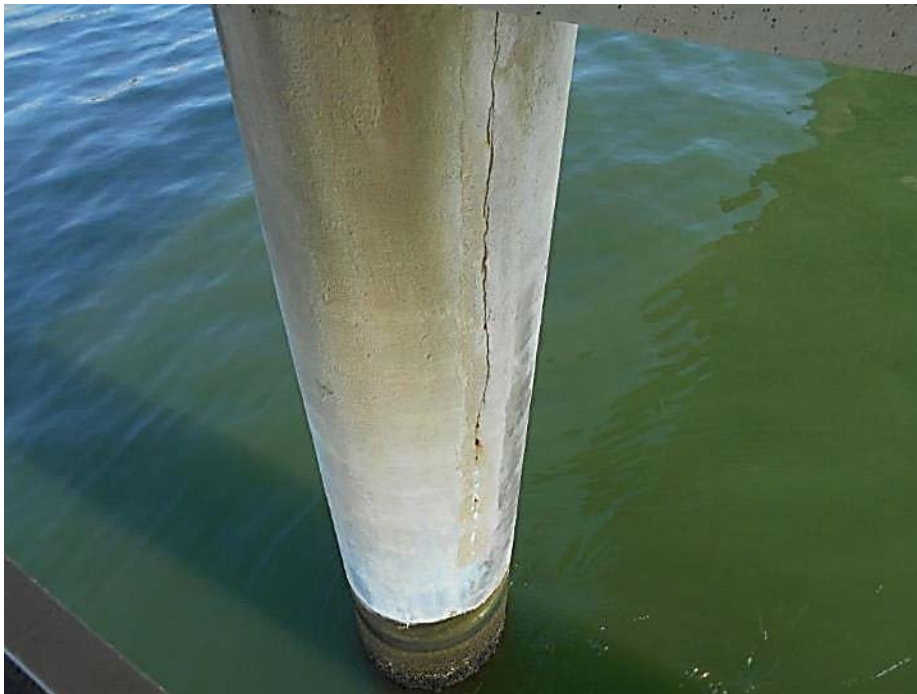
Photo 8.1-14: ANB96 Pile A - Crack through Protective Coating with Rust Staining (Looking Northeast)
