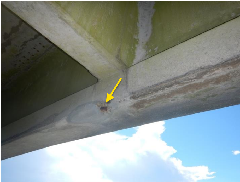
Photo 8.12-12: FSB6 Girder 1 - Failed Repair in Zone 1 with 1 Exposed Prestressing Strands (Looking Southeast)
