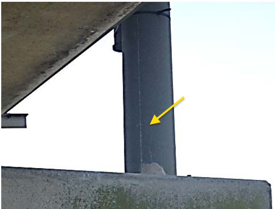
Photo 8.2-8: ASB15 Light Pole – Vertical Cracking Near Baseplate above Repair Area (Looking Southwest)
