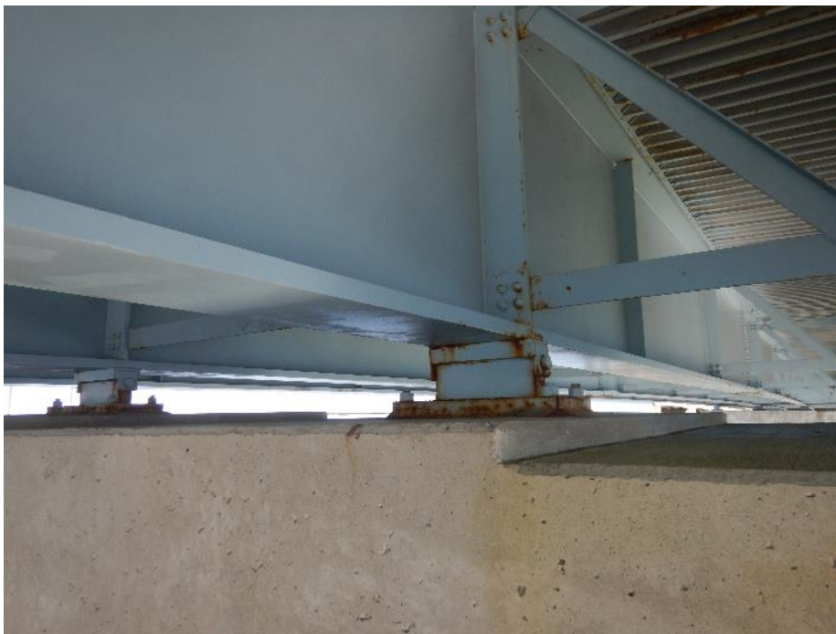
Photo 8.11-8: FIB-NB Pier 2 G2 Fixed Bearing - Typical Condition of Isolated areas of Surface Rust (Looking Northwest)
