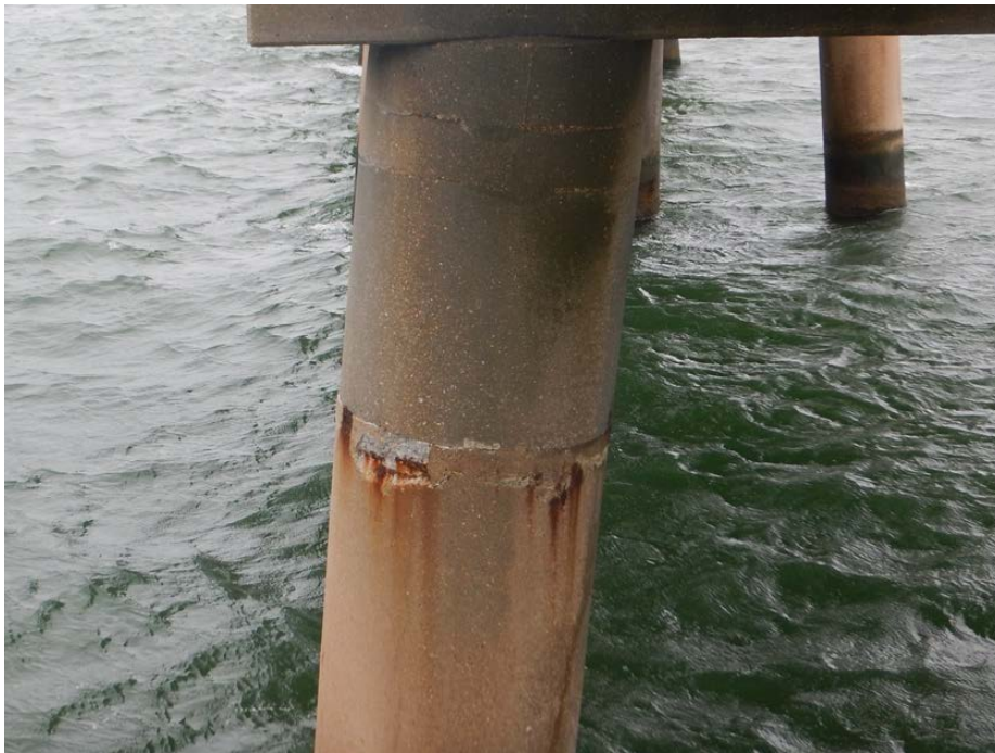
Photo 8.5-22: CNB184 Pile A - Spall with Exposed Reinforcement (Looking Northeast)
