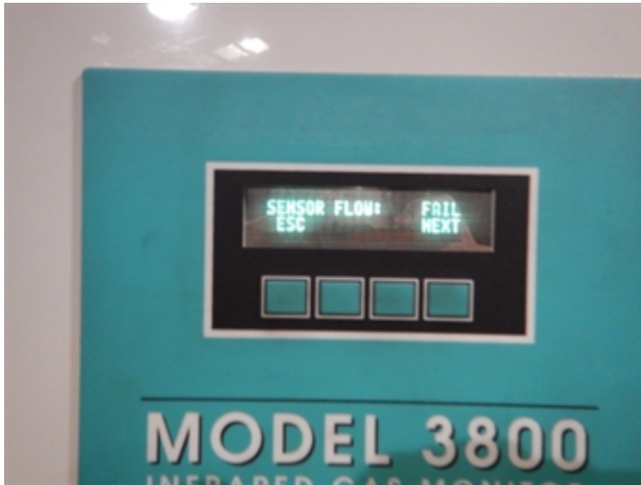
Photo 8.14-27: Ventilation System - Portal Island #4 Exhaust Duct CO Monitor Device Had an Error Reading "Sensor Flow - Fail" (Possibly Due to Moisture)
