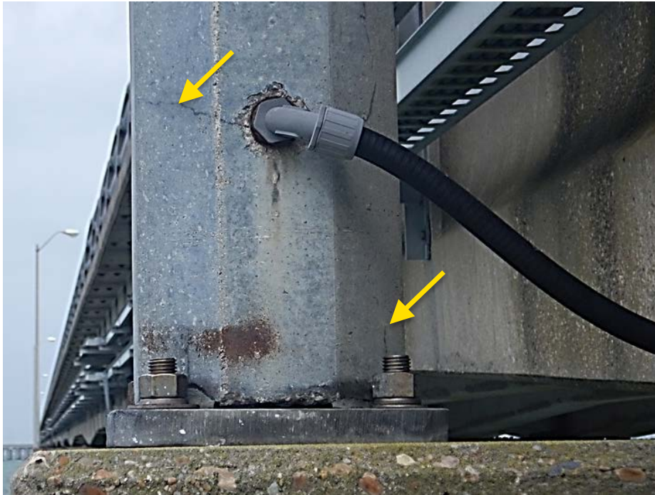
Photo 8.5-29: CNB192 Light Pole – Cracking at Baseplate (Looking Northeast)
