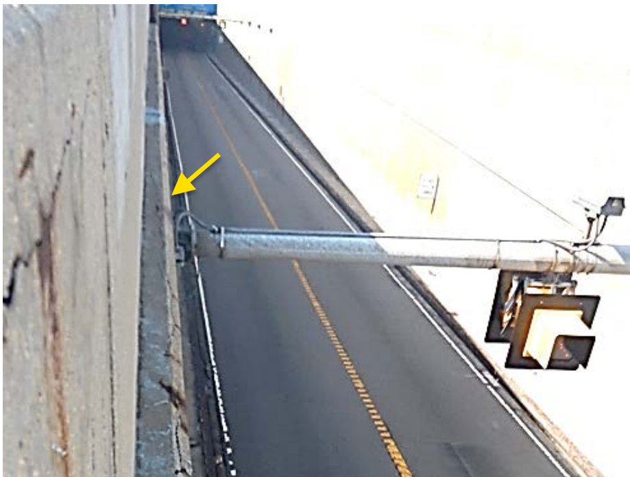
Photo 8.15-22: Portal Island 4 – Cracking/Delamination on East Approach Wall at Overhead Signal Anchorage Approximately 530' from North (Looking South)
