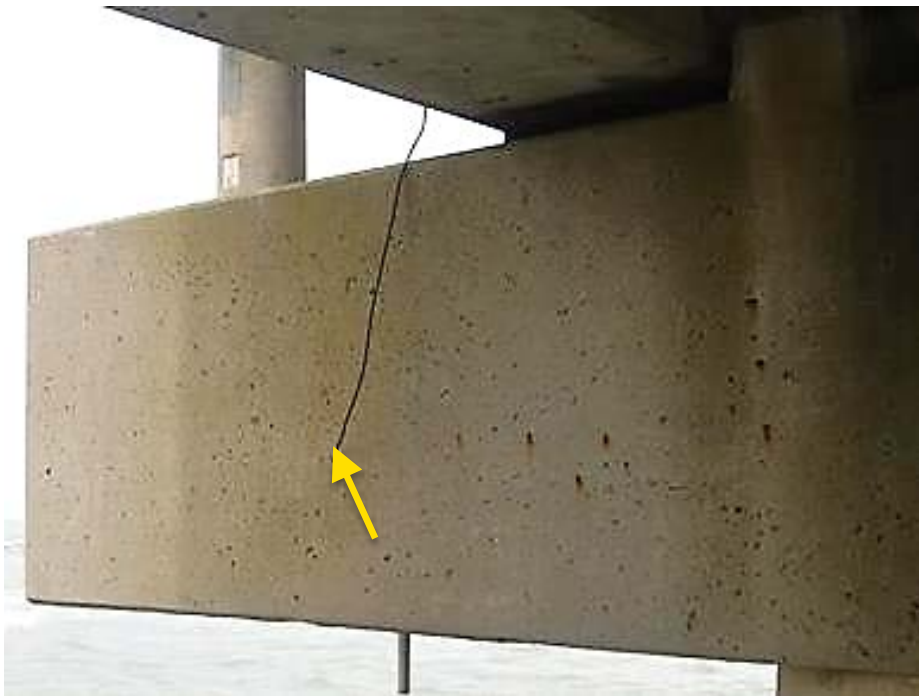
Photo 8.6-10: CSB Bent 131 - Disconnected Cable (Looking Northwest)
