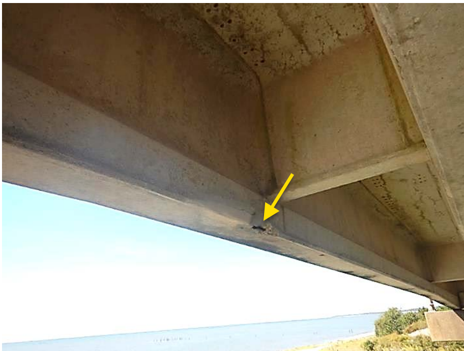
Photo 8.12-10: FSB4 Girder 1 - Failed Repair in Zone 1 with 1 Exposed Prestressing Strands (Looking Northwest)
