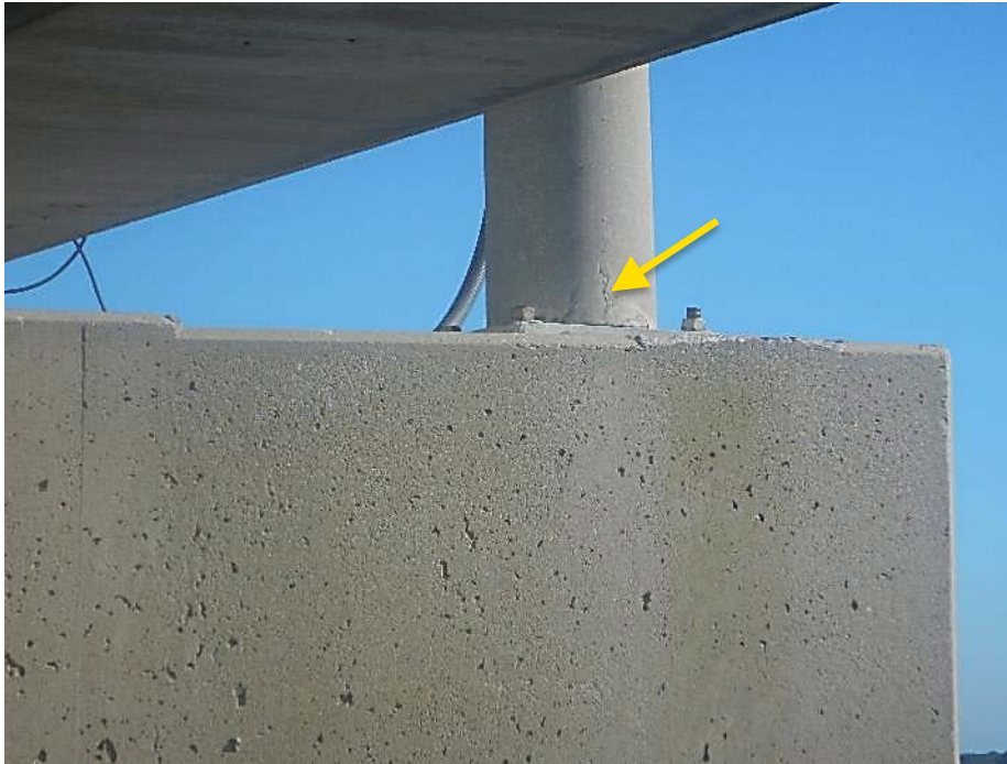
Photo 8.11-9: ENB8 Light Pole – Cracking at Baseplate (Looking Northeast)
