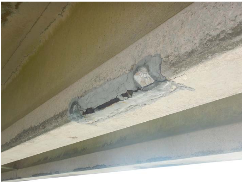
Photo 8.3-8: ANB127 Girder 2 - Failed Repair with 1 Exposed Prestressing Strand (Looking Northeast)
