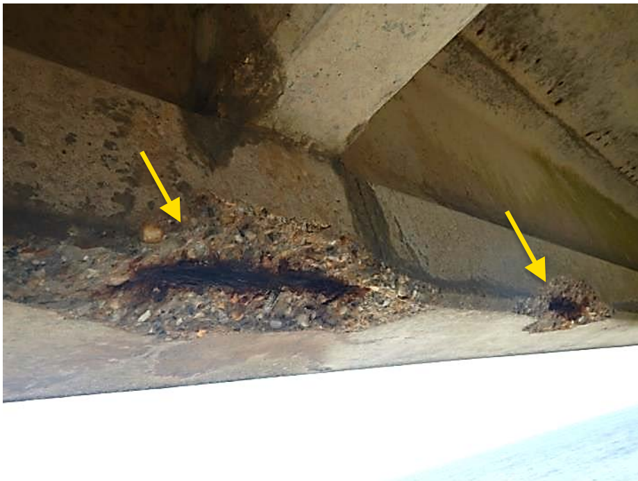
Photo 8.9-6: DNB3 Girder 3 – 2 Spall Locations with 1 Exposed Prestressing Strand (Looking Southeast)
