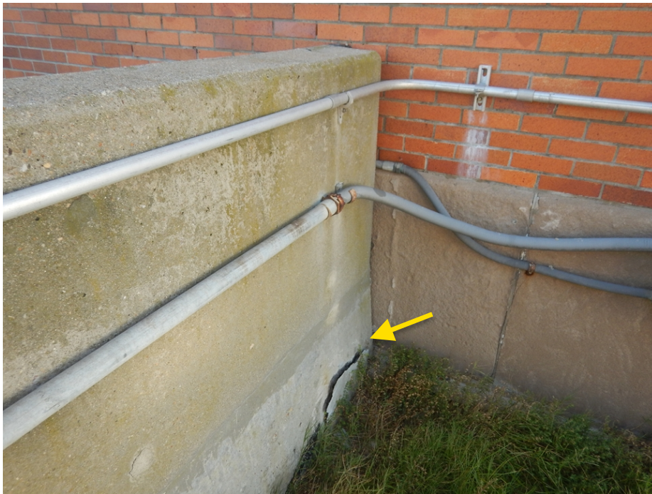
Photo 8.15-6: Portal Island 3 – Failed Concrete Repair on East Approach Wall at Ventilation Building (Looking Northwest)
