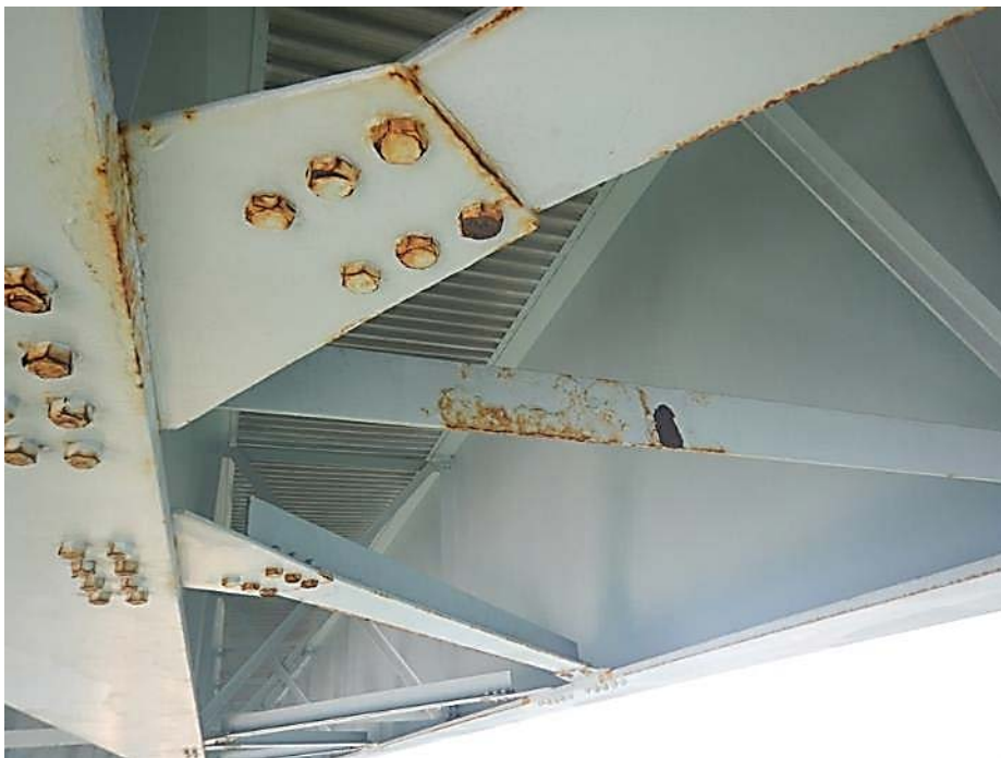
Photo 8.8-10: NCB-SB Span 8, Bay 1, Cross Frame 7 Bracing – Typical Freckled Rust at Connections and Paint Failure on Bracing (Looking Southwest)
