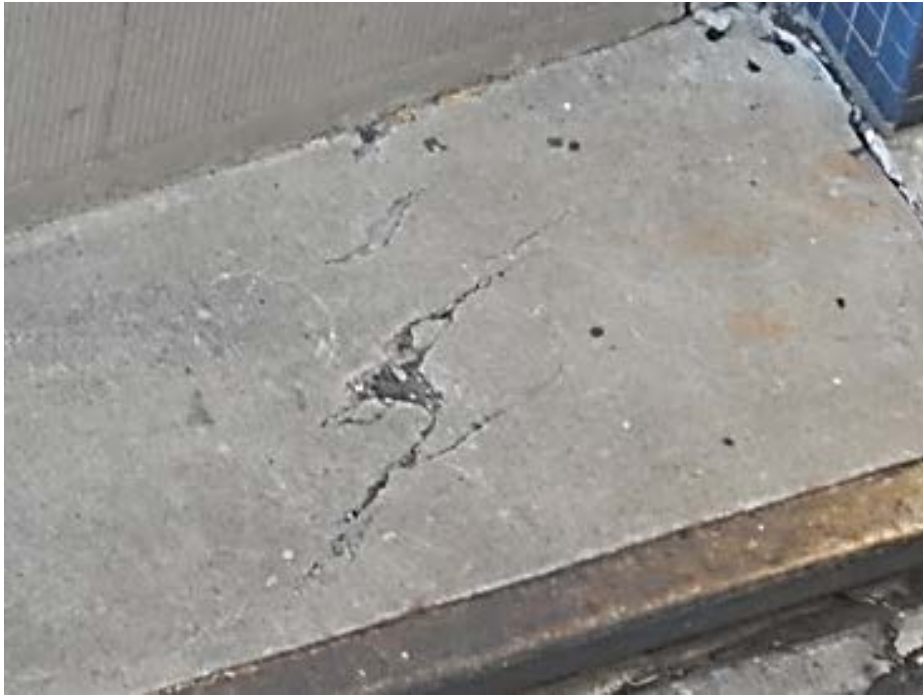
Photo 8.15-5: Portal Island 3 – Cracking/Delamination on West Sidewalk at Tunnel Portal (Looking Northwest)
