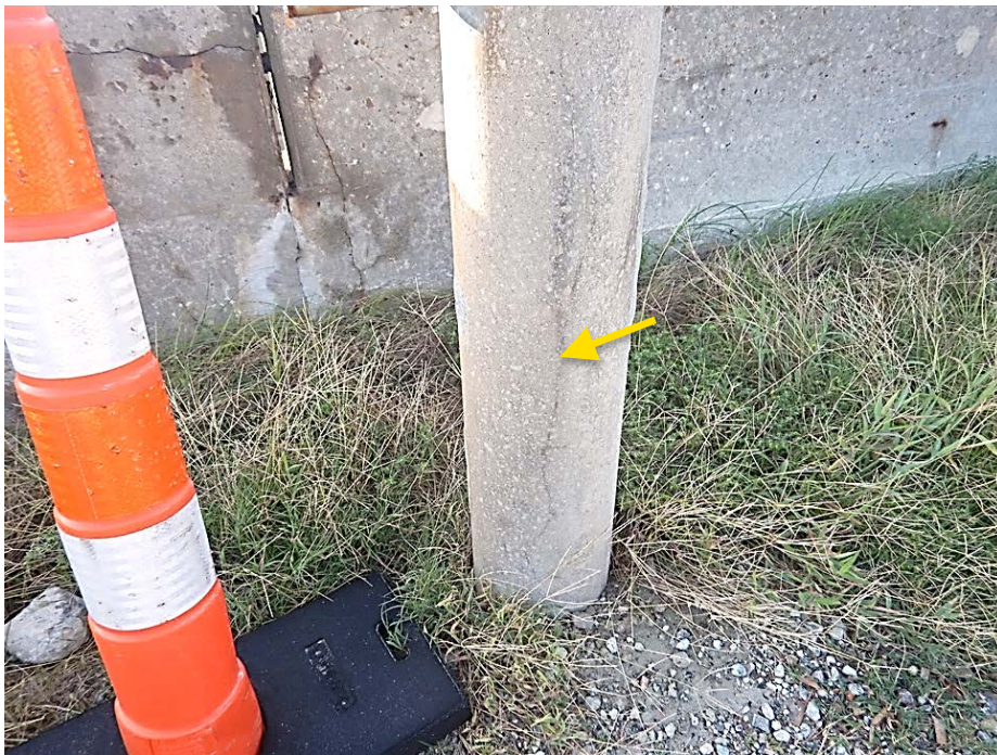
Photo 8.15-16: Portal Island 3 – 3 rd Light Pole from Southwest Cracking at Base (Looking Northeast)
