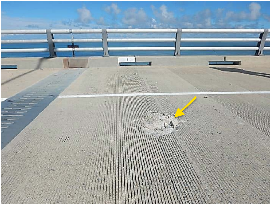
Photo 8.8-2: NCB-SB Span 8 Concrete Deck – Spall (Previously Patched), No Exposed Reinforcement (Looking West)
