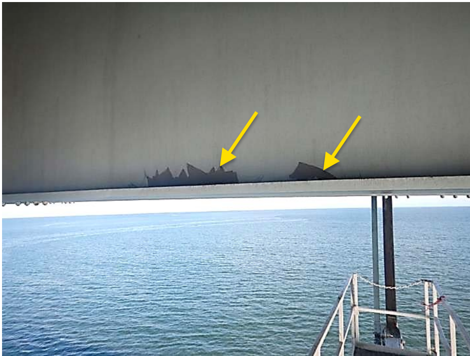
Photo 8.8-8: NCB-SB Span 12 Girder 2 – Top Protective Coating Peeled Off Exposing Zinc Primer (Looking West)
