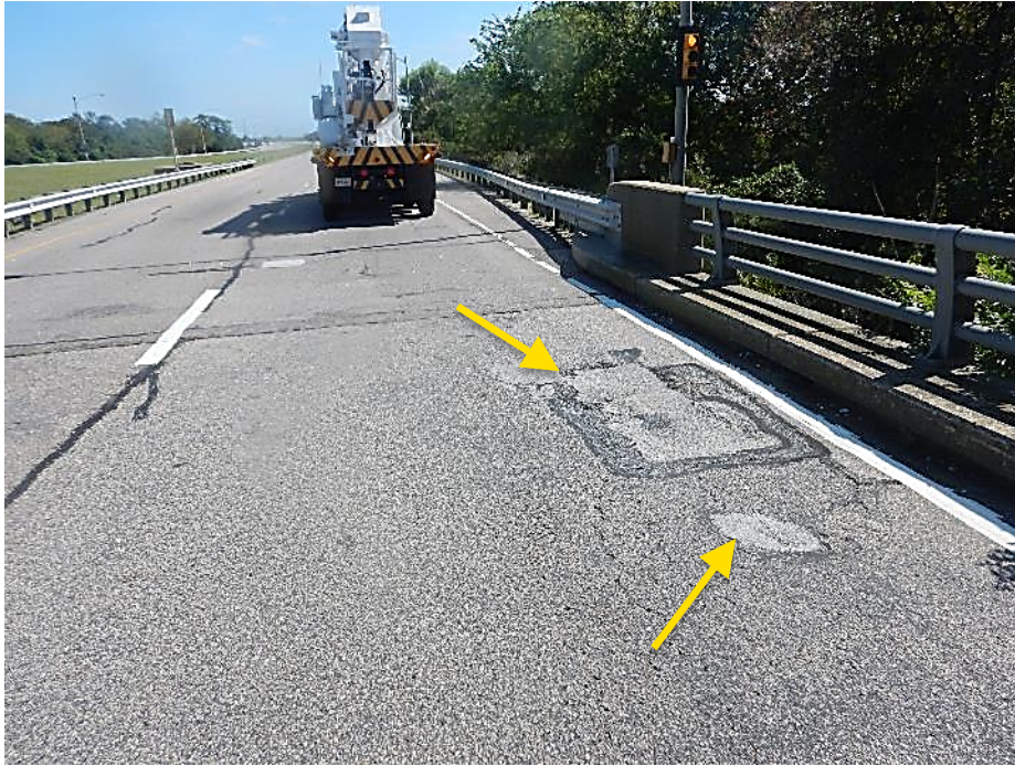
Photo 8.9-1: DNB18 Asphalt Wearing Surface – Repair Areas and Minor Cracking (Looking Northeast)
