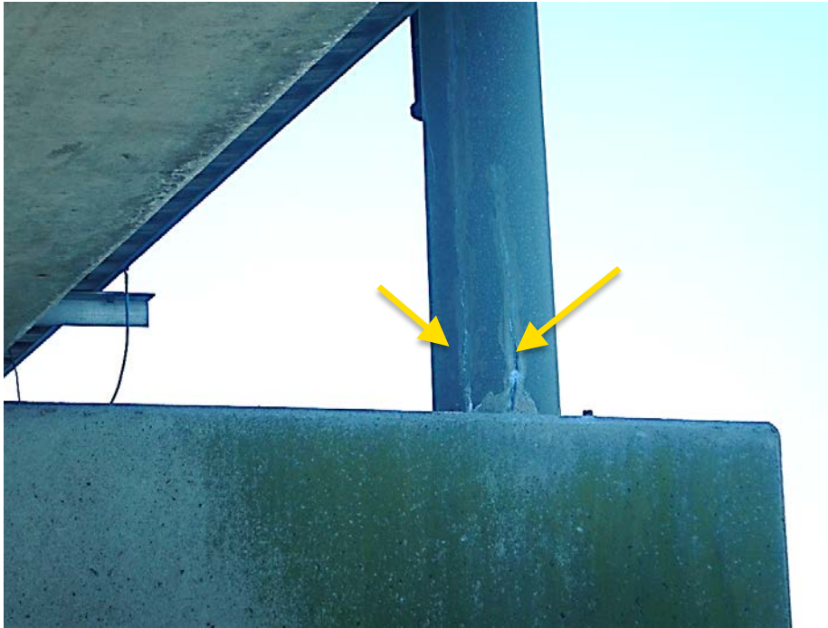
Photo 8.2-9: ASB119 Light Pole – Vertical Cracking Near Baseplate (Looking Southwest)
