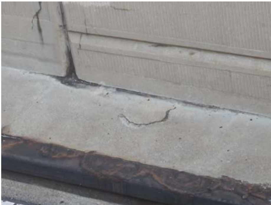
Photo 8.15-2: Portal Island 3 – Cracking/Delamination on West Sidewalk Approximately 600' from South (Looking Southwest)
