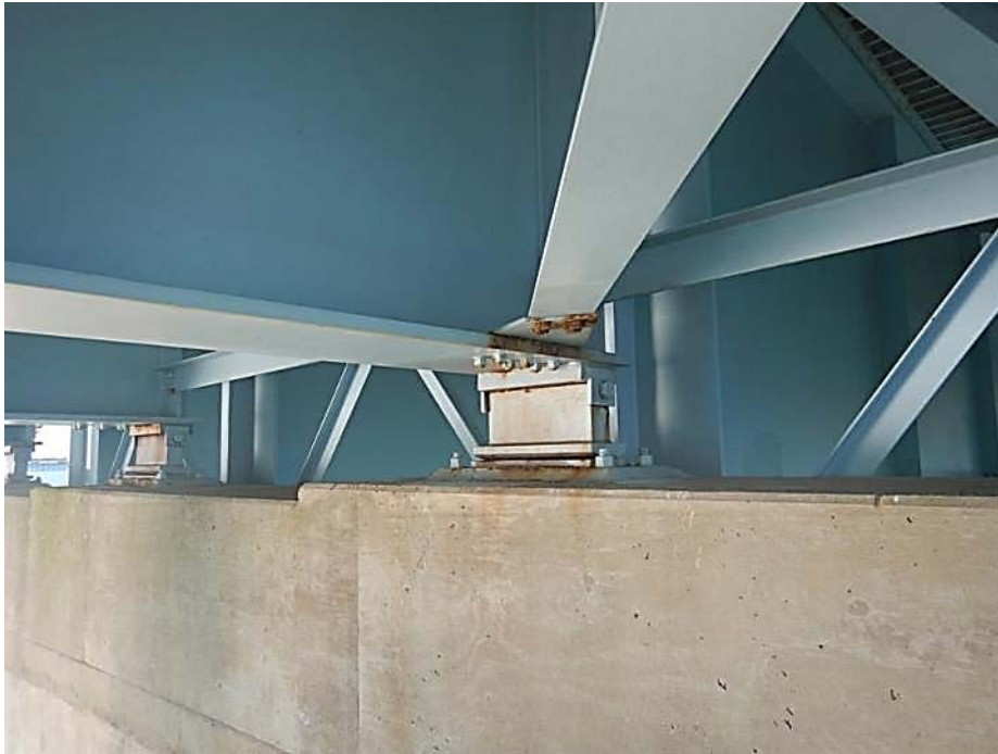
Photo 8.8-11: NCB-NB Pier 11 G2 Movable Bearing - Typical Condition of Isolated areas of Surface Rust (Looking Southeast)
