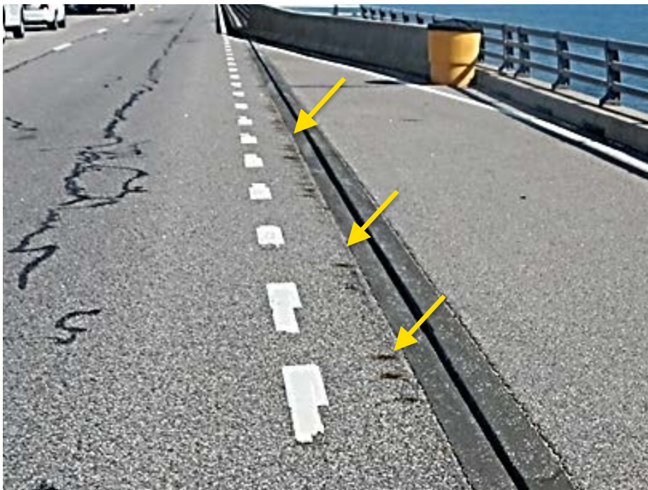
Photo 8.3-4: BNB132 Asphalt Wearing Surface – Rust Staining along Joint with EPO (Looking North)
