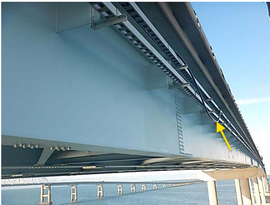
Photo 8.8-16: NCB-SB Span 12 Cable Tray – Cable Displaced from Tray (Looking Southeast)
