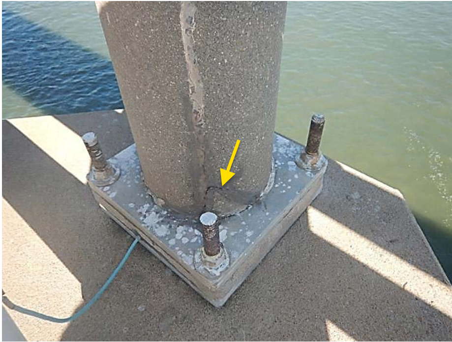
Photo 8.8-21: NCB-SB Span 9 Light Pole – Cracking at Baseplate was Previously Filled and Crack Has Reappeared (Looking Southwest)
