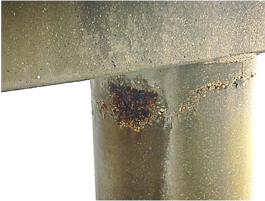
Photo 8.5-19: CNB175 Pile A - Spall with Exposed Reinforcement (Looking Southwest)
