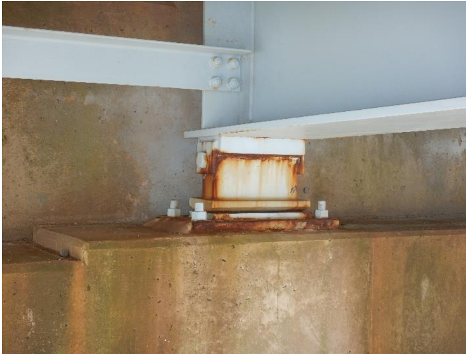
Photo 8.11-7: FIB-NB Pier 1 G3 Movable Bearing - Typical Condition of Isolated areas of Surface Rust (Looking Southwest)
