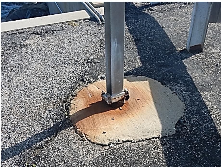
Photo 8.15-30: Portal Island 4 – Northwest Approach “Authorized Vehicles Only” Sign with Corroded Baseplate and Hardware (Looking Northeast)
