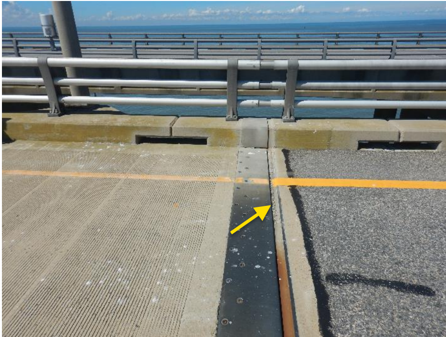
Photo 8.11-3: FIB4 Assembly Joint without Seal - Sliding Plate Expansion Joint Loose Debris Present in Joint (Looking West)
