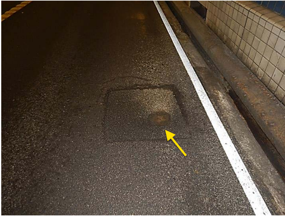
Photo 8.14-5: Asphalt Wearing Surface at STA 513+90 – Repair Patch with Depression (Looking North)
