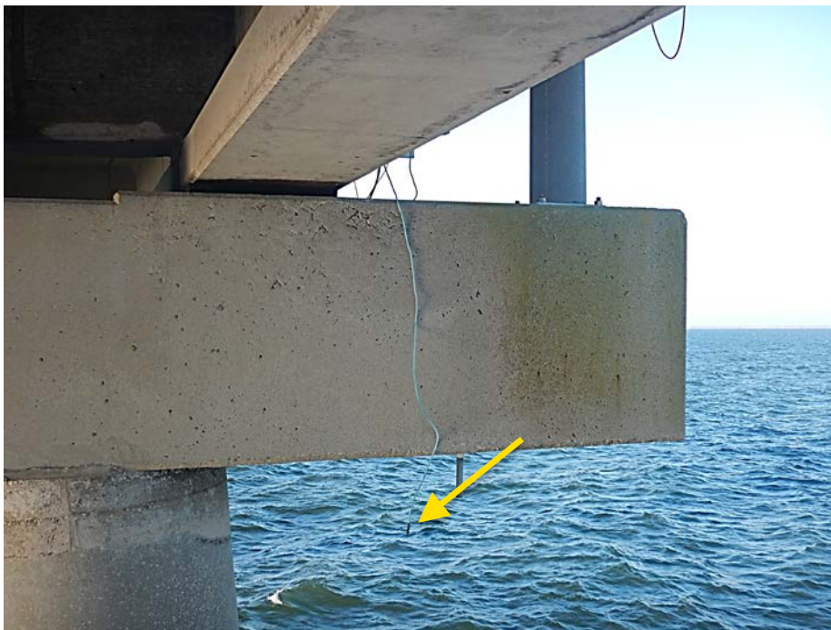
Photo 8.4-6: BSB Bent 107 - Disconnected Cable (Looking Southwest)
