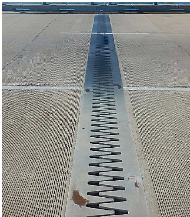
Photo 8.8-6: NCB-SB Pier 11 Assembly Joint without Seal – Tooth Expansion Joint Typical Condition with Minor and Isolated Locations of Freckled Rust (Looking East)
