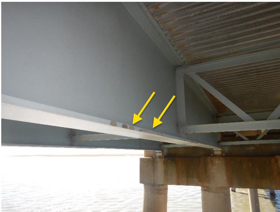
Photo 8.11-6: NCB-SB Span 1 Girder 2 – Top Protective Coating Peeled Off Exposing Zinc Primer (Looking Southeast)
