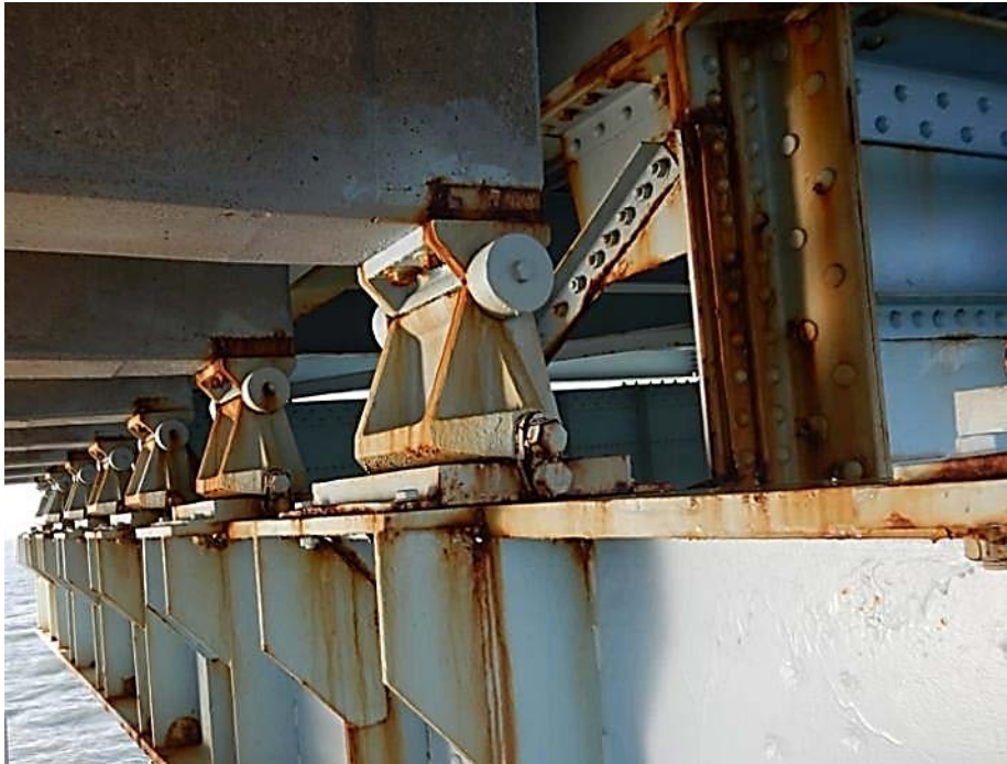
Photo 8.9-11: DNB1 – Rocker Bearings with Minor Paint Failure, Rust Staining, and Relatively No Section Loss (Looking Southeast)
