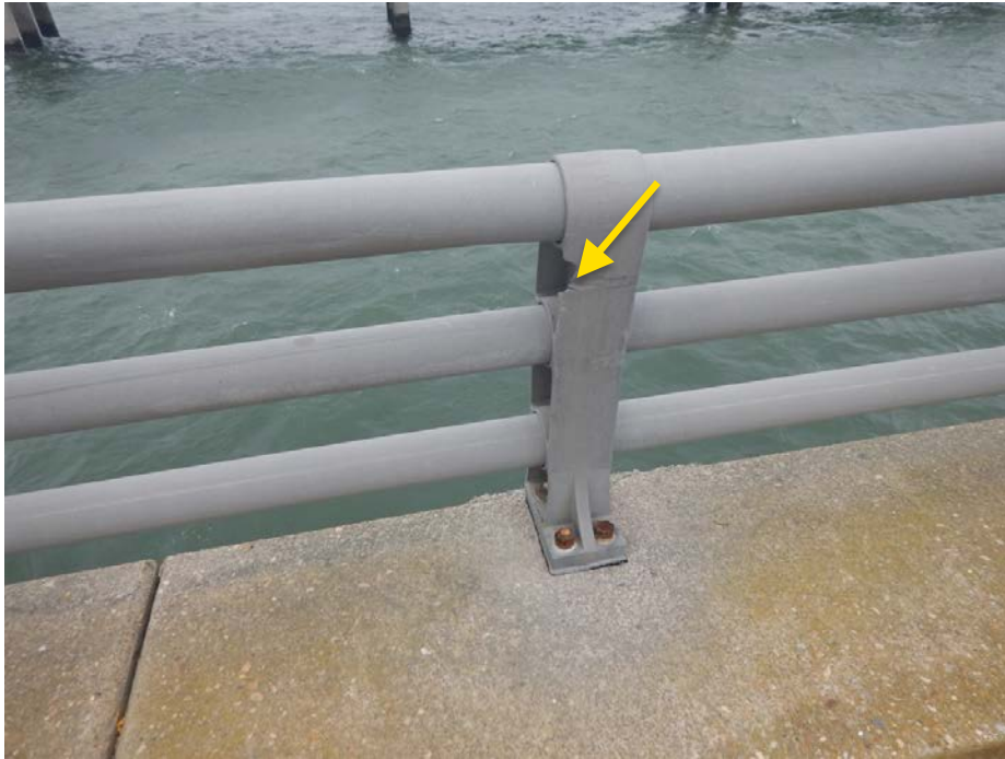
Photo 8.5-3: CNB181 Metal Bridge Railing 2 nd Post from the North - Impact Damage to Post above Middle Rail (Looking Northwest)
