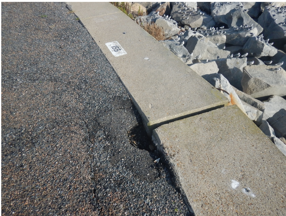
Photo 8.15-20: Portal Island 3 – Splash Wall Blocks 155-156, Typical Isolated Areas of Settlement and Erosion at Splash Wall Joints (Looking North)
