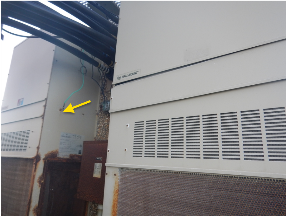
Photo 8.15-9: Portal Island 3 Utility Structure – Disconnected Grounding Cable (Looking Southeast)
