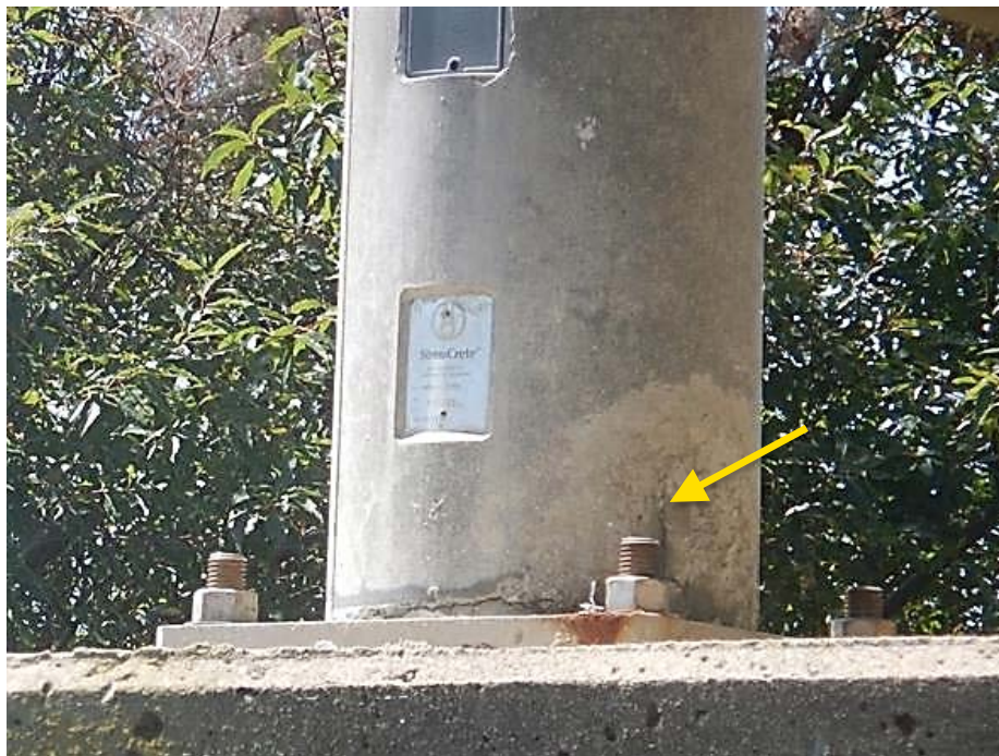
Photo 8.10-6: DSB15 Light Pole – Delamination and Vertical Cracking Near Baseplate (Looking Northwest)
