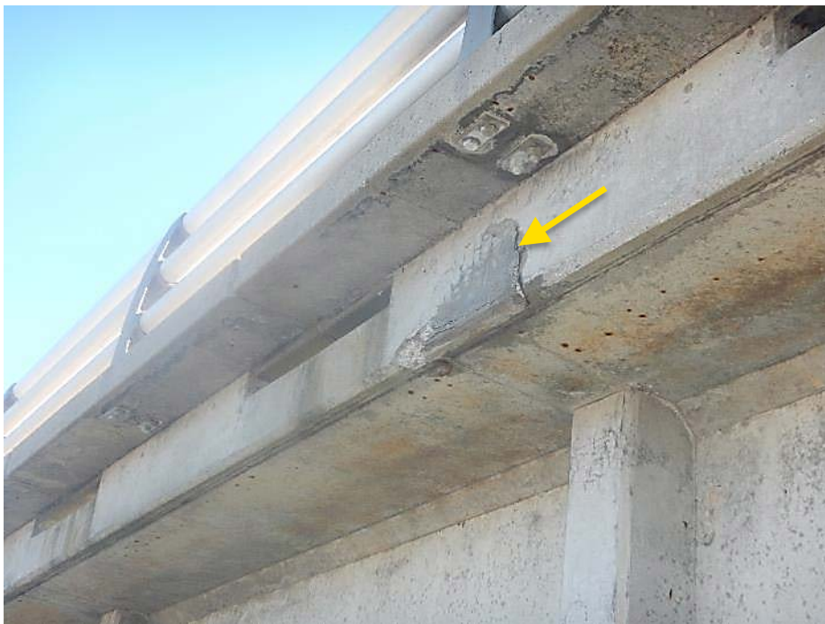
Photo 8.11-4: ENB6 Reinforced Concrete Deck – Delamination (Looking Northeast)
