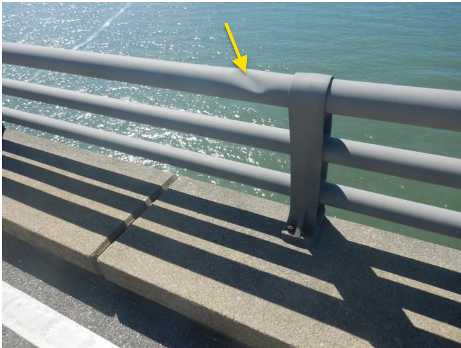
Photo 8.12-2: ESB13 Metal Bridge Railing 4 th Span from the North - Impact Damage to Top Rail (Looking Southwest)
