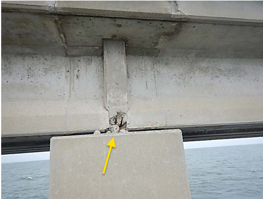
Photo 8.6-7: CSB153 Girder 6 – Spalling at Closure Diaphragm with Exposed Reinforcement and Prestressing Strand (Looking West)
