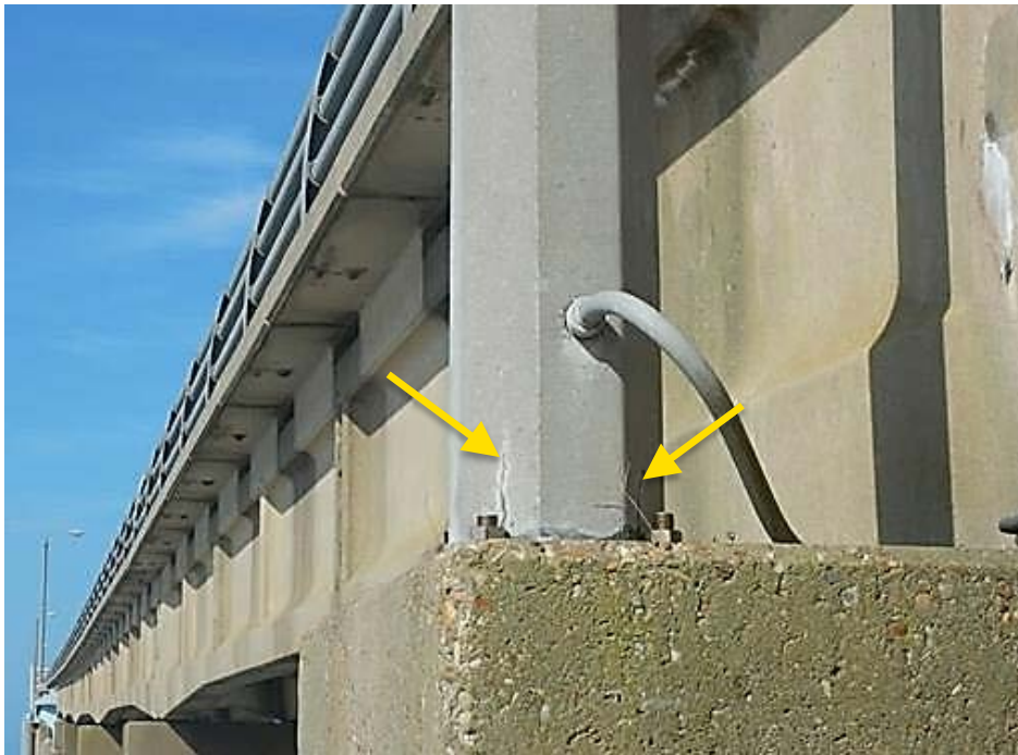
Photo 8.9-14: DNB5 Light Pole – Cracking at Baseplate (Looking Southwest)
