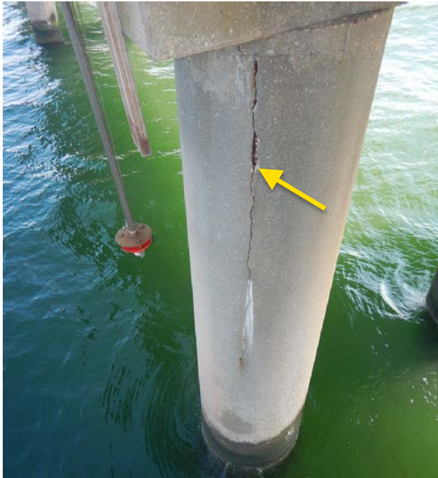
Photo 8.3-19: BNB131 Pile A – Wide Crack along Exposed Prestressing Strand with Efflorescence and Rust Staining (Looking Northeast)
