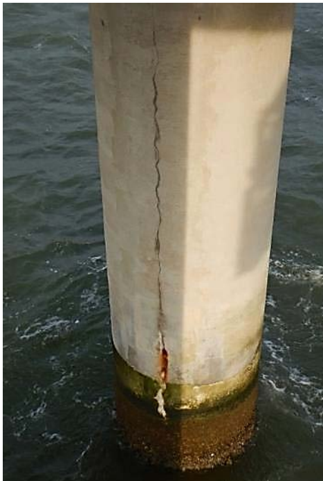
Photo 8.1-12: ANB75 Pile A - Wide Crack in Pile through Protective Coating with Rust Staining (Looking West)
