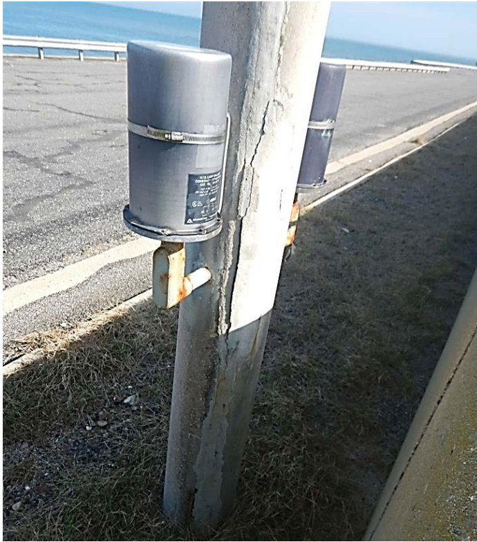
Photo 8.15-29: Portal Island 4 – 2 nd Light Pole from Northwest with Delamination and Cracking extending towards the Base (Looking Northwest)
