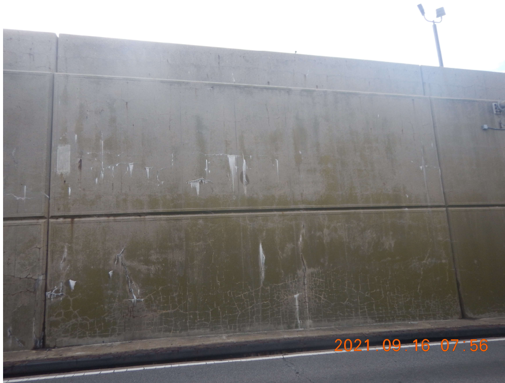
Photo 60: TSCT Island 2 Open Approach –Typical Satisfactory Condition with Minor Cracking with Efflorescence (Looking East)
