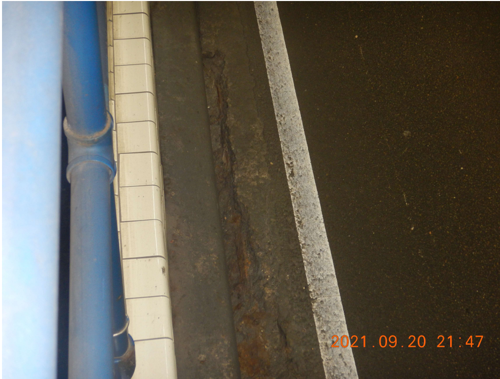
Photo 64: TSCT Roadway – STA193+50 Random Edge Spalling with Exposed Reinforcement along Roadway Curb, Worst Case Scenario (Looking North)
