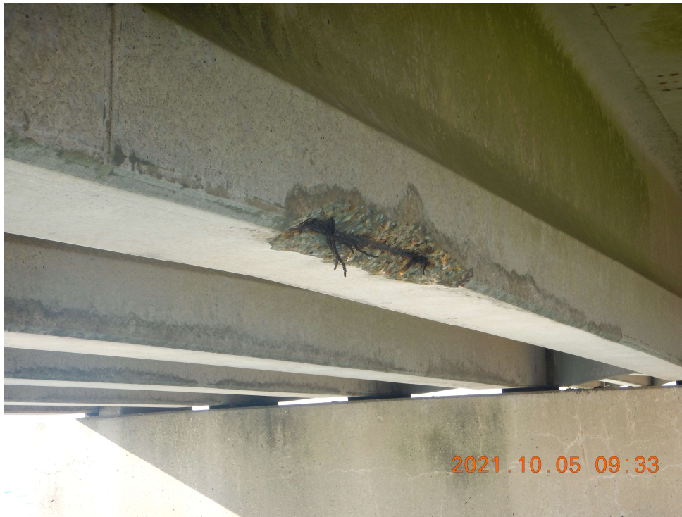
Photo 35: CNB40 Prestressed Girder – Spalling with Exposed and Broken Strands at Girder 5 (Worst Case Observed) (Looking Southeast)
