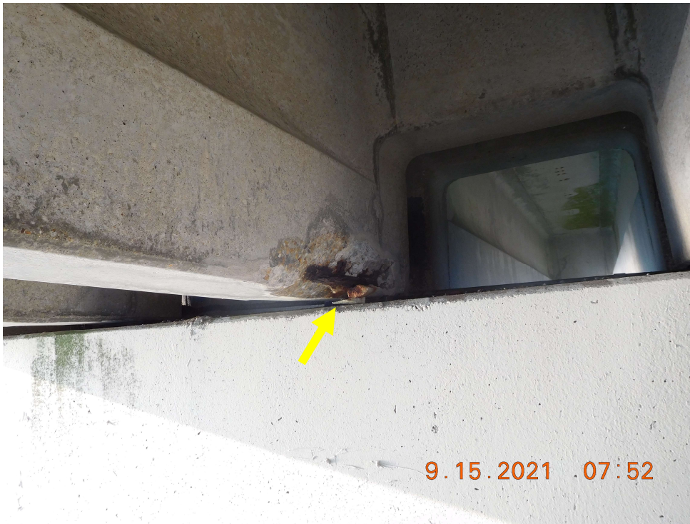
Photo 3: ANB37 Prestressed Concrete Girder – Spalling with Exposed Reinforcement in Bottom Flange of Girder 3 Beam End, Defect represents <0.1\% of Total Quantity (Looking Southeast)
