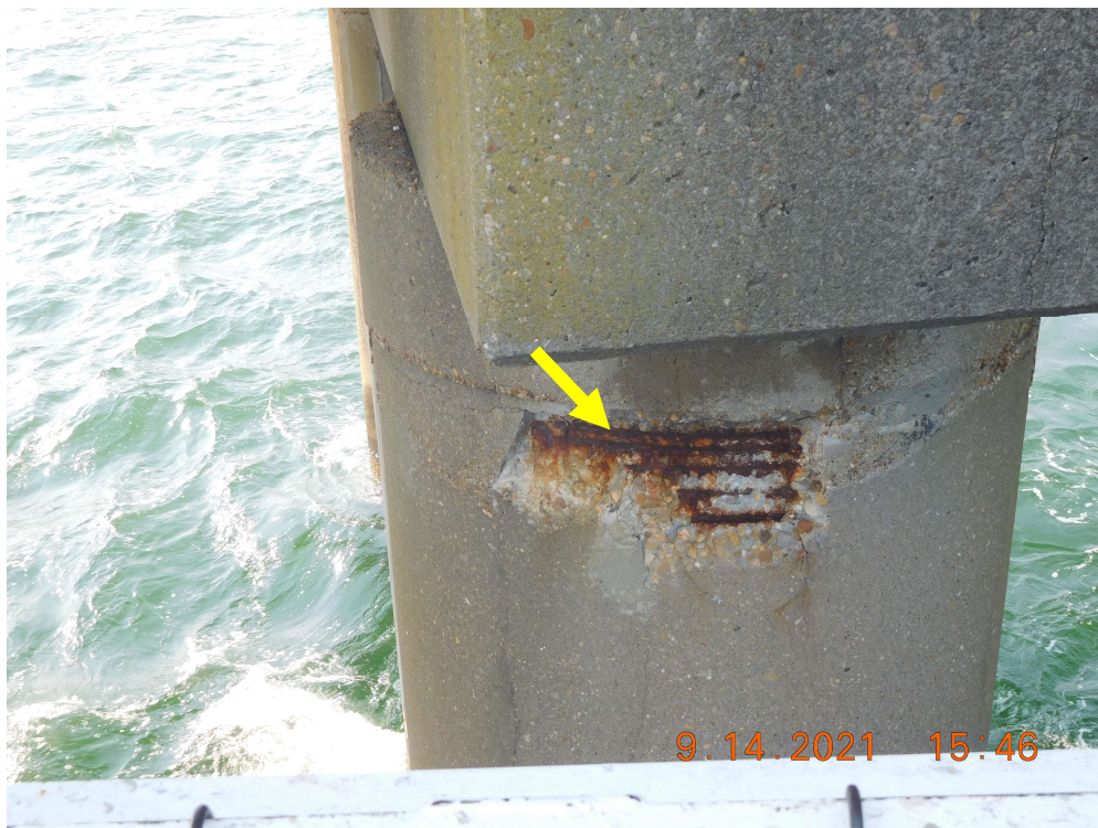
Photo 22: BNB40 Prestressed Concrete Pile – Spall with Exposed Reinforcement at Top of Pile C (Looking West)
