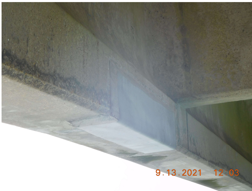
Photo 36: CNB13 Prestressed Girder 1 – Typical Sound Patch, Defect Represents 2.5% of Total Quantity (Looking Southeast)
