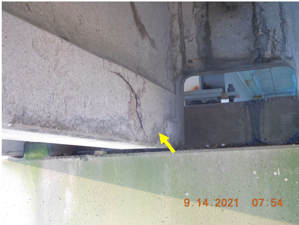
Photo 16: BNB3 Prestressed Girder – Delamination in Bottom Flange of Girder 3 at Bent 3 (Looking South)
