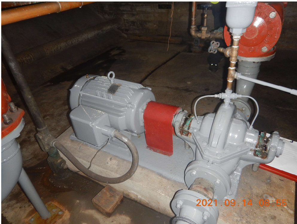
Photo 57: TSCT Pumps –Typical Good Condition of Mid-channel Pump #2
