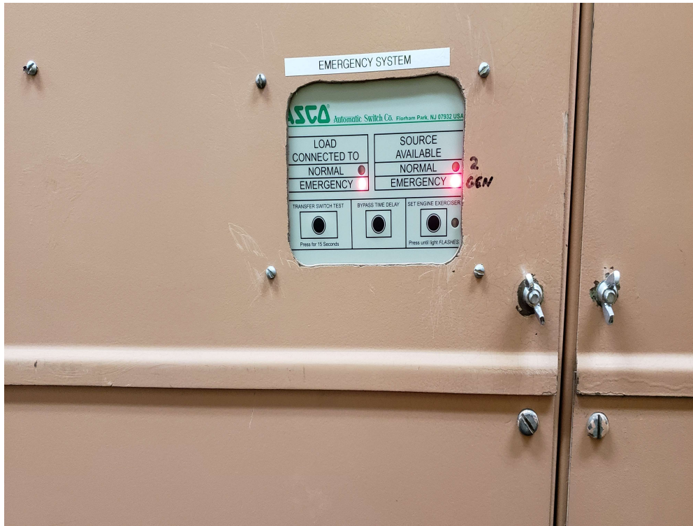
Photo 58: TSCT Island 1 –ATS Status Indicators during Emergency Testing Phase
