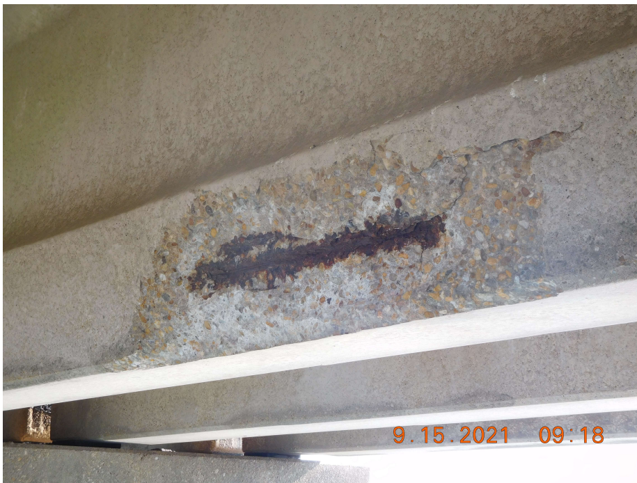
Photo 4: ANB37 Prestressed Concrete Girder – Spall with Two Exposed Strands in Bottom Flange of Girder 3, Defect Represents <0.1\% of (Looking Northeast)
