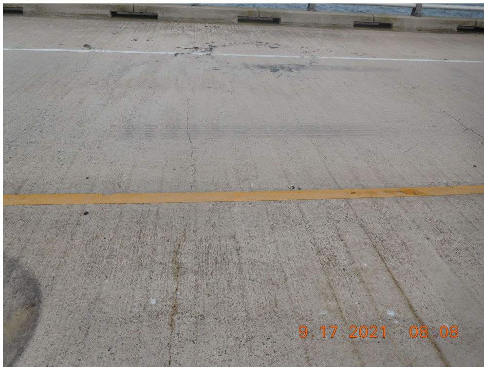
Photo 24: BSB16 Reinforced Concrete Top Flange – Typical Satisfactory Condition with Typical Transverse Cracking (Looking Southwest)
