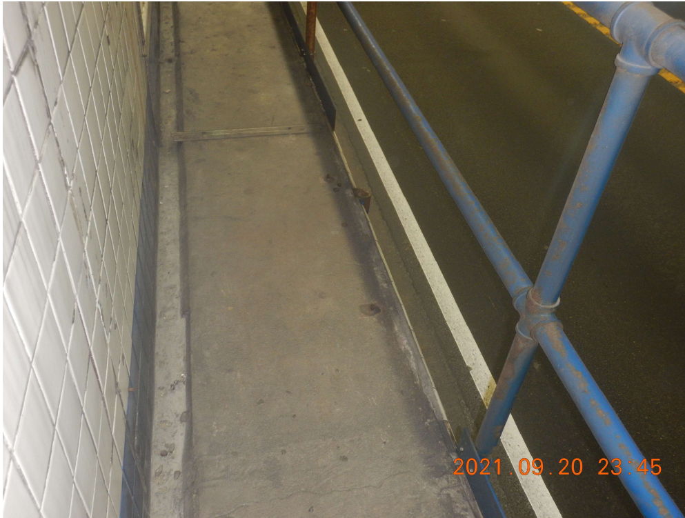
Photo 66: TSCT Steel Railing – STA203+50 Missing toe board and post, Worst Case Location (Looking Northeast)
