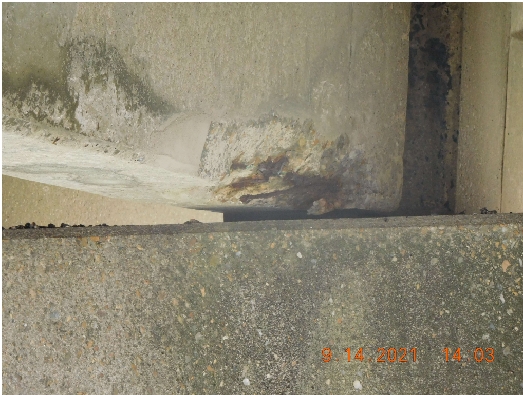
Photo 17: BNB29 Prestressed Concrete Girder – Spall with Exposed Prestressing Strand in Girder 2 in Zone 1 (Looking Southeast)
