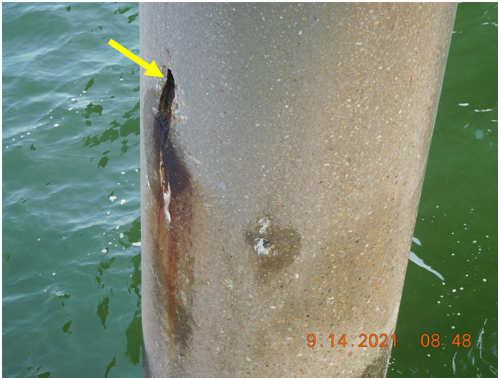
Photo 19: BNB7 Prestressed Concrete Pile – Spalling with Exposed Reinforcing on West Face of Pile A (Looking North)
