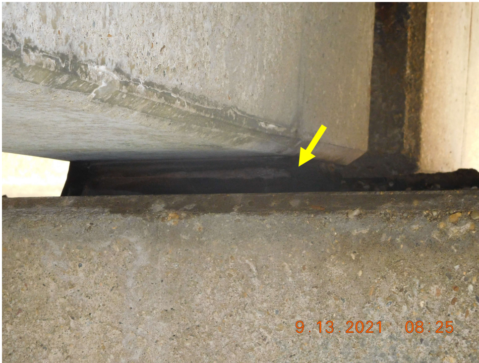
Photo 37: CNB3 Elastomeric Bearing – Deformed Elastomeric Bearing at Bent 4 for Beam 6 (Looking Northwest)
