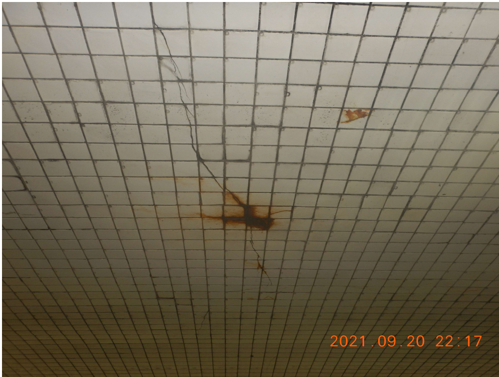
Photo 65: TSCT Roadway –STA 235+20 Cracked Ceiling Tiles with Minor to Moderate Rust Staining, Worst Case Scenario (Looking East)
