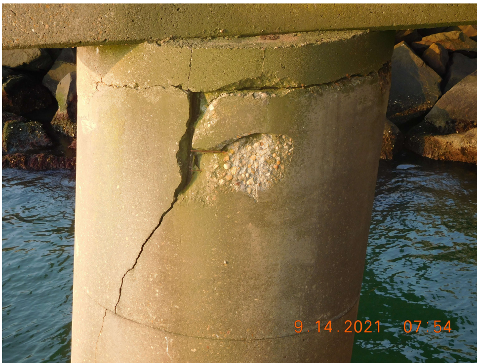
Photo 18: BNB3 Prestressed Concrete Pile – Moderate Cracking and Spalling in Pile C (Looking South)
