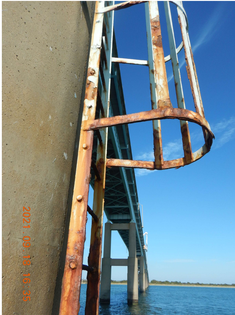
Photo 46: NCB-NB10- Peeling Paint with Minor to Moderate Corrosion of Access Ladder at Pier 10
