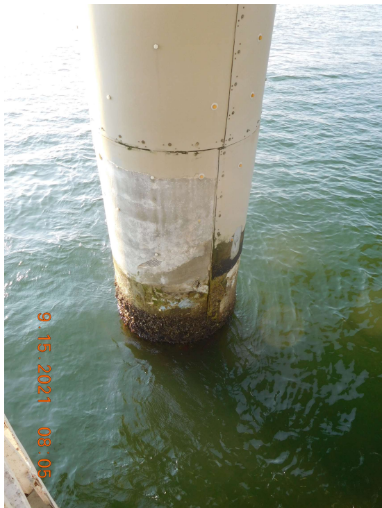
Photo 6: ANB37 Pile C – Missing Bottom Section of Protective Jacket (Looking Southeast)
