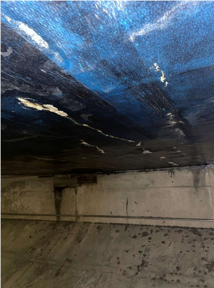
Photo 69: TSCT Invert Slab – STA197+40 Repaired Spall with Fiber Wrap on Underside of Invert Slab
