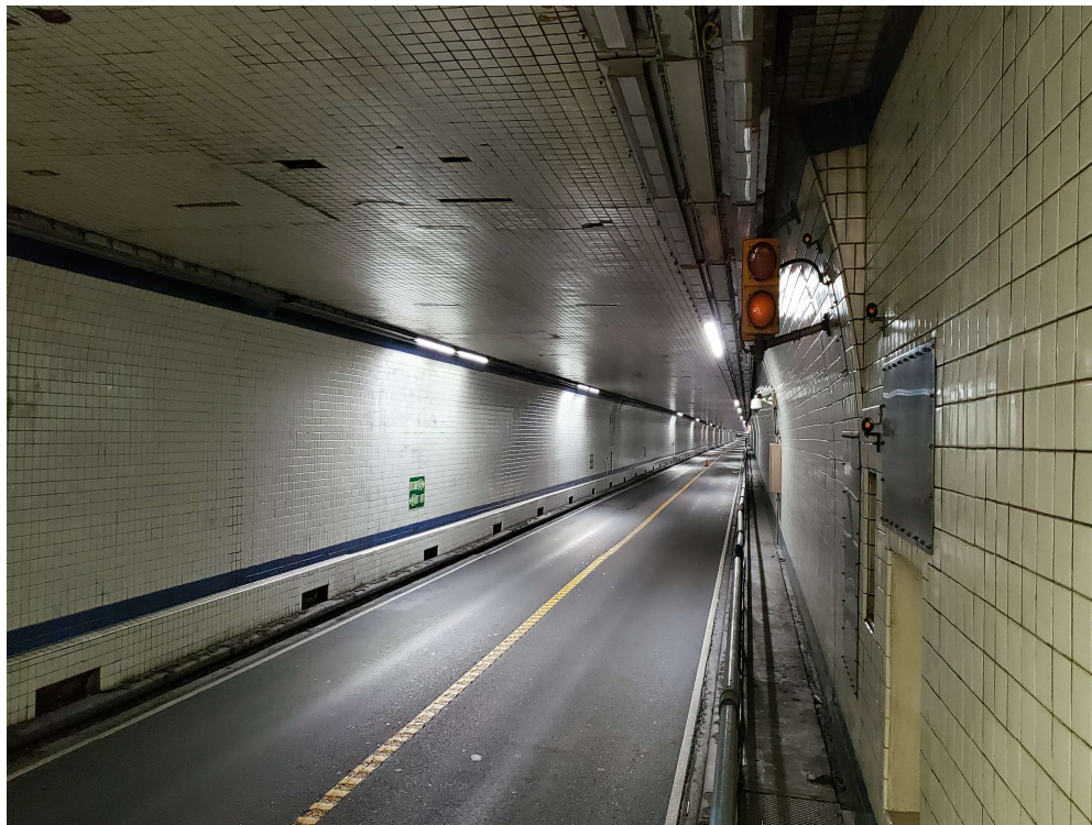
Photo 59: TSCT Lighting –Typical Condition of Emergency Lighting at Island 2 Portal (Looking South)
