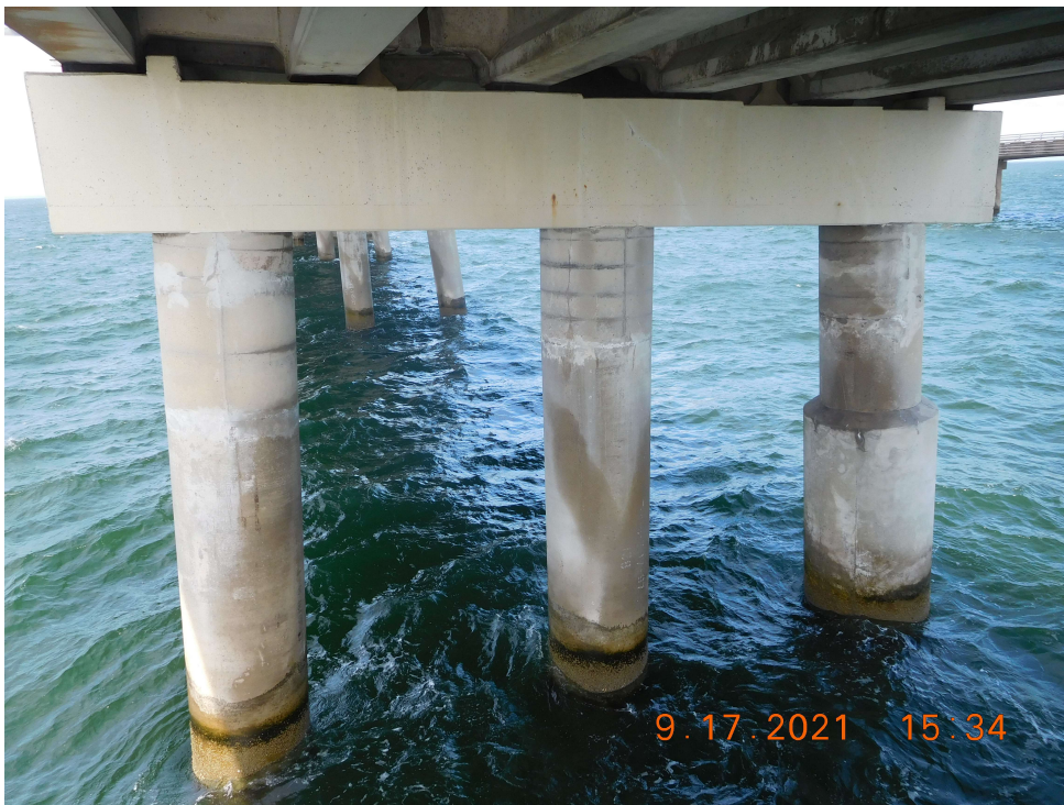
Photo 28: BSB186 Prestressed Concrete Pile – Hairline Cracking with Minor Efflorescence in Pile C (Looking Northeast)
