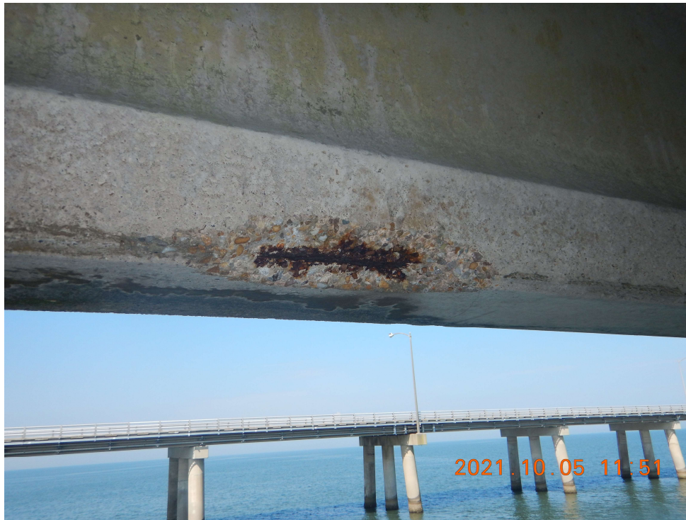
Photo 5: ANB77 Prestressed Concrete Girder – Spall with Exposed Strand in Bottom Flange of Girder 8, Defect Represents <0.1% of Total Quantity (Looking Northwest)
