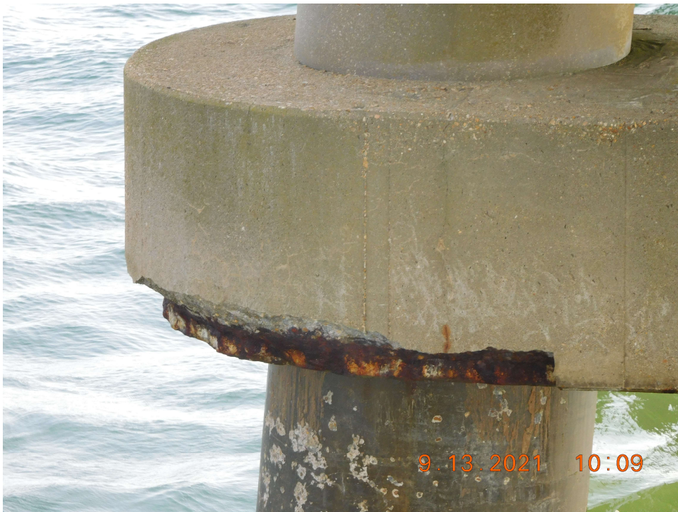
Photo 38: CNB8 Reinforced Concrete Pier Cap – Spalling with Exposed Reinforcement at Base of Cap over Pile A (Looking North)
