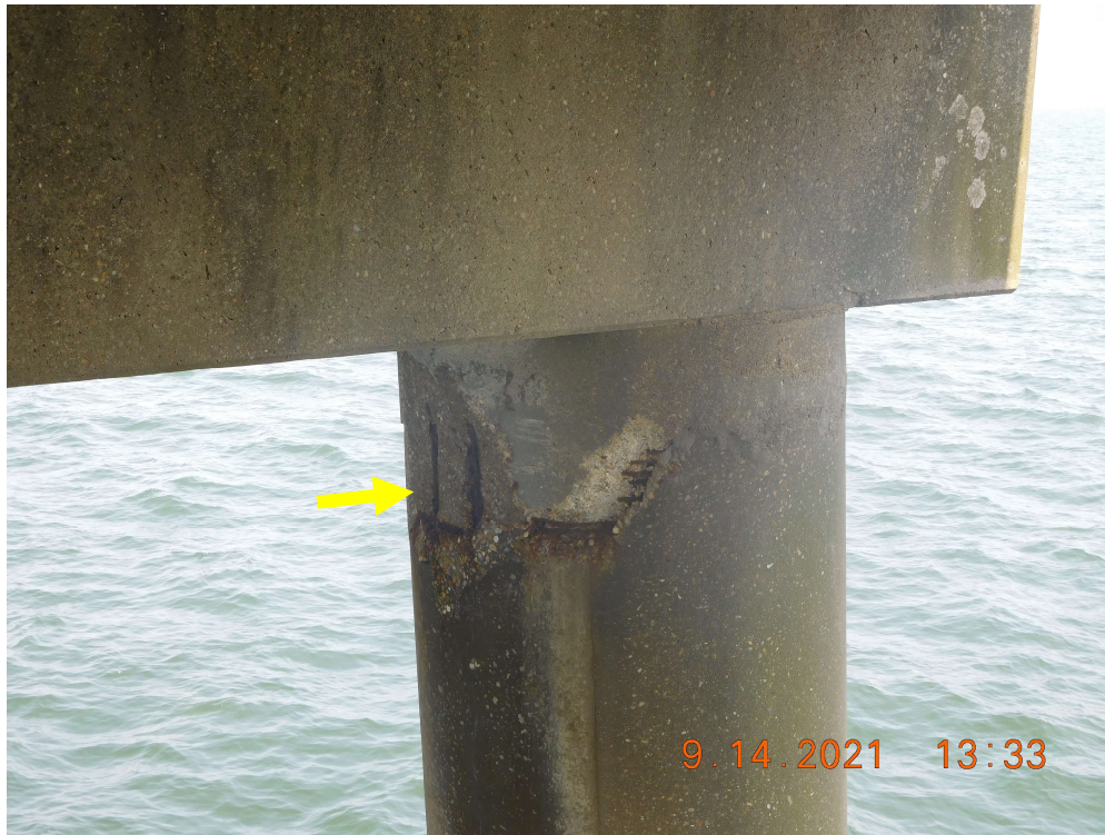
Photo 21: BNB25 Prestressed Concrete Pile – Spall with Exposed Reinforcement at Top of Pile C (Looking East)
