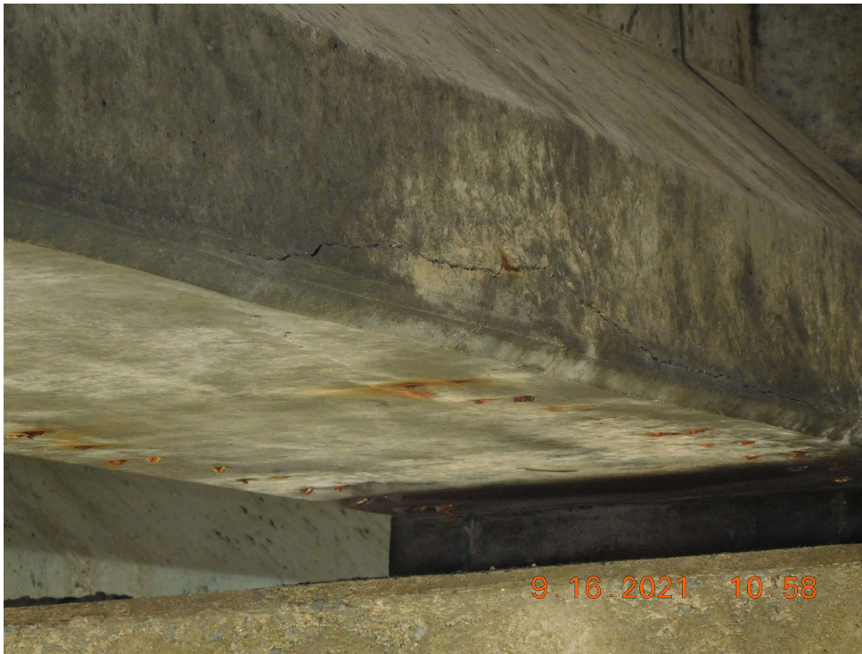
Photo 42: CSB227 Prestressed Concrete Girder – Delaminated Concrete at Bottom Flange of Girder 3
