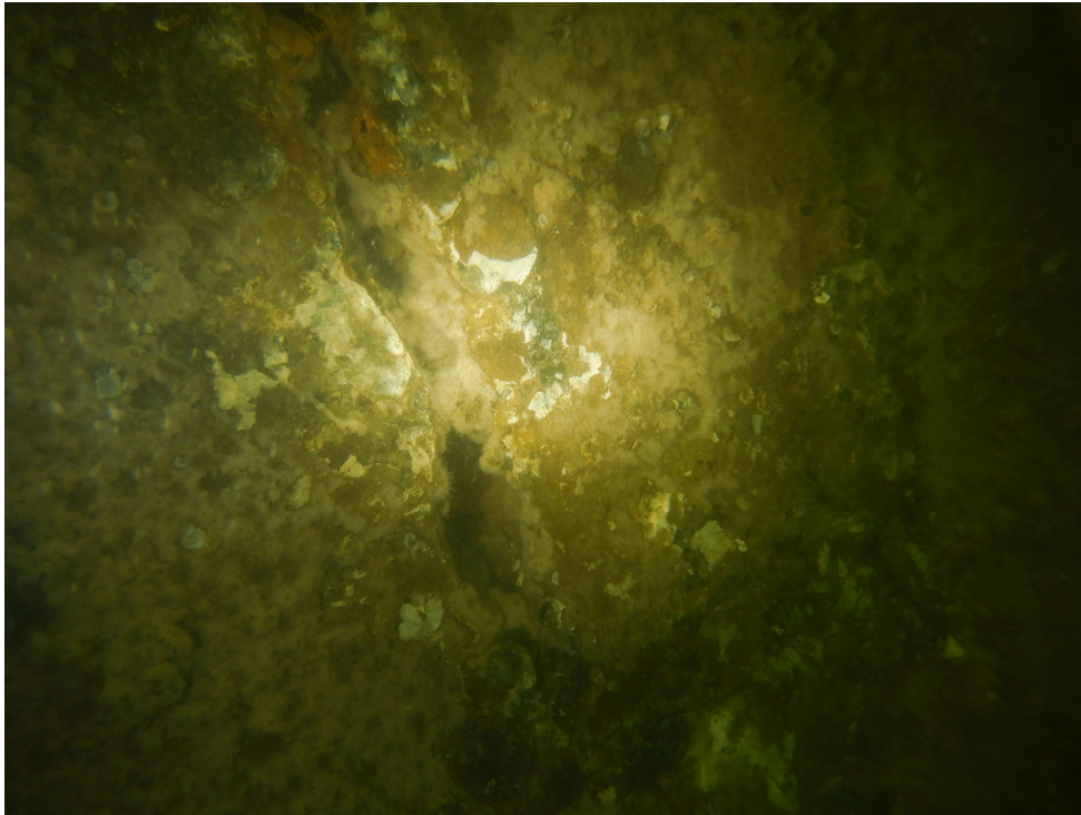
Photo 31: BSB101 Pile C – Minor Cracking in South Face (Looking North)
