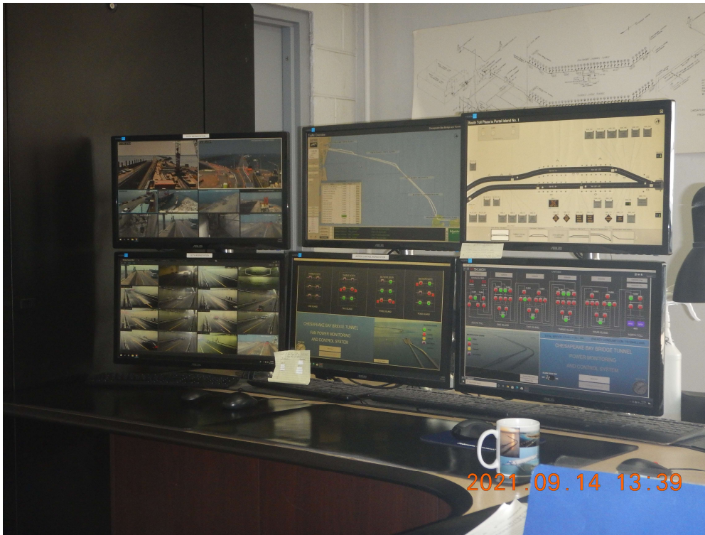
Photo 52: TSCT Island 1 Control Room –Typical Condition of Camera Control Room
