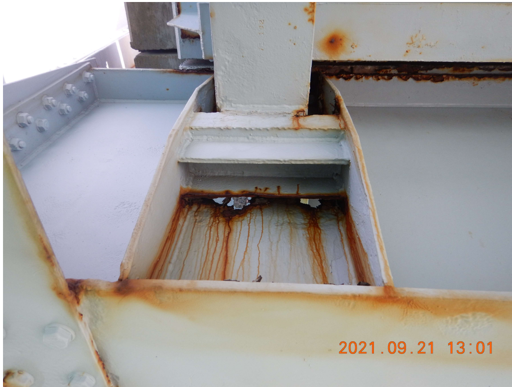
Photo 47: NCB-NB FB3'- Corrosion Holes in Web of Floorbeam at Stringer 1
