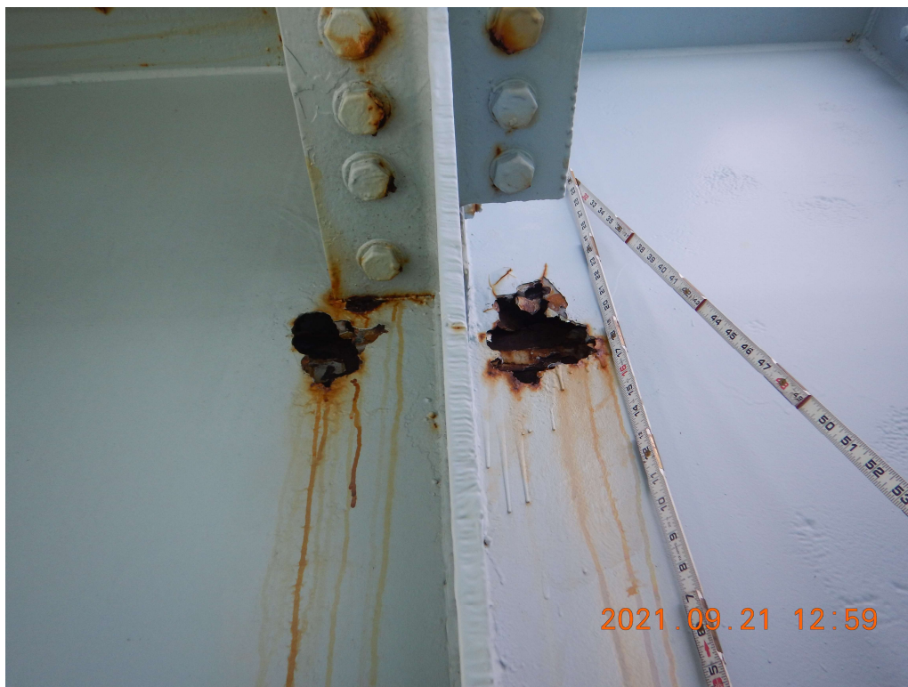
Photo 48: NCB-NB FB3' – Corrosion Holes in Transverse Stiffeners at Stringer 1
