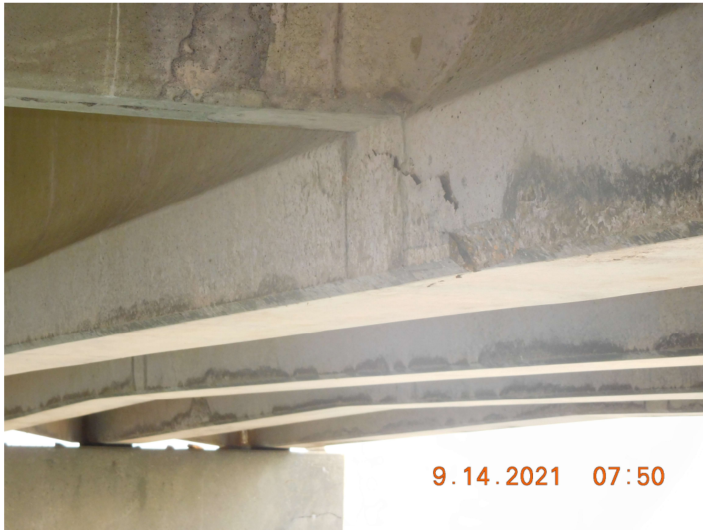
Photo 15: BNB3 Prestressed Girder – Delamination in Bottom Flange of Girder 4 (Looking East)
