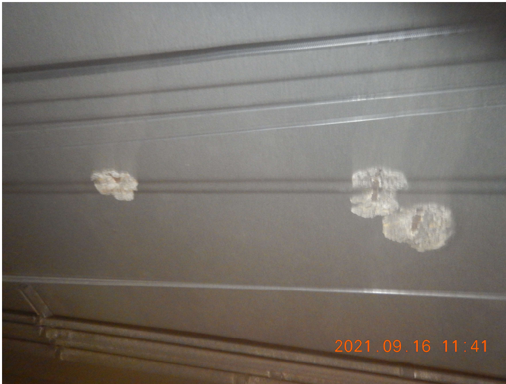
Photo 62: TSCT Tunnel Liner –STA 191+00 Minor Spalling with Exposed reinforcement (Looking East)
