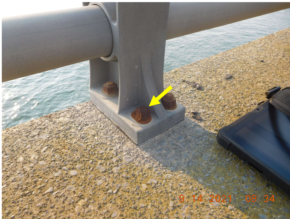
Photo 10: BNB4 Metal Bridge Railing – Corrosion with Section Loss of Rail Post Connections (Looking Southeast)
