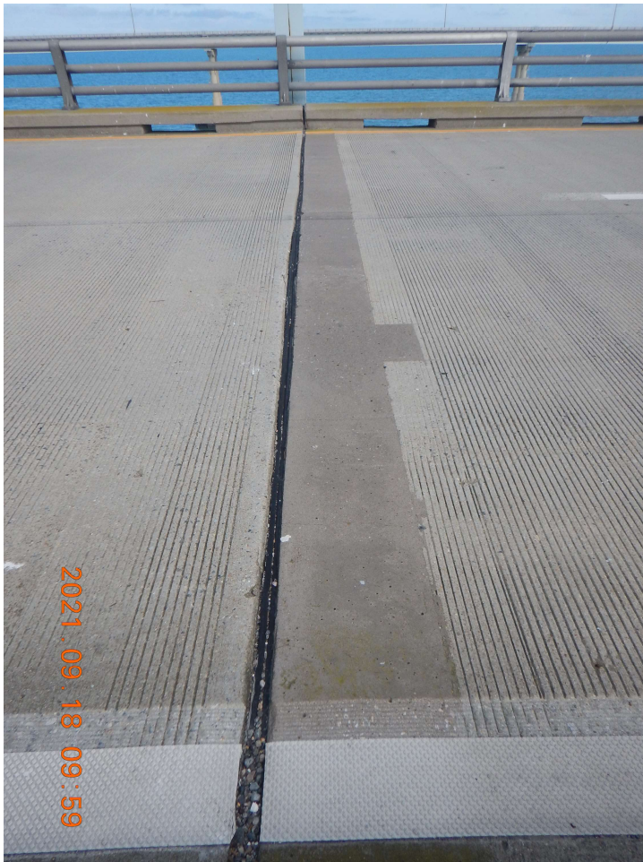
Photo 45: NCB-NB9- Deck patch adjacent to joint in satisfactory condition
