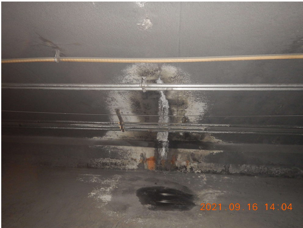
Photo 63: TSCT Tunnel Liner –STA 231+20 in Exhaust Duct Hairline Cracking with Heavy Efflorescence (Looking East)
