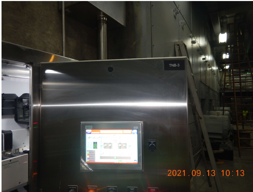
Photo 54: TSCT Island 2 Fans –HMI for New Ventilation Fan MCCs
