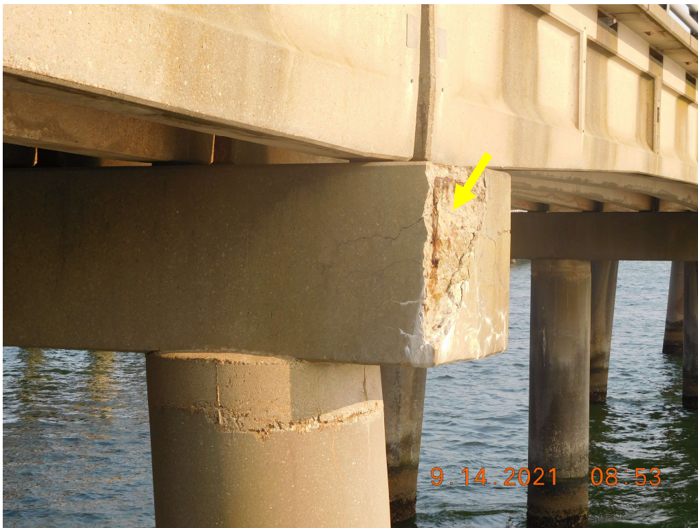
Photo 20: BNB7 Reinforced Concrete Pier Cap – Spalling with Exposed Reinforcement on East Face (Looking Northwest)
