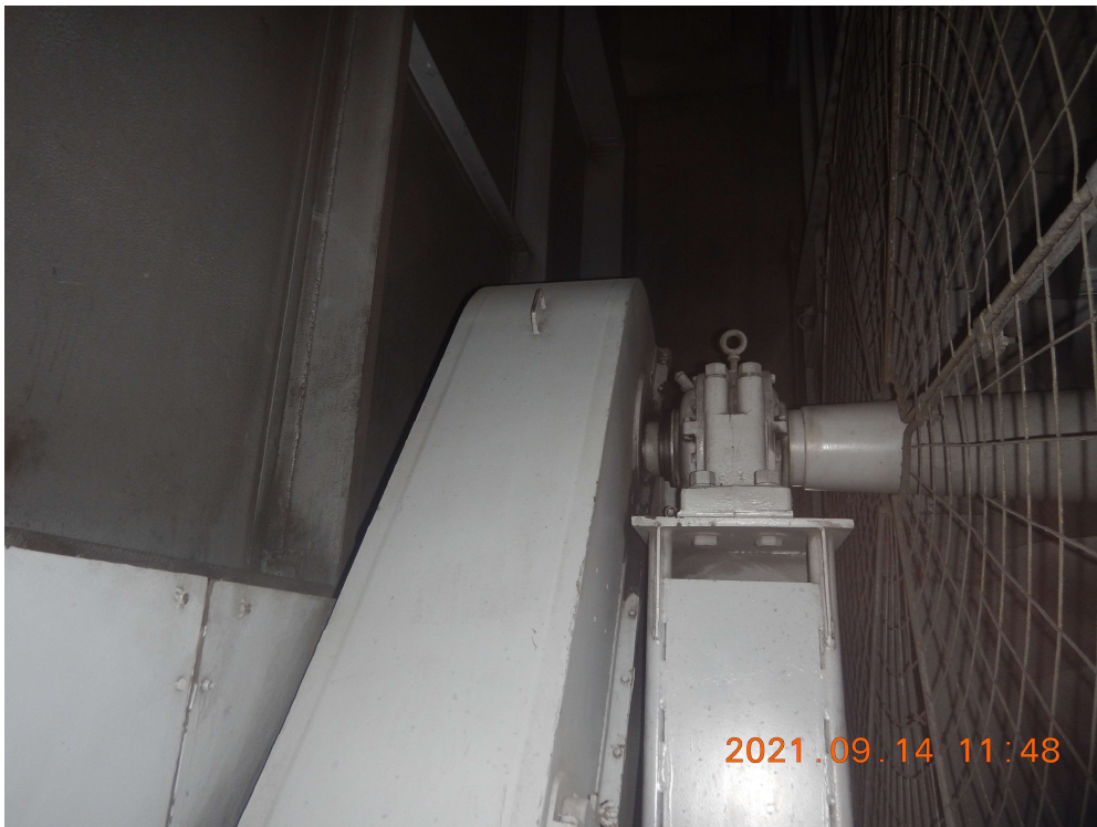
Photo 53: TSCT Island 1 Fans –Typical Good Condition
