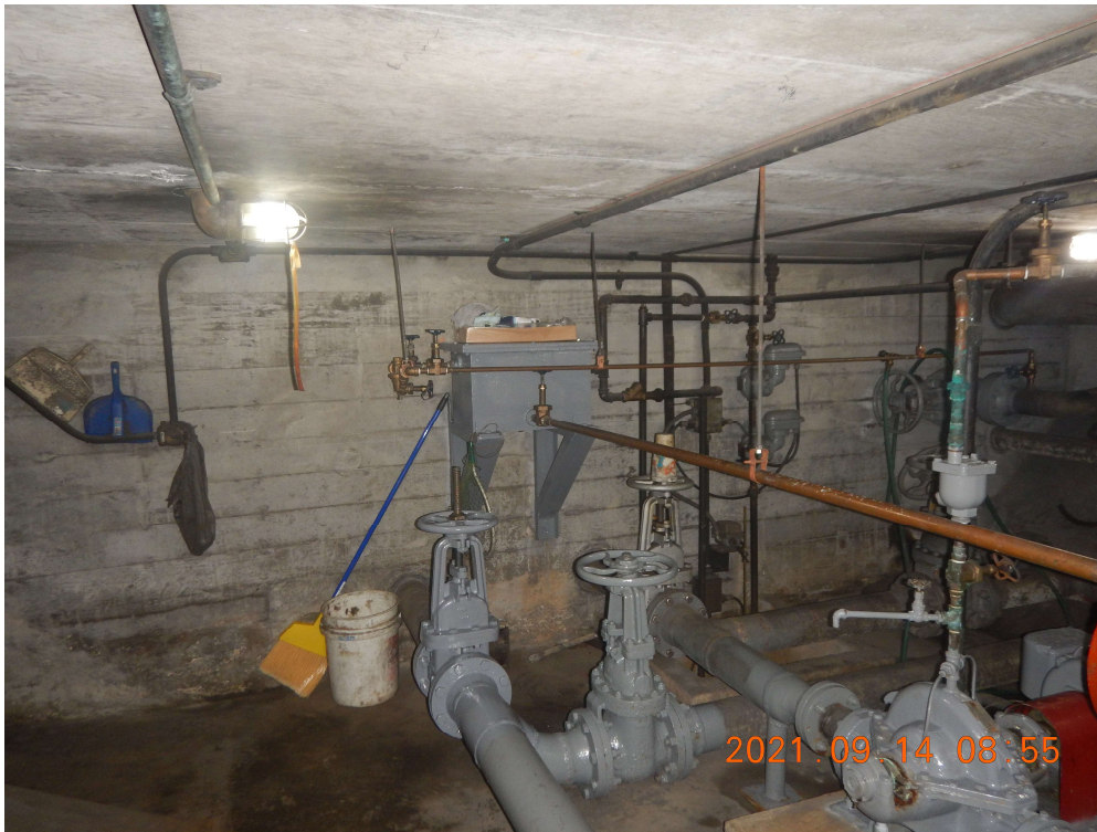
Photo 56: TSCT Pumps –General View of Mid-channel Pump Room
