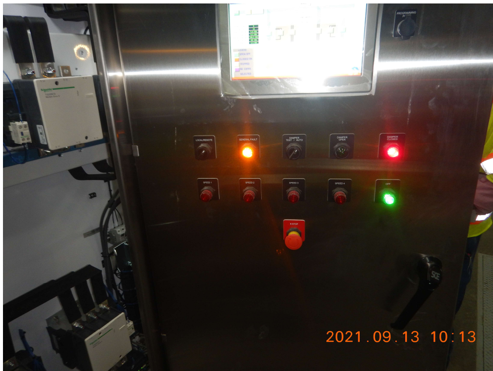
Photo 55: TSCT Fans –Typical New Ventilation Fan MCC Controls on Front Panel
