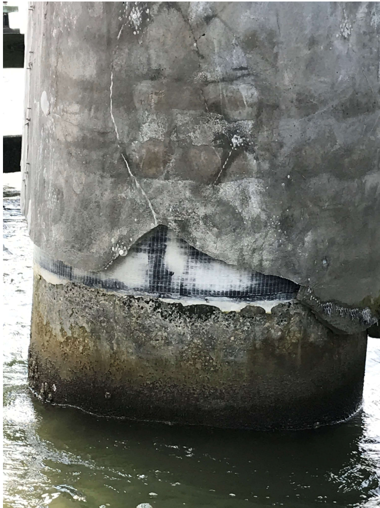
Photo 49: FIB-SB Bent 3, Pile C– Missing Fiberglass Jacket and Grout Annulus with Exposed Fiber Mesh
