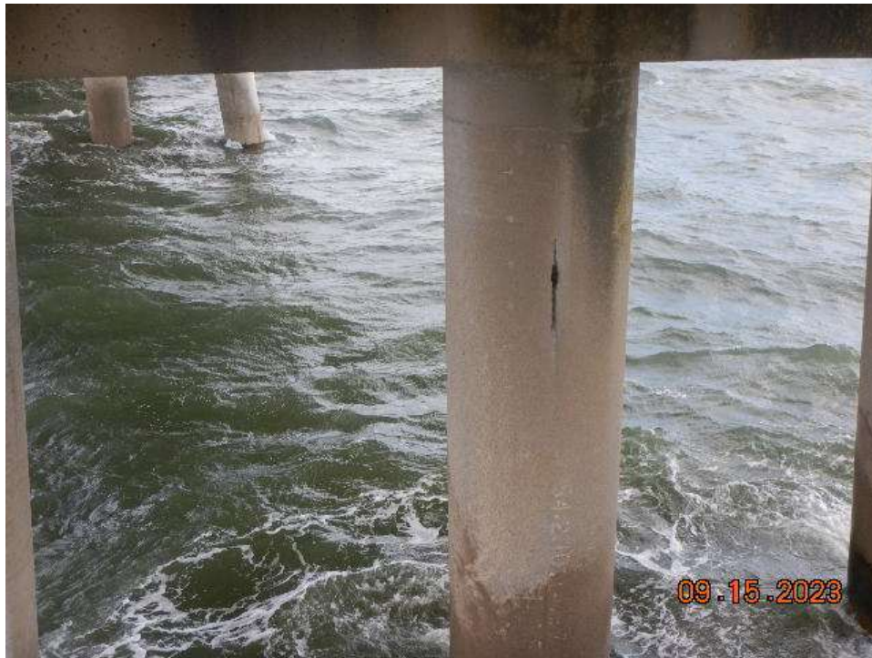
Photo 36: BSB111 Prestressed Concrete Pile – Spall in Pile B in South Face
