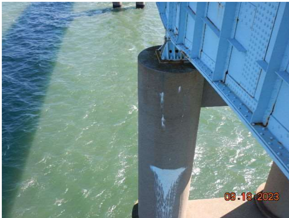
Photo 62: NCB-NB7 Reinforced Concrete Column – Cracking with Heavy Efflorescence on Column 1 at Bent 7
