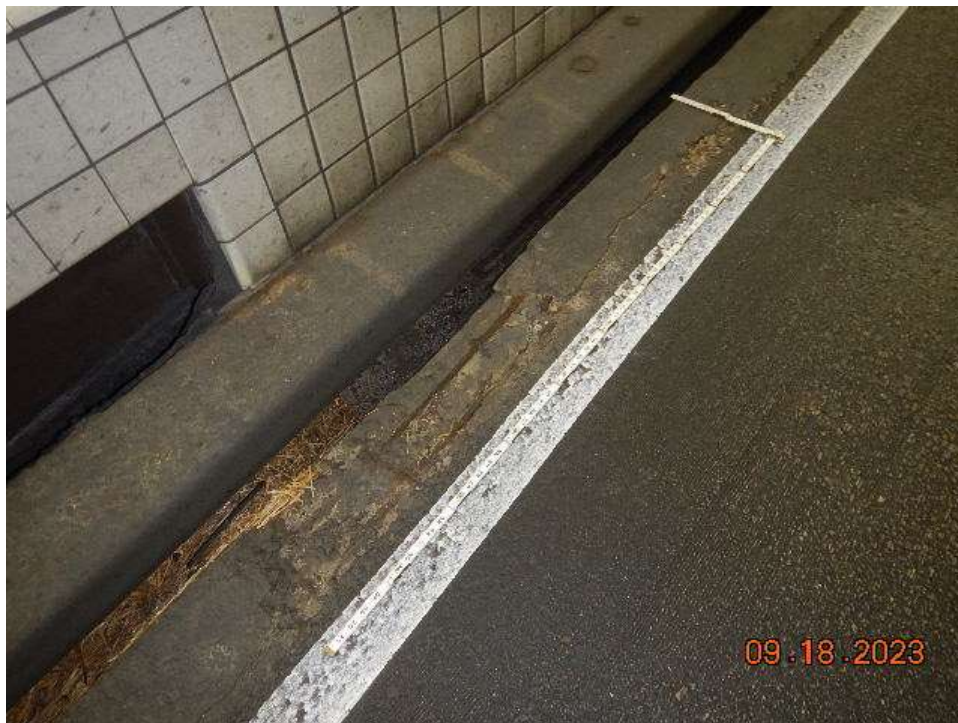
Photo 87: Typical Spalling of Invert Slab along Curblin (175 SF Total in Tunnel)
