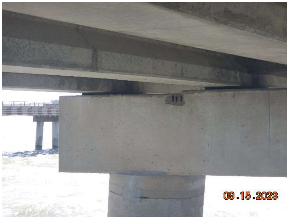
Photo 17: ASB98 Reinforced Concrete Pier Cap – Shallow Spall with Exposed Reinforcing
