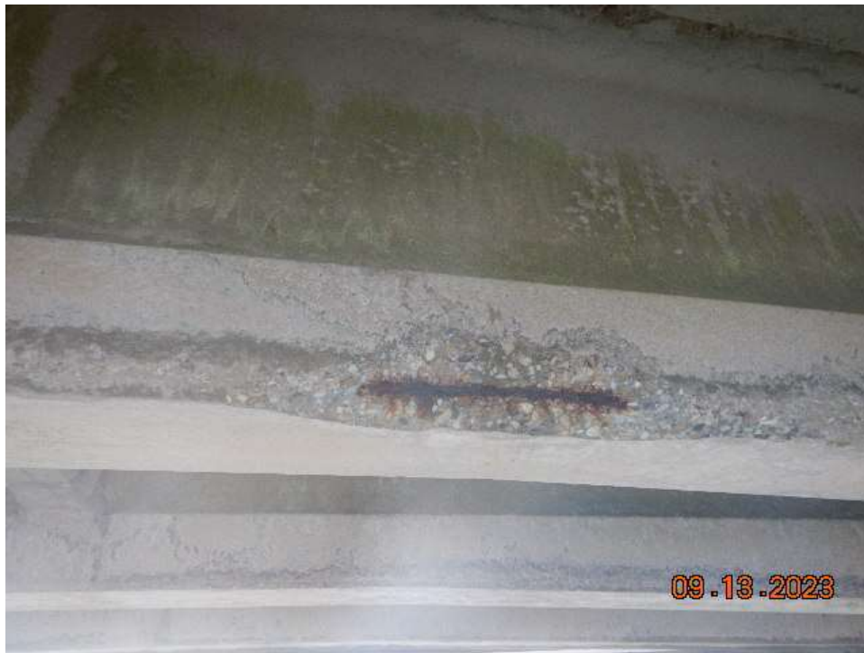
Photo 42: CNB137 Prestressed Concrete Girder – Girder 3 Spall with Exposed & Corroded Strand
