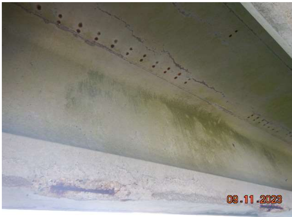
Photo 8: ANB157 Prestressed Concrete Girder – Two (2) Spalls with Exposed Strand in Girder 8
