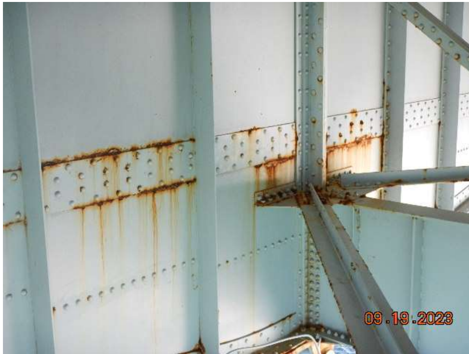
Photo 59: NCB-NB5 Steel Girder – Typical Corrosion at Haunch Splice, Girder 2 at Pier 6
