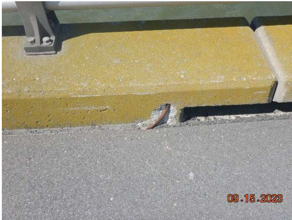
Photo 16: ASB102 Concrete Curb – Random Exposed Rebar in West Curb
