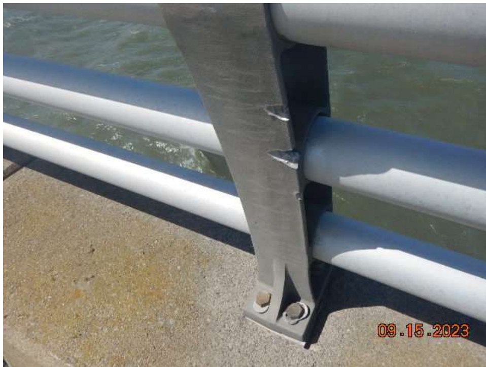
Photo 15: ASB111 Metal Bridge Railing – Minor Vehicle Impact Damage
