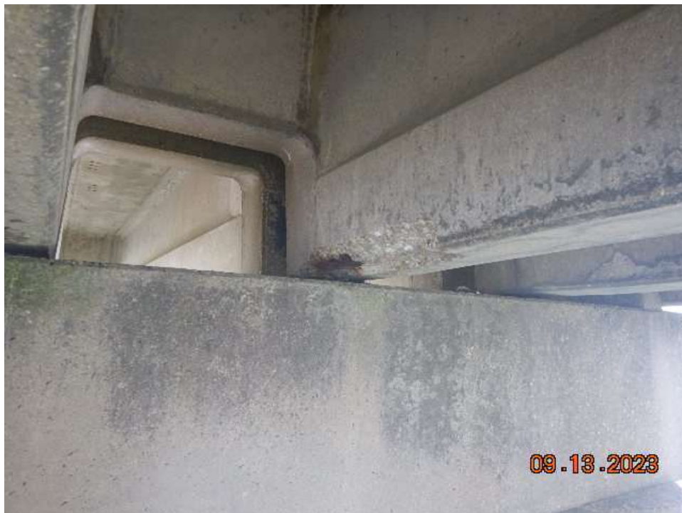
Photo 43: CNB196 Prestressed Concrete Girder – Girder 3 Spall with Exposed Strand at Bent 197
