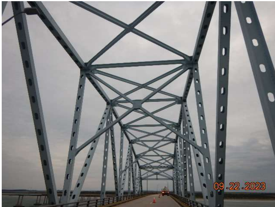
Photo 71: NCB-NB9 Steel Truss – Typical View and Condition of Upper Chord, Verticals and Diagonals
