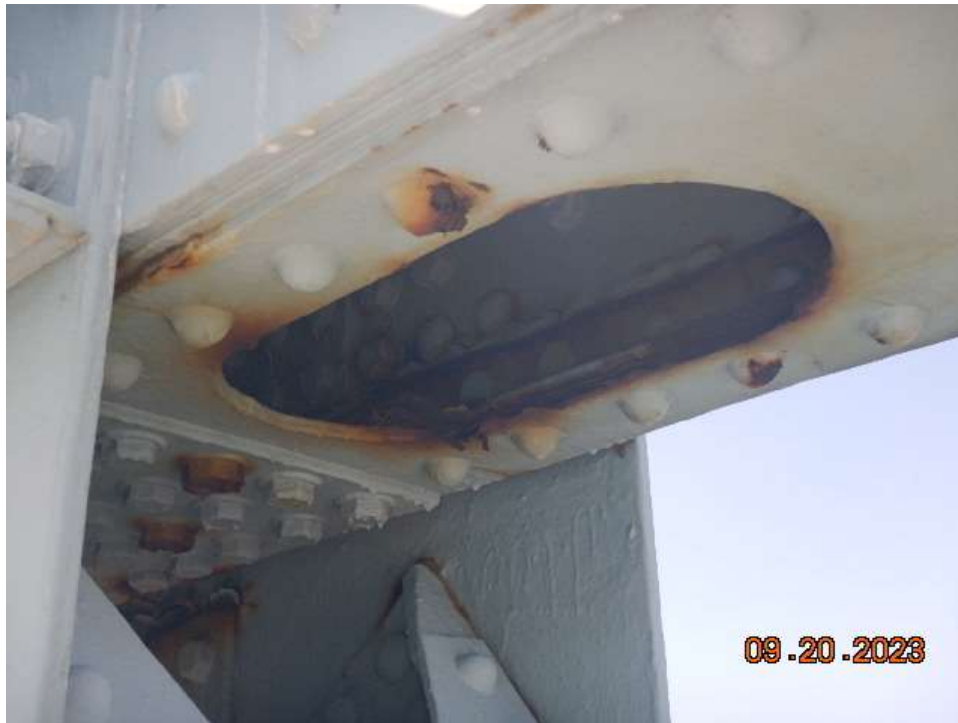
Photo 73: NCB-NB9 Steel Truss – Corrosion with Minor Section Loss at Handhole in the Upper Chord at U5, West Truss
