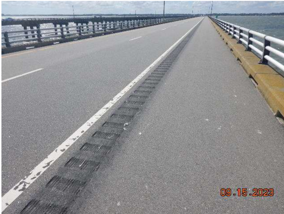
Photo 10: ASB119 Asphalt Wearing Surface – Typical Good Condition of Wearing Surface (Looking South)
