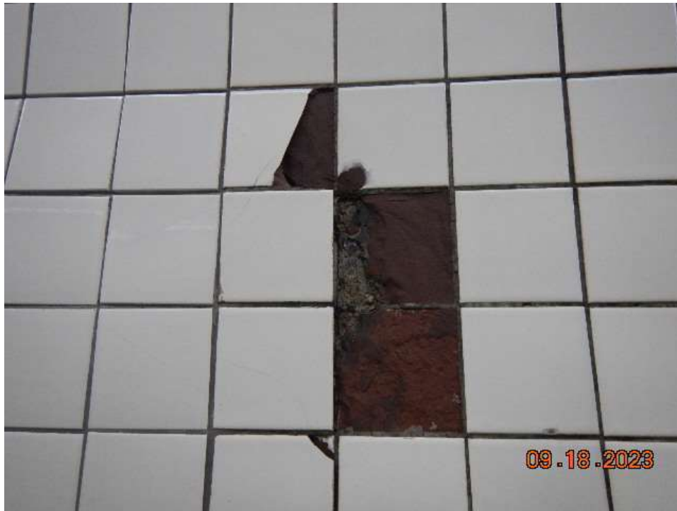
Photo 84: Sta. 194+05 – Broken and Missing Tiles on West Wall Adjacent to Safety Walkway
