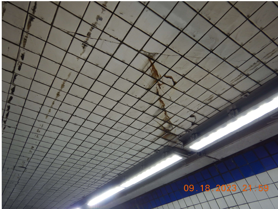
Photo 86: Sta. 195+65 – Cracked Ceiling Tiles with Rust Stains over NB Lane
