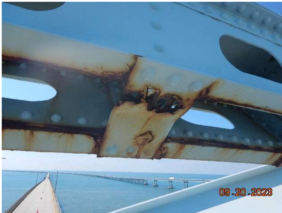
Photo 72: NCB-NB9 Steel Truss – Corrosion with 100% Section Loss of Batten Plates at South Portal Bracing
