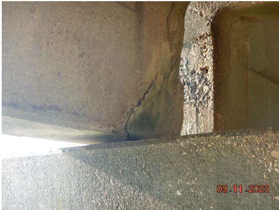
Photo 7: ANB137 Prestressed Concrete Girder – Delamination at End of Girder 1 at Bent 137
