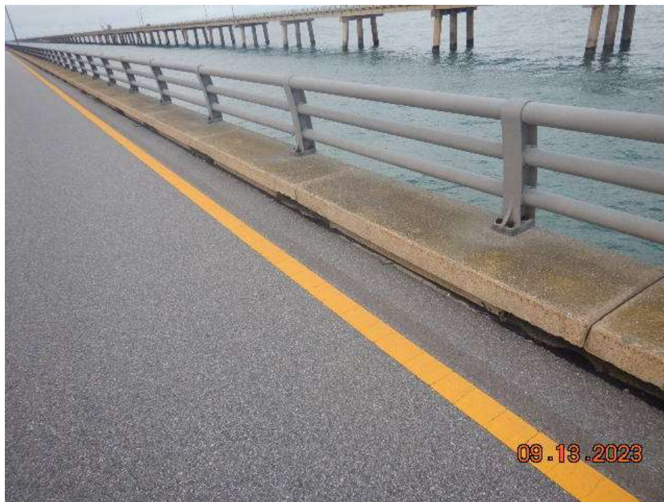
Photo 39: CNB140 – Metal Bridge Railing – Typical Condition of Metal Railing & Curb (Looking Southwest)
