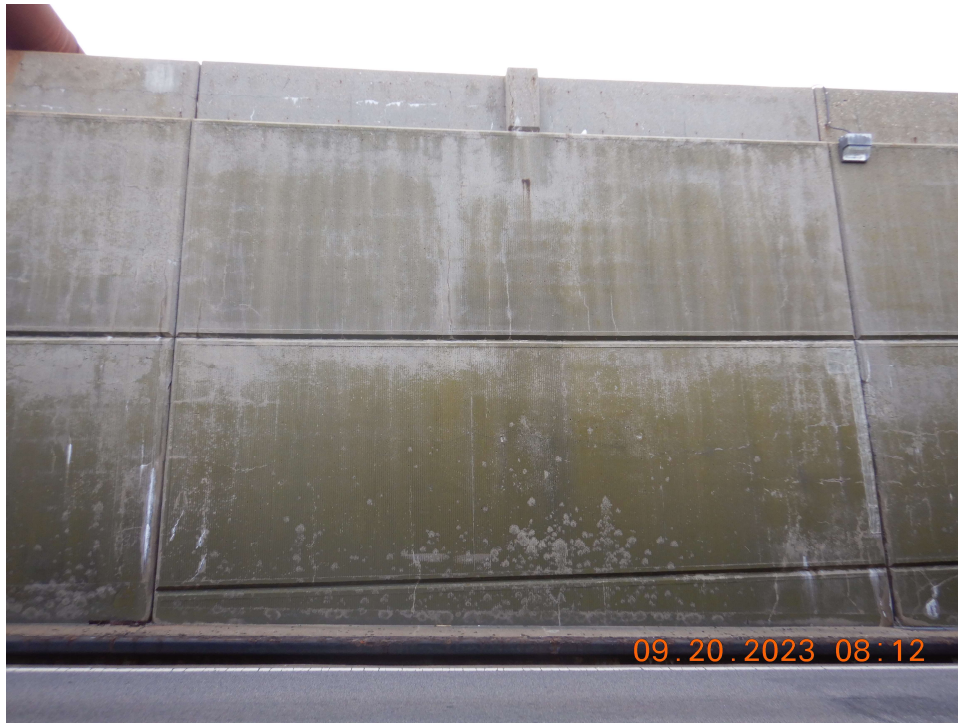
Photo 88: Typical Hairline Cracking with Efflorescence of Open Approach Retaining Walls (Island 2 Approach Shown)
