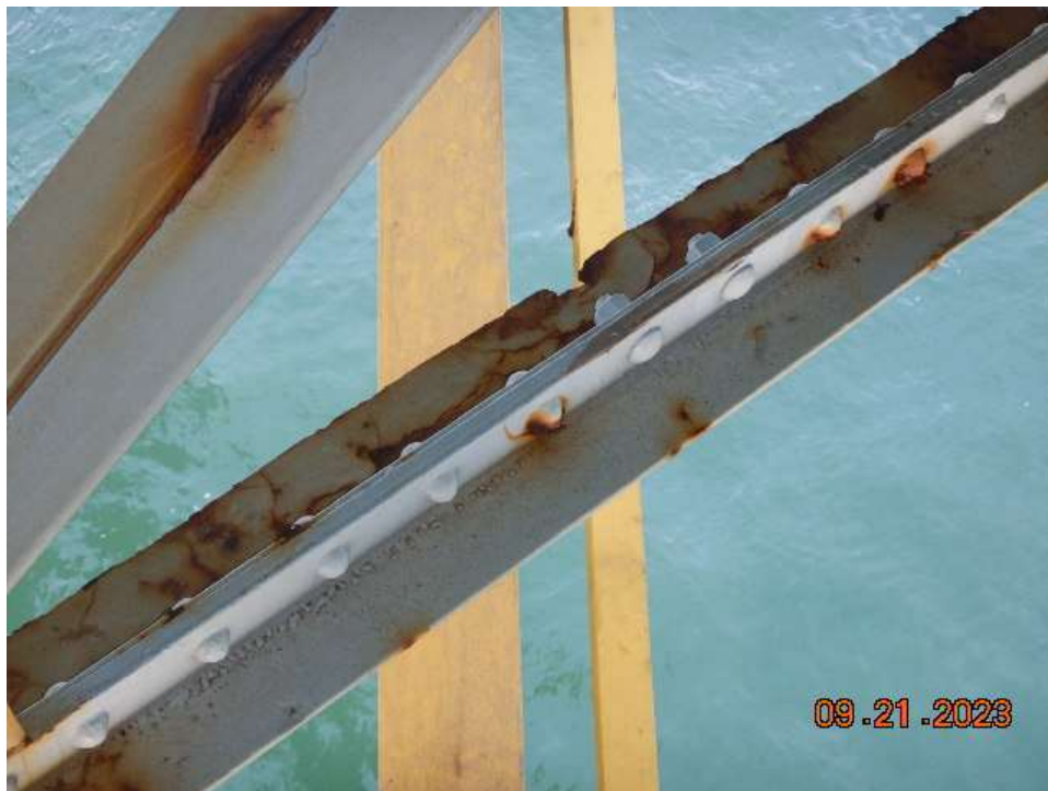
Photo 68: NCB-NB15 – Peeling Paint with up to 100% Section Loss in Cross Bracing at Floorbeam 6
