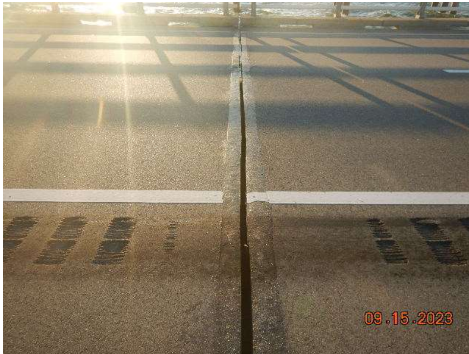
Photo 32: BSB138 Open Joint - Typical Condition of Open Joint
