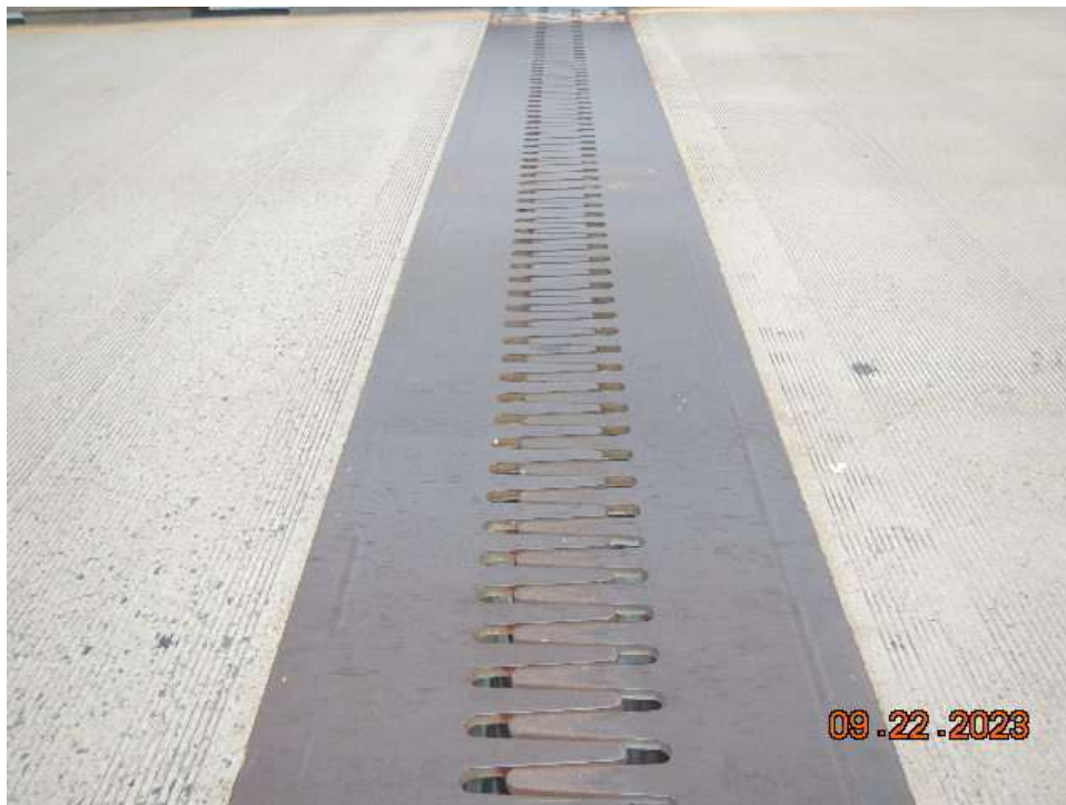
Photo 52: Typical Condition of Finger Joints
