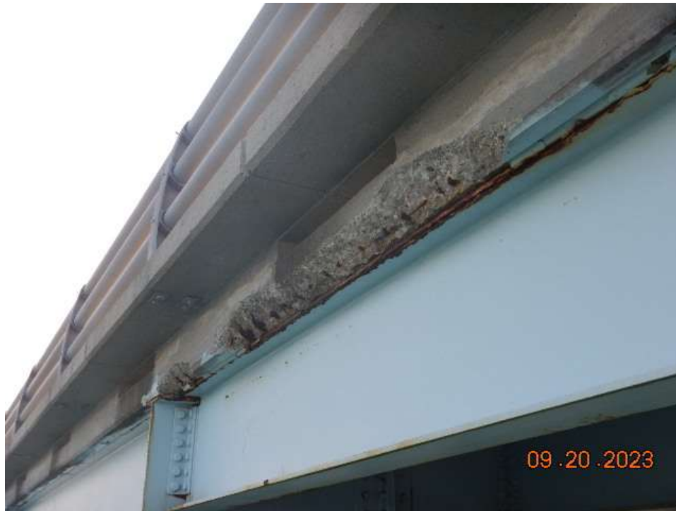
Photo 65: NCB-NB11 Reinforced Concrete Deck – Spall with Exposed Reinforcing in the West Fascia near Floorbeam 9
