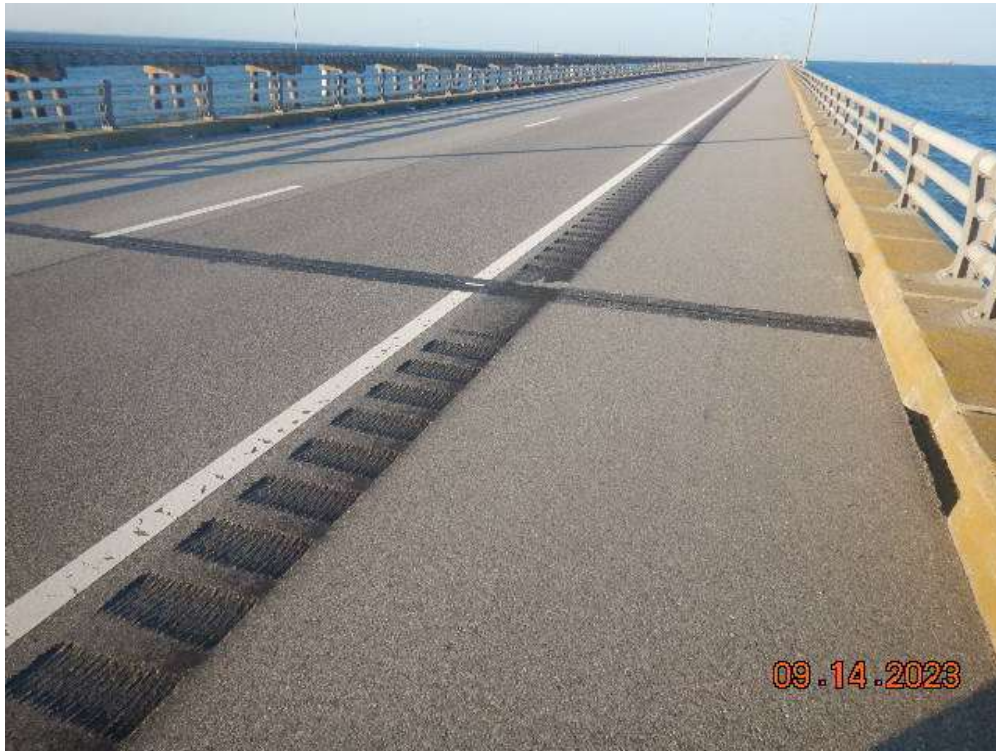
Photo 44: CSB153 Wearing Surface – Typical Good Condition of Deck and Bridge Railing (Looking South)
