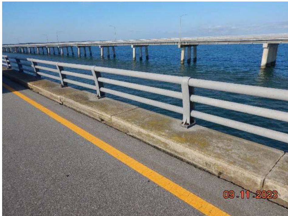
Photo 2: ANB141 Concrete Curb & Metal Bridge Railing – Typical Good Condition of Curb & Railing (Looking Southwest)
