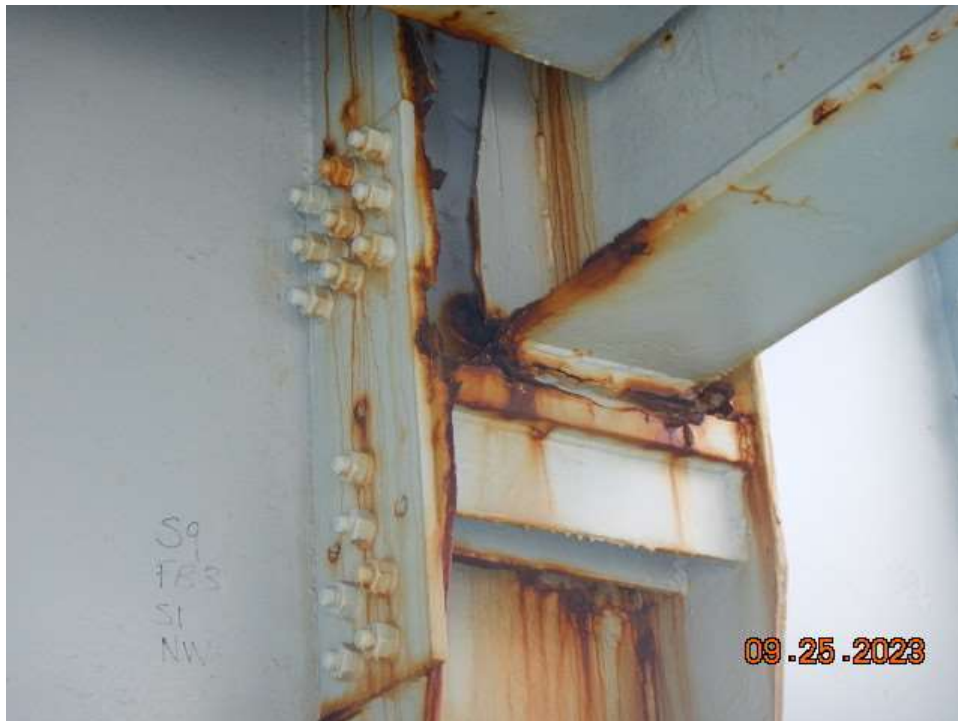
Photo 75: NCB-NB9 Steel Floorbeam – Severe Corrosion with 100% Section Loss in Floorbeam 3 Web under Stringer 1
