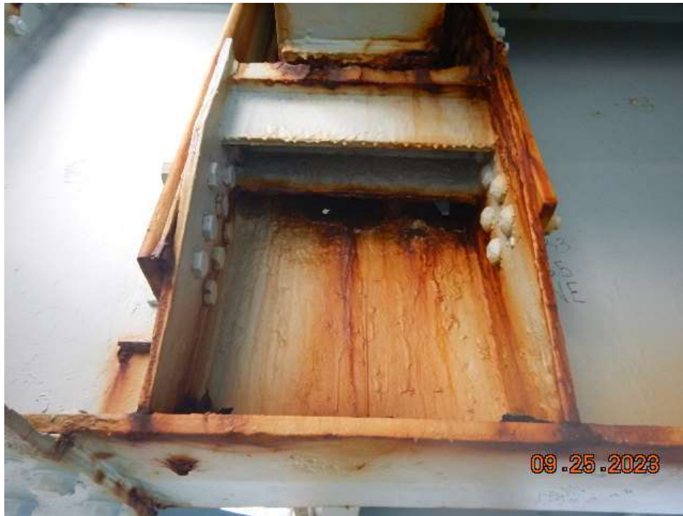
Photo 74: NCB-NB9 Steel Floorbeam – 100% Section Loss in Floorbeam 3 Web at the Northeast Corner below Stringer 5
