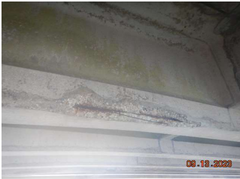
Photo 41: CNB136 Prestressed Concrete Girder – Girder 4 Spall with Exposed & Corroded Strand
