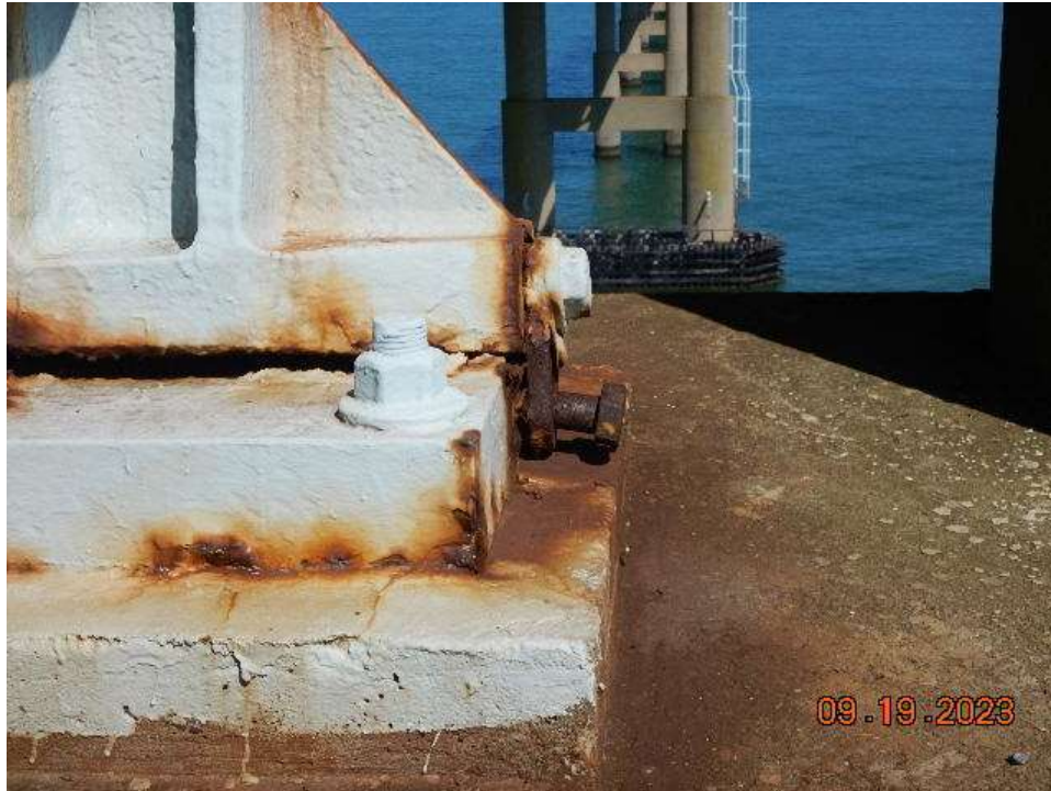
Photo 63: NCB-NB9 – Bearings – Loose Keeper Bolt at Bearing 1
