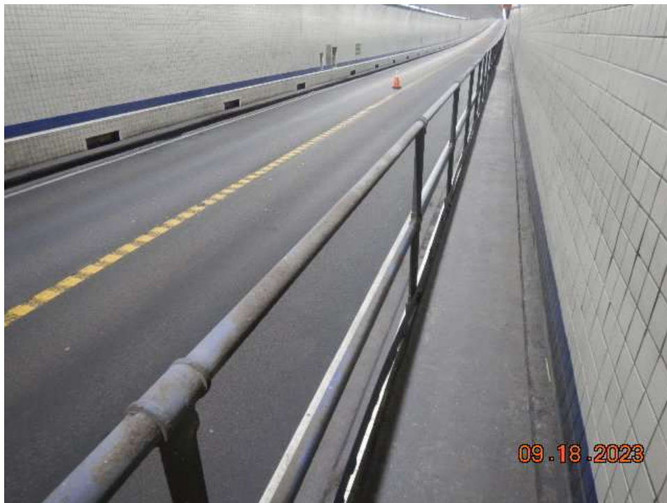
Photo 83: Typical Condition of Metal Handrail with Corrosion
