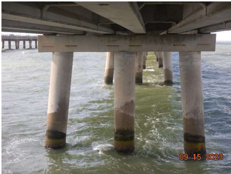
Photo 35: BSB113 Reinforced Concrete Pier Cap – Exposed Reinforcing due to Insufficient Cover
