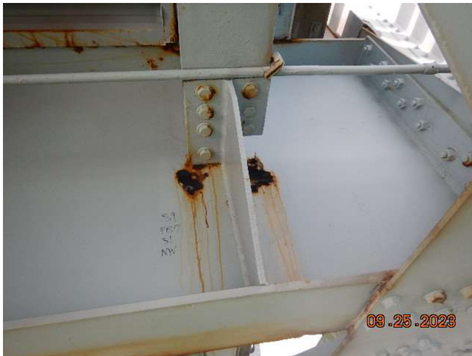
Photo 77: NCB-NB9 Steel Floorbeam – Severe Corrosion with 100% Section Loss in Floorbeam 3' Web at Stringer 1
