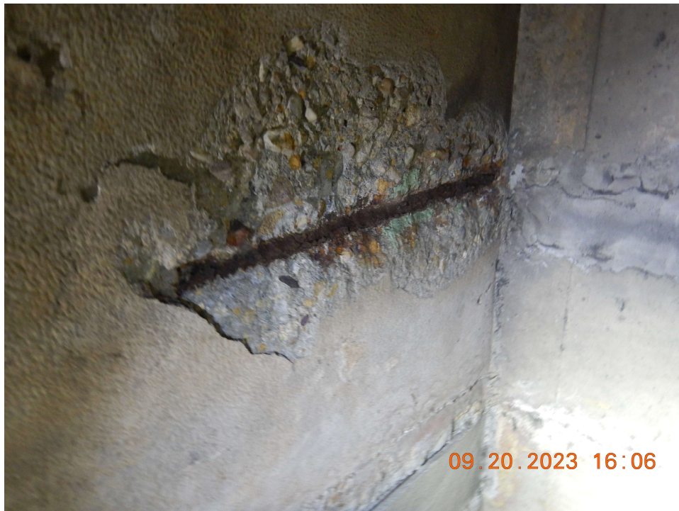
Photo 89: Supply Duct – Sta. 191+10 Spall with Exposed Reinforcement in Underside of Invert Slab
