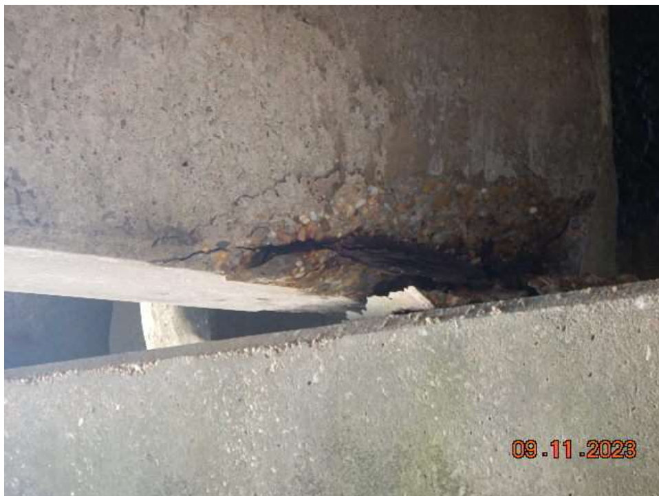
Photo 6: ANB133 – Prestressed Concrete Girder – 2' Long Spall with Exposed & Corroded Strand in Girder 3 at Bent 133
