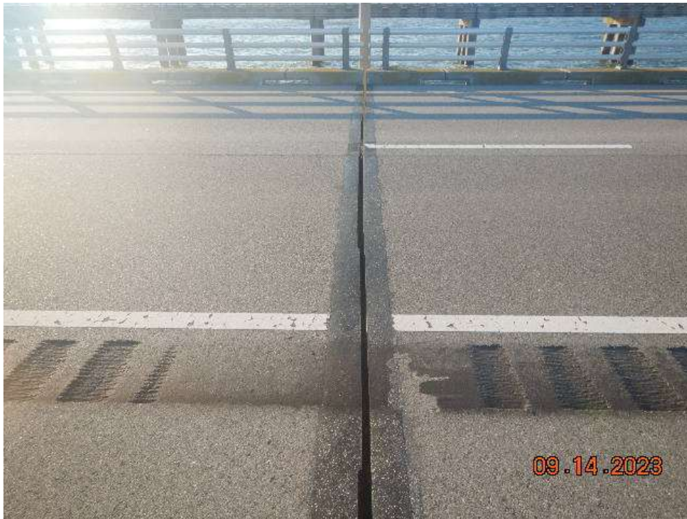
Photo 46: CSB153 Open Expansion Joint – Typical Good Condition of Open Expansion Joints (Looking East)
