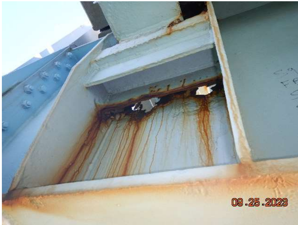
Photo 76: NCB-NB9 Steel Floorbeam – Severe Corrosion with 100% Section Loss in Floorbeam 3' Web
