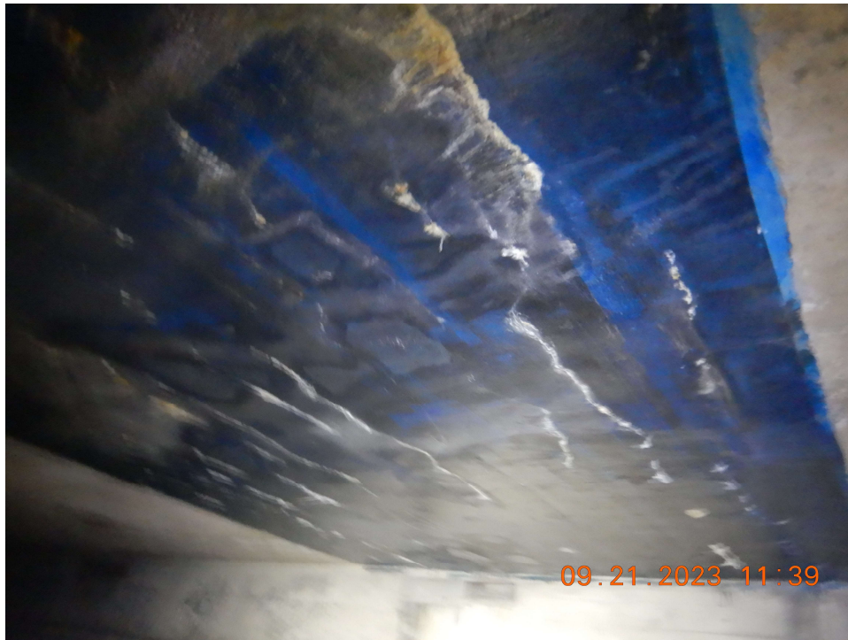
Photo 90: Supply Duct – Sta. 194+50 Patch in Underside of Slab with Carbon Fiber Wrap
