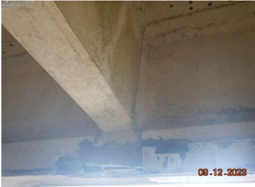
Photo 23: BNB124 Prestressed Concrete Girder – Failed Patch in Girder 2 with Formwork in Place
