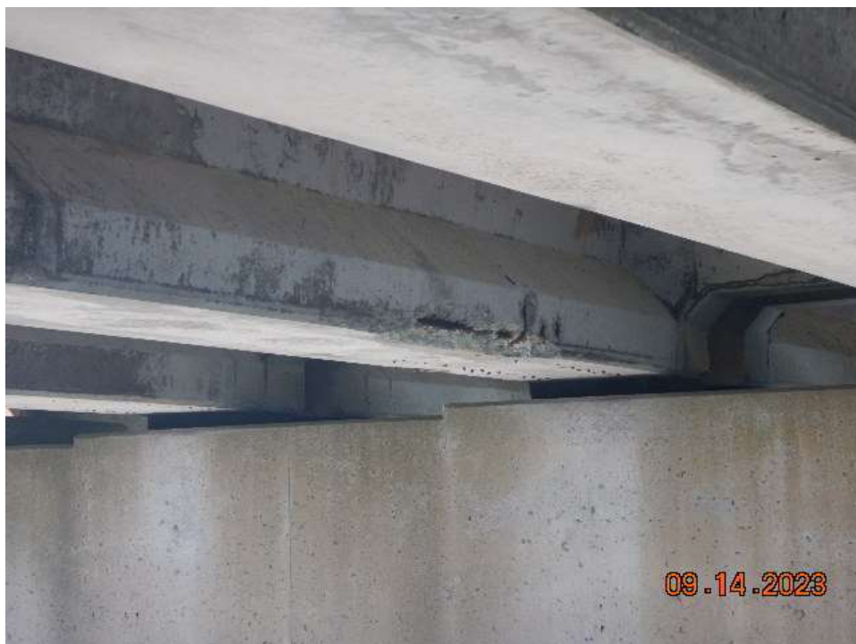
Photo 49: CSB100 – Prestressed Concrete Girder – Girder 4, Spall with Exposed Reinforcing
