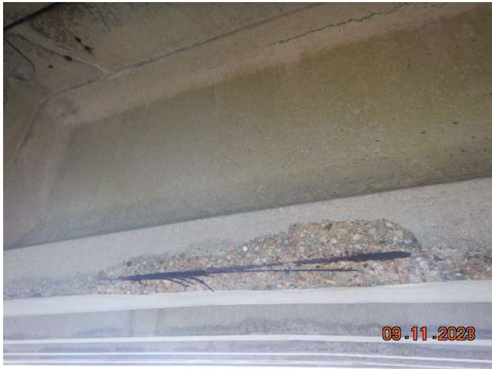
Photo 9: ANB159 – Prestressed Concrete Girder – 2' Long Spall with Exposed Strand in Girder 4
