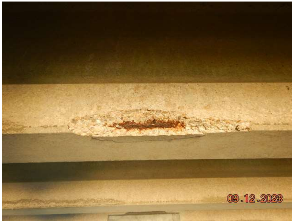
Photo 24: BNB108 Prestressed Concrete Girder – Spall with Exposed Strand in Girder 6
