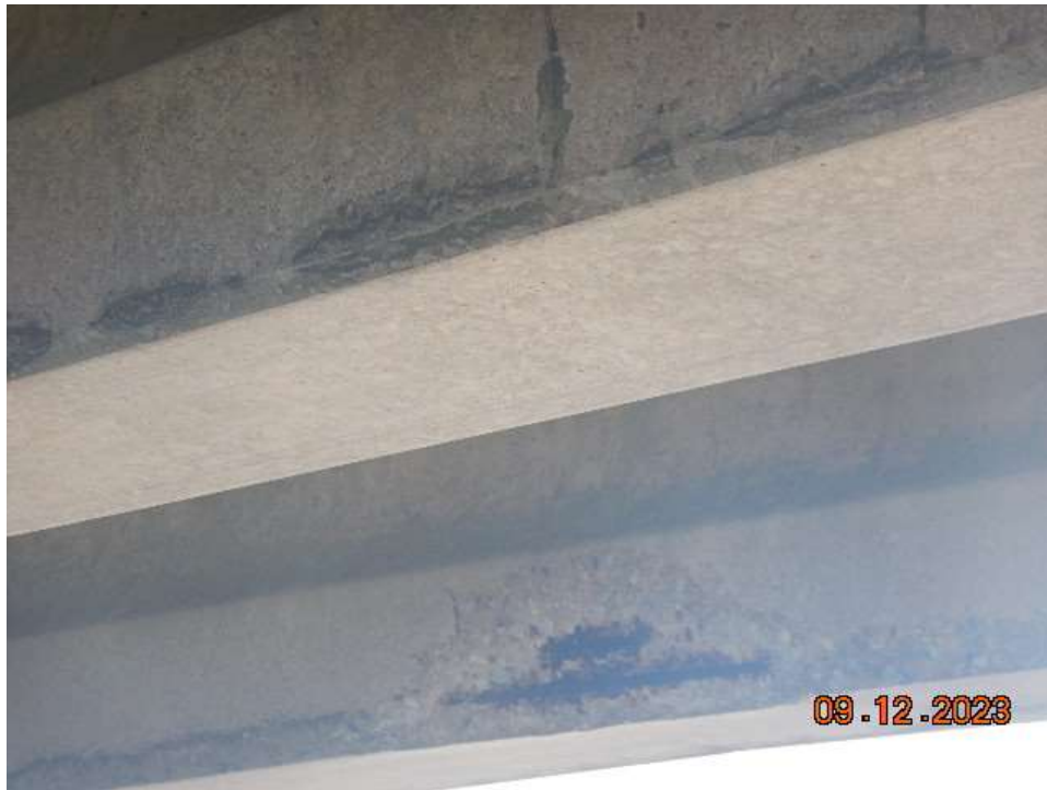
Photo 27: BNB121 Prestressed Concrete Girder – Girder 8 Spalling with Exposed Strands
