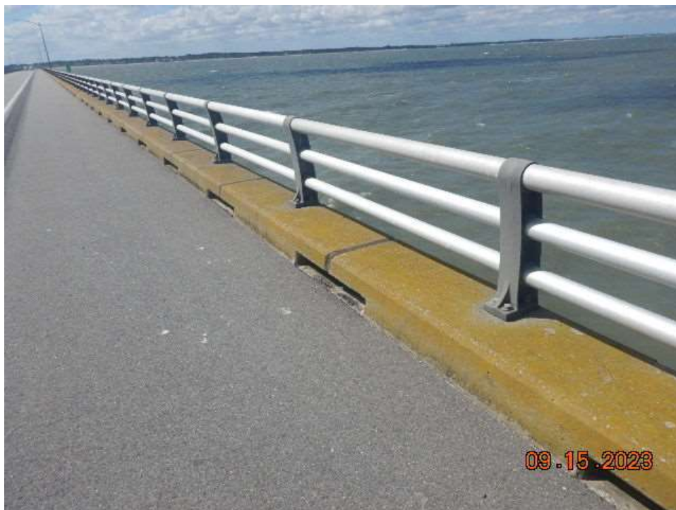
Photo 11: ASB118 Metal Bridge Railing – Typical Good Condition of Bridge Railing and Curb (Looking Southwest)
