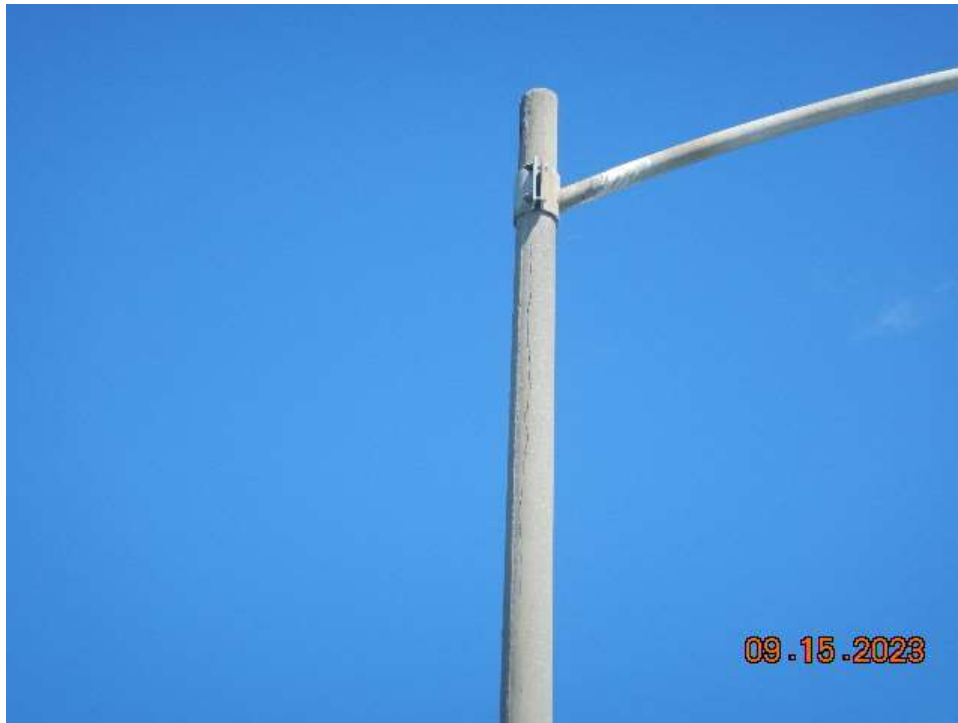
Photo 18: ASB115 – Vertical Crack in Light Pole at Bent 115
