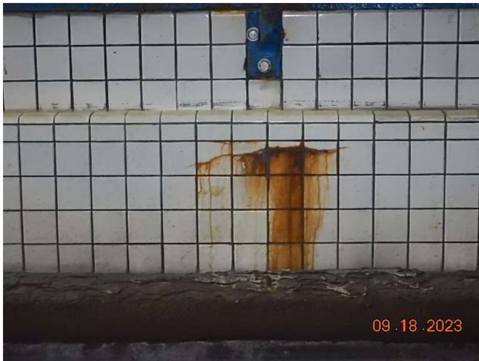
Photo 85: Sta. 210+95 – Four Cracked Tiles with Rust Staining Below Safety Walkway
