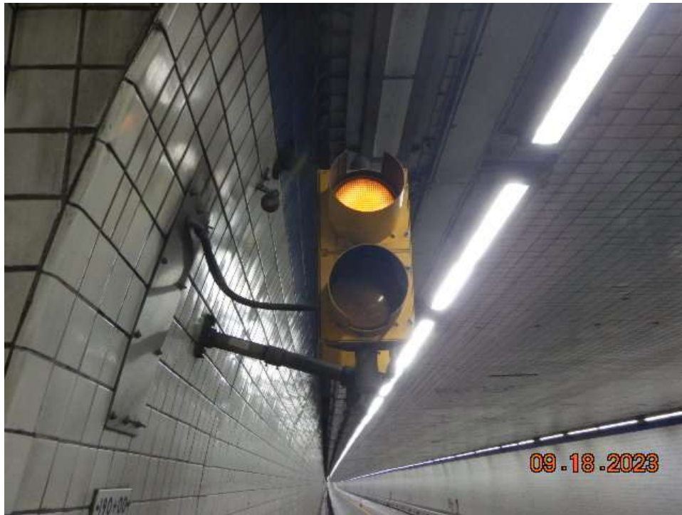
Photo 82: Sta. 190+00 – Non-functioning Signal Light (Bottom Light Never Illuminated)
