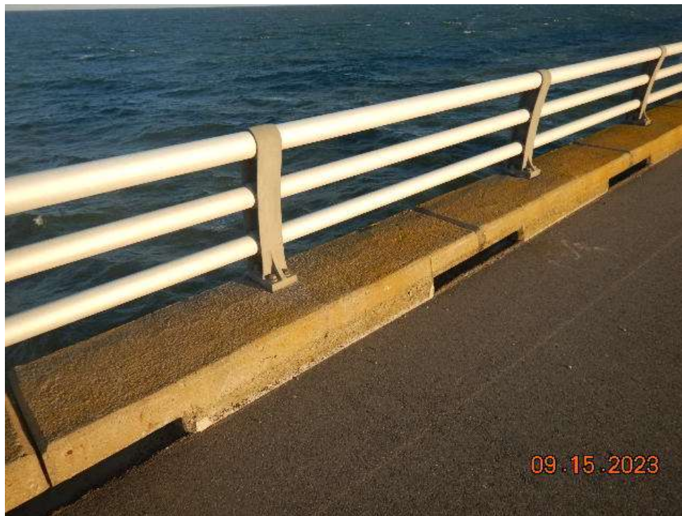
Photo 31: BSB140 Metal Bridge Railing – Typical Good Condition of Bridge Railing & Curb (Looking Northwest)
