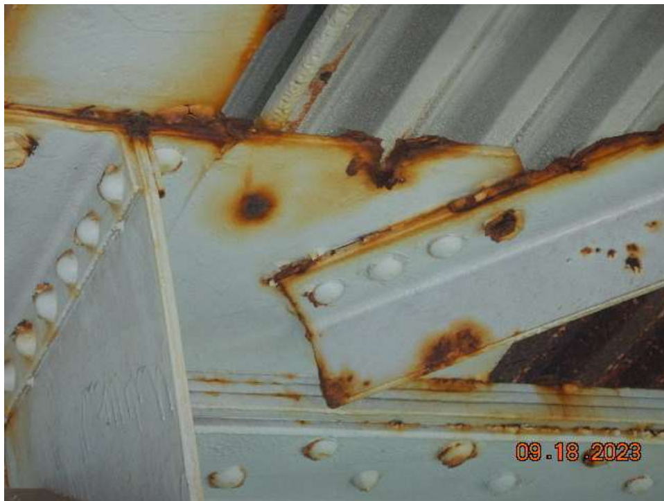
Photo 56: NCB-NB Corrosion with 100% Section Loss in Horizontal Connection Plate
