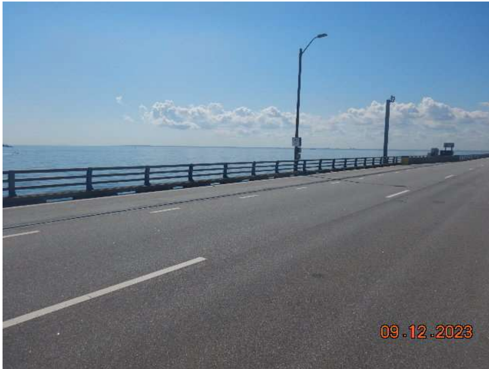
Photo 19: BNB132 - Wearing Surface and Metal Bridge Railing – Typical Good Condition (Looking Southeast)
