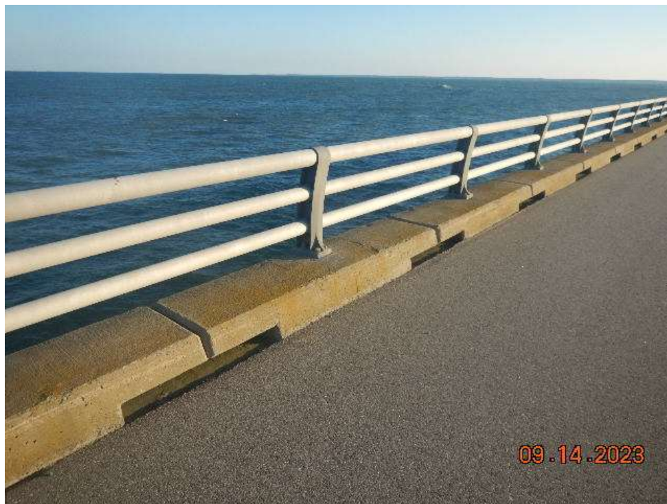
Photo 45: CSB153 Metal Bridge Railing– Typical Good Condition of Bridge Railing (Looking Northwest)
