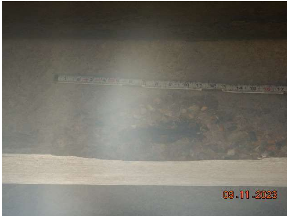
Photo 5: ANB133 Prestressed Concrete Girder – Spall with Exposed Strand in Girder 4 near Midspan
