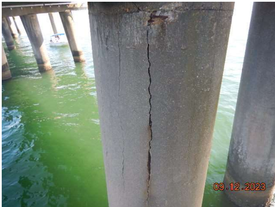
Photo 28: BNB123 Prestressed Concrete Pile – Bent 123, Pile A CS3 Crack in Southwest Face
