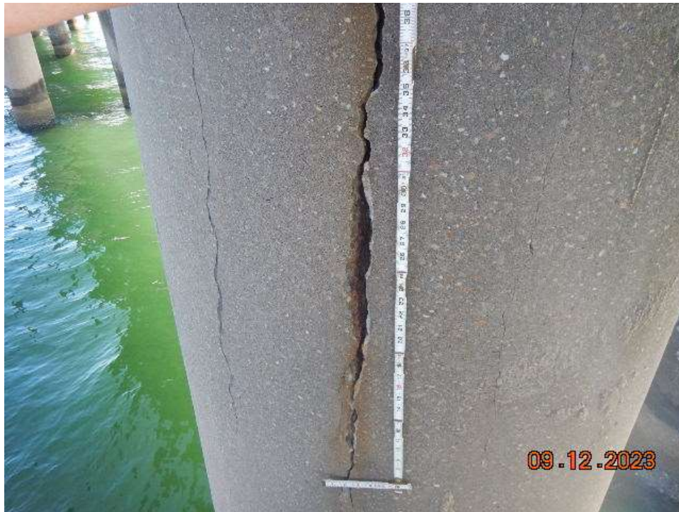
Photo 29: BNB123 Prestressed Concrete Pile – Bent 123, Pile A CS3 Crack in Southwest Face
