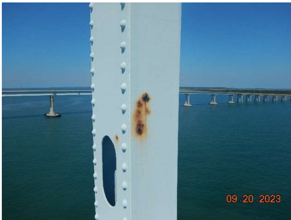
Photo 74: NCB-NB9 Steel Truss – Corrosion Holes in Vertical U4'L4', West Truss
