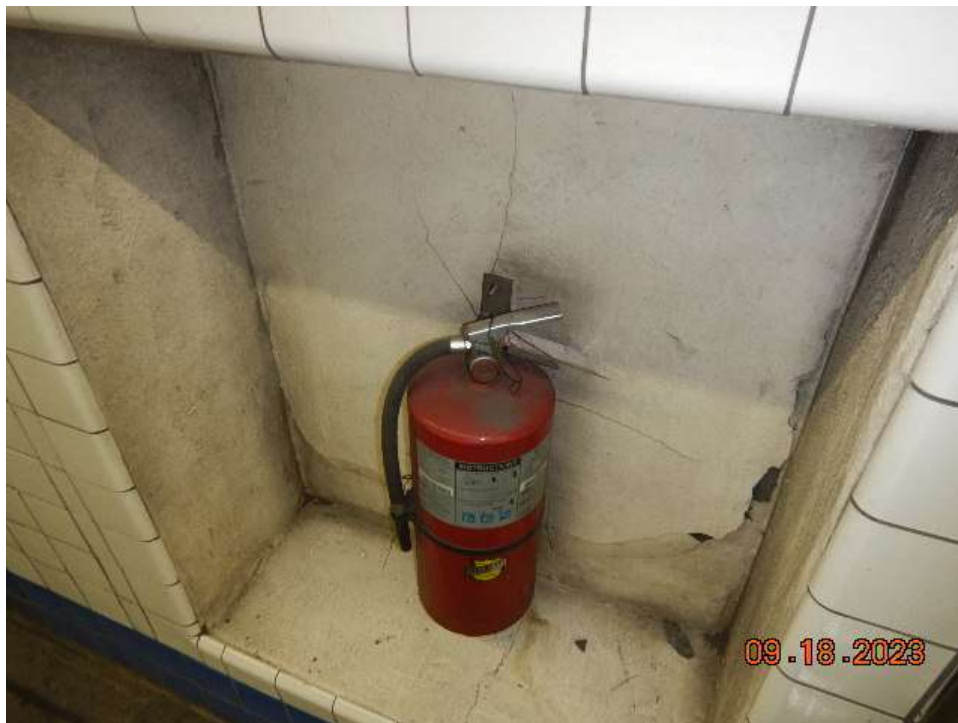
Photo 81: Typical Replaced Fire Extinguisher (100% of Fire Extinguishers replaced since 2021)
