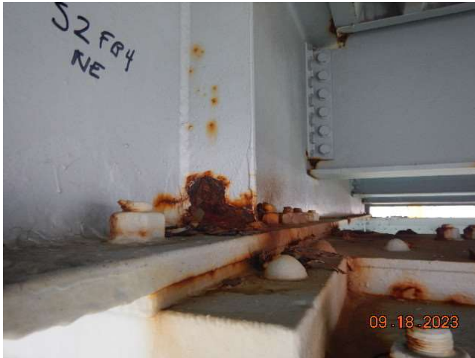
Photo 55: NCB-GB2 Floorbeam – Corrosion Hole in Floorbeam 4, Northeast Stiffener in Span 2
