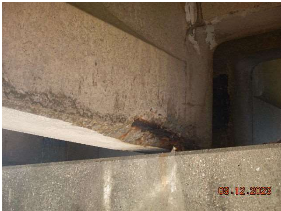
Photo 26: BNB109 Prestressed Concrete Girder – Girder 3 Spall with Exposed Strand at Bent 109
