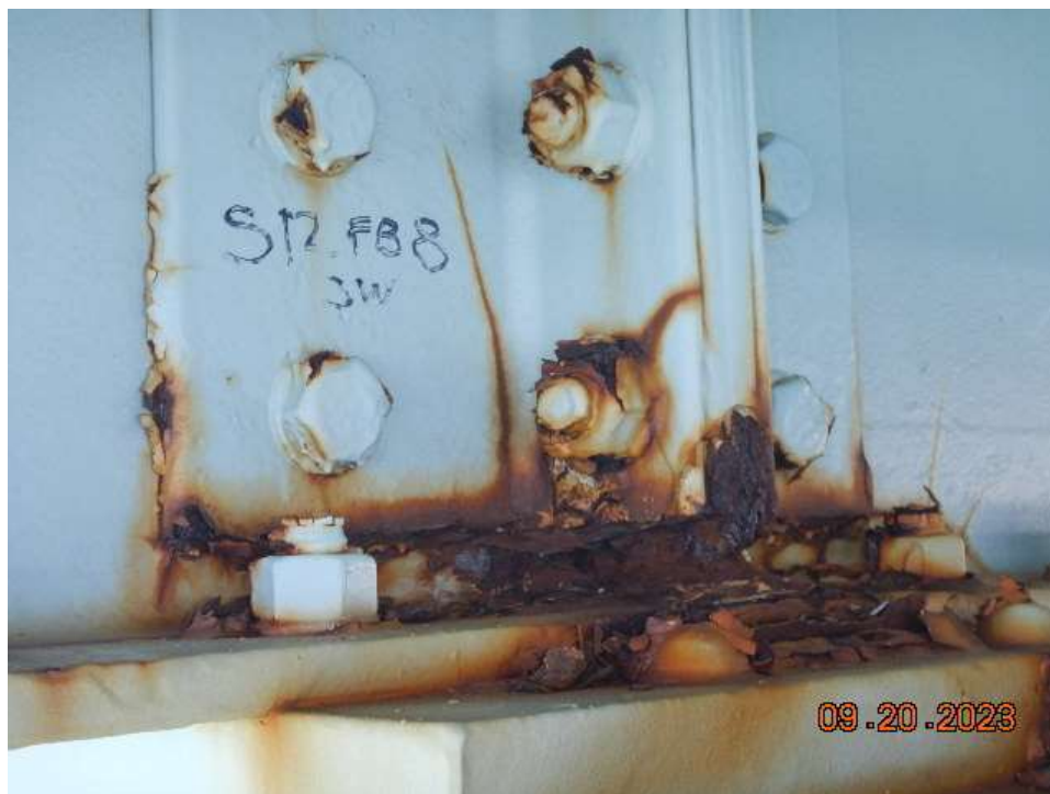
Photo 66: NCB-NB12 Steel Floorbeam – Crack in Connection Plate at the Southwest Stiffener at Floorbeam 8
