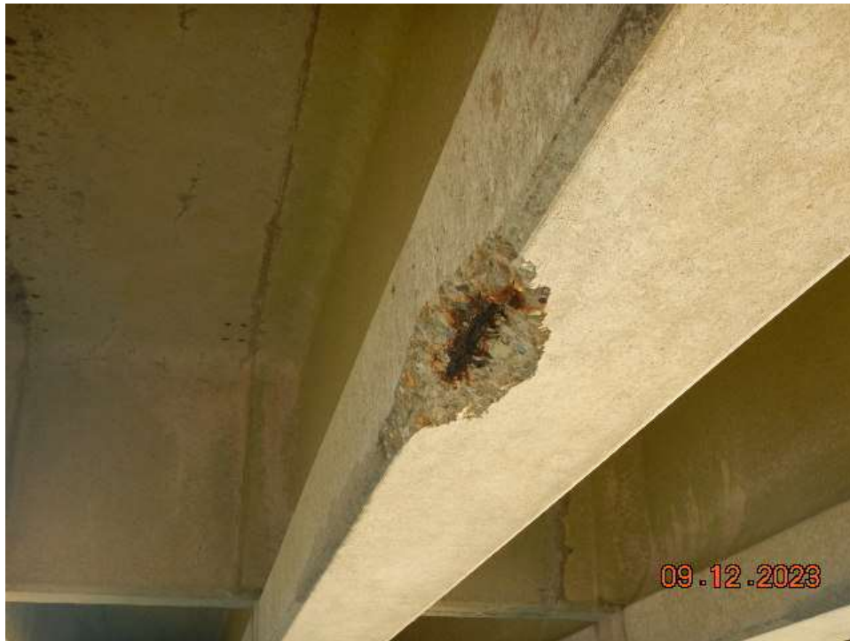
Photo 25: BNB110 Prestressed Concrete Girder – Girder 7 Spall with Exposed Strand
