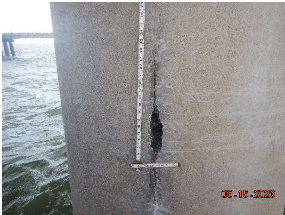
Photo 37: BSB108 Prestressed Concrete Pile – Spall in Pile A in West Face (Looking East)
