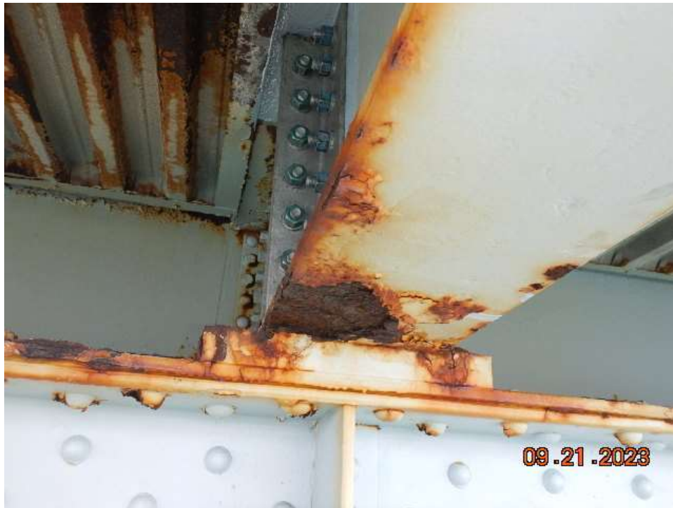
Photo 69: NCB-NB17 Steel Floorbeam – Corrosion with Section Loss on Bottom Flange of Floorbeam 8, West Cantilever
